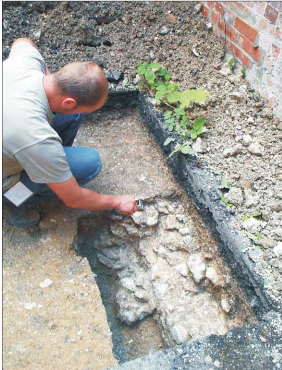
Plate 1: Trench 2 - Medieval wall 204 as exposed in base of robber cut, looking west
