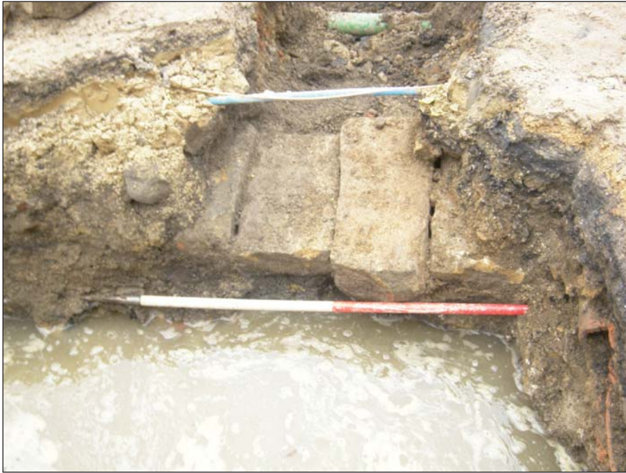
Plate 15: Detail of east-west aligned stone culvert 1014 at corner of Trench as it turns to run parallel with the Conservative Wall glasshouse
