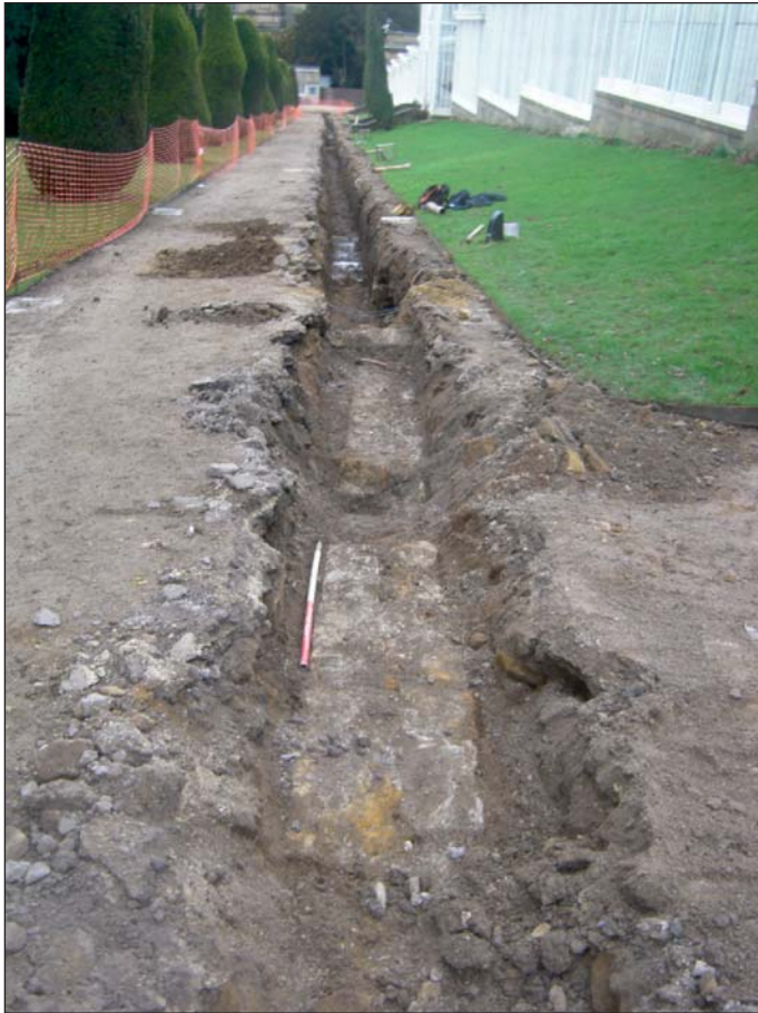
Plate 3: View of Trench, looking west along path beside the Conservative Wall greenhouse, noting wall 1042
