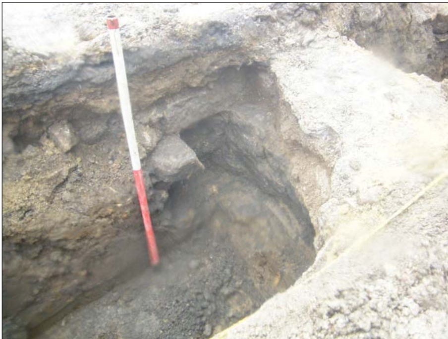
Plate 16: Detail of north-south aligned stone culvert 1015 , at western end of Trench parallel with the Conservative Wall glasshouse
