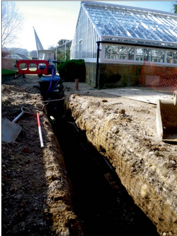
Plate 5: View of Trench, looking west beside the main glass house and vinery
