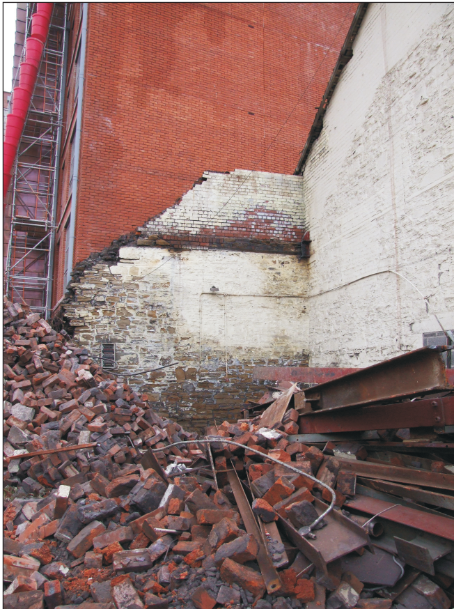
Plate 29: General view the south corner of G12 during demolition, showing the change in fabric from stone to brick after the removal of the traveling crane (Film D.112)
