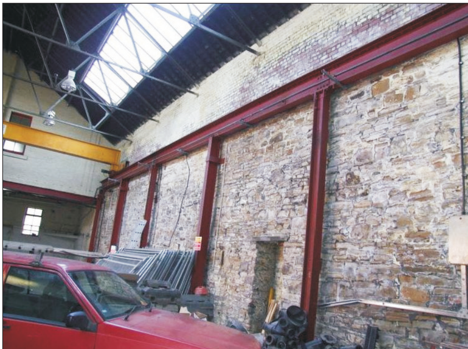
Plate 28: General view of the southeast wall of G12, showing blocked doorway (Film D.41)
