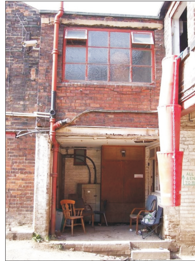
Plate 58: General view of the southeast elevation of the Northwest Range - northeast end, showing G9 (Film D.92)
