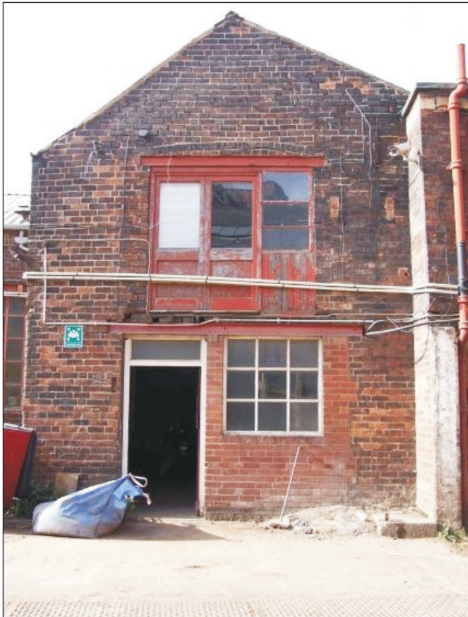
Plate 57: General view the southeast elevation of the Northwest Range - northeast end (Film D.91)
