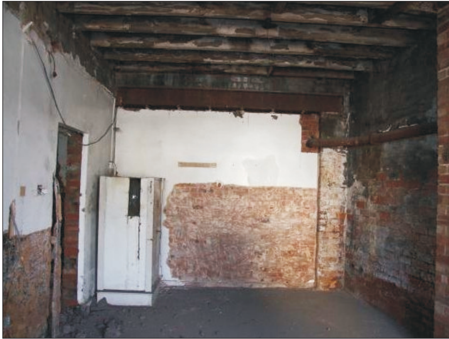
Plate 11: General view of G1, showing former opening within the southwest wall (Film D.18)
