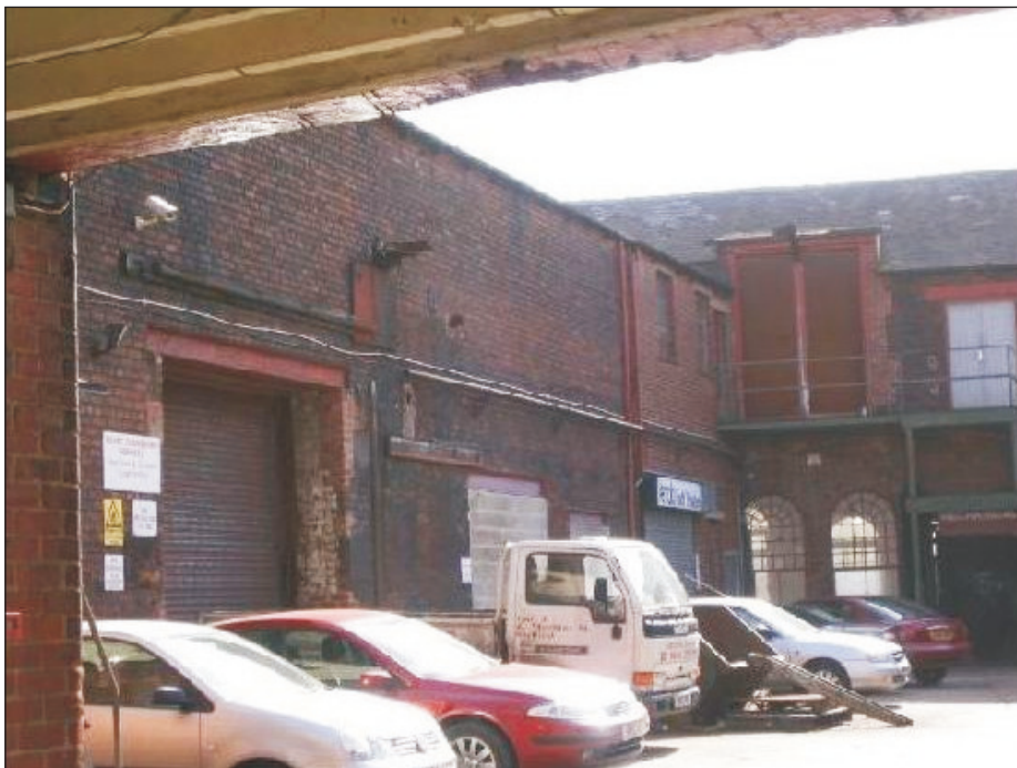
Plate 22: General view of the northwest elevation of the Southeast Range, from the cart passage (Film D.32)
