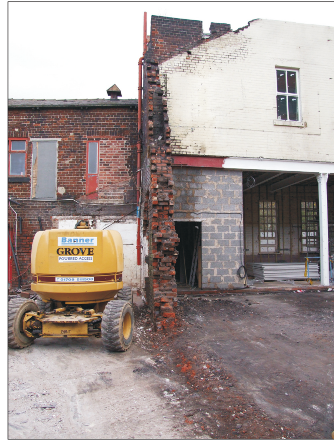
Plate 32: Detail of the northwest wall of the Southeast Range, showing a flue, plus two truncated chimneys in the southwest gable of the Northeast Range (Film D.123)
