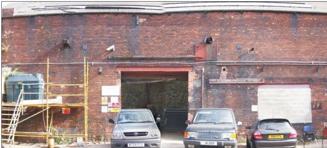
Plate 24: General view of the northwest elevation of the Southeast Range, showing loading door, and two large truncated timber beams (Film D.34)
