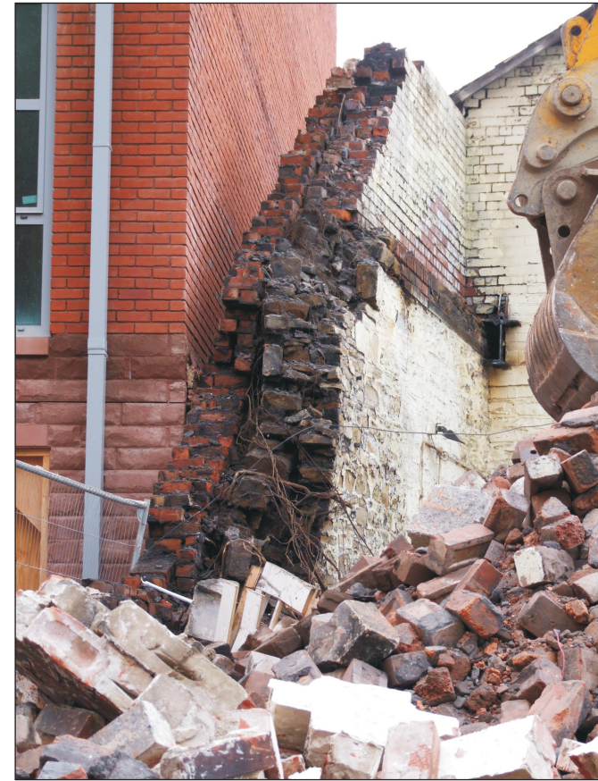
Plate 30: Detail of the southeast wall of the Southeast Range, during demolition, showing the phase 1 stone wall of the Caledonia Works, and the later brick wall of the former adjacent works (Film D.116)
