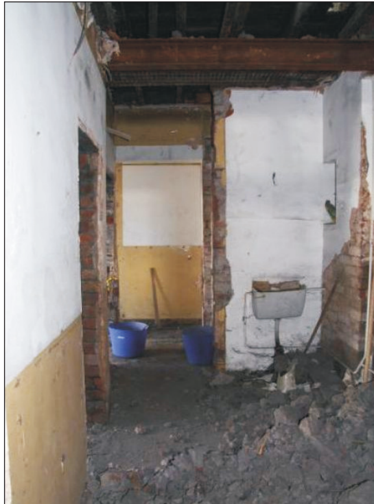
Plate 9: General view of G2a, showing former corridor & W.C partition locations (Film D.17)
