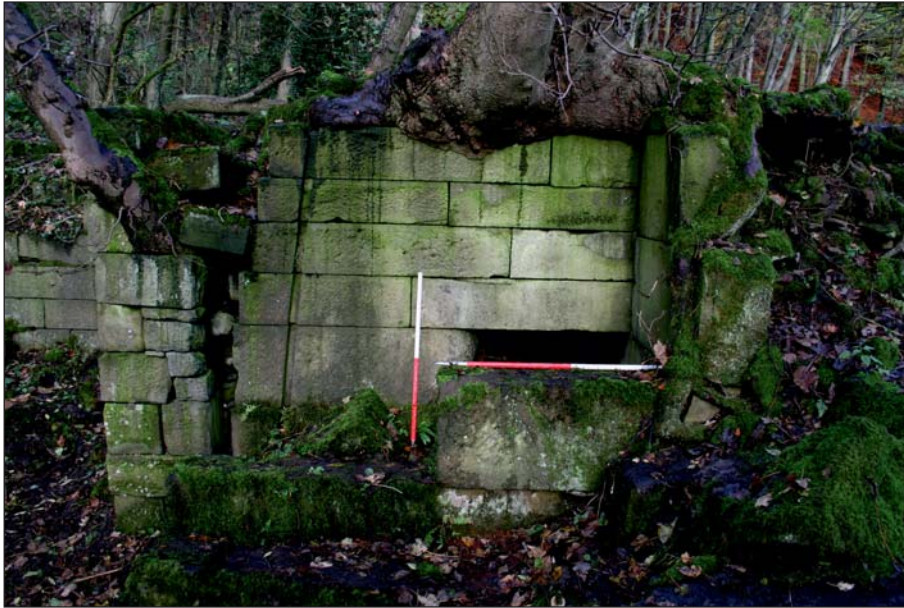
Plate 7: South elevation of 108 , showing inlet, channel for shuttle and damage caused by vegetation
