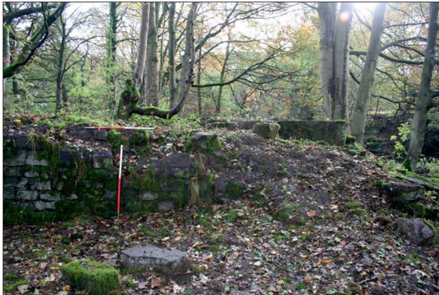
Plate 15: Example of collapse of retaining wall 110
