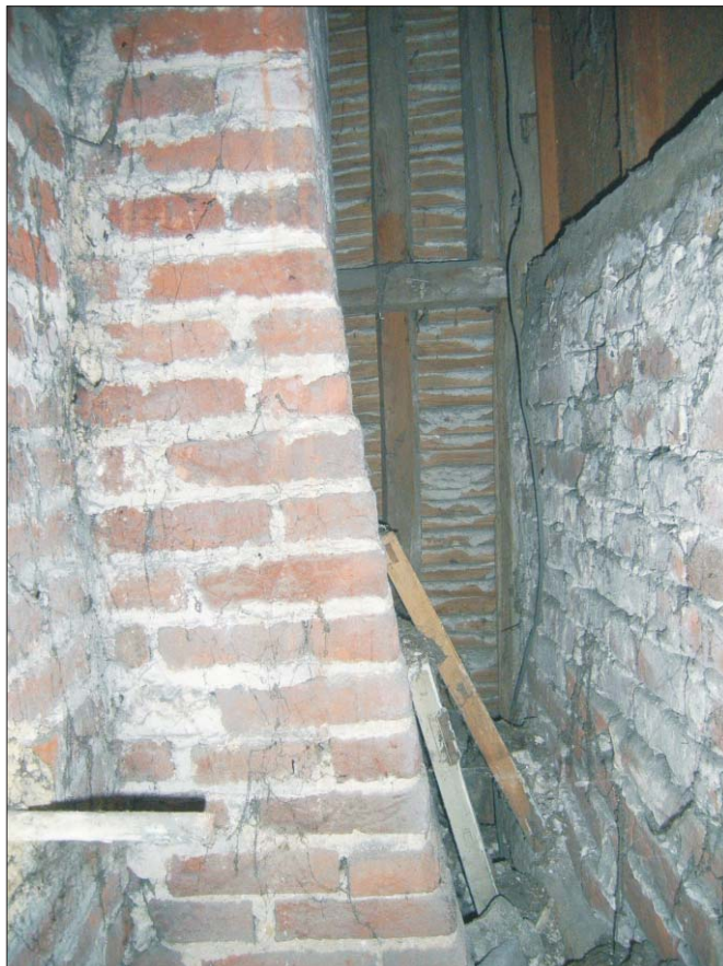
Plate 26 : Attic floor - Exposed stack and framing detail within roof-space above front range
