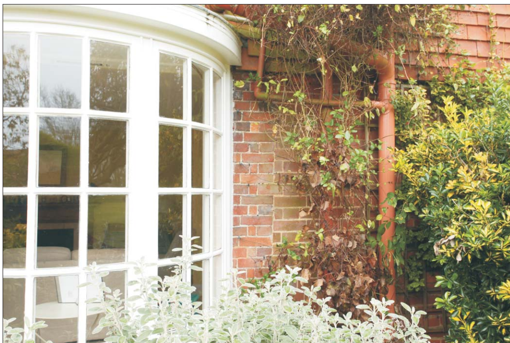
Plate 4 : West elevation - straight joint visible in the brickwork
