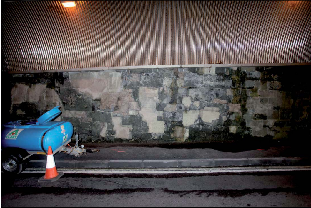
Plate 27: Example of deteriorating tunnel wall fabric showing many repairs viewed from west
