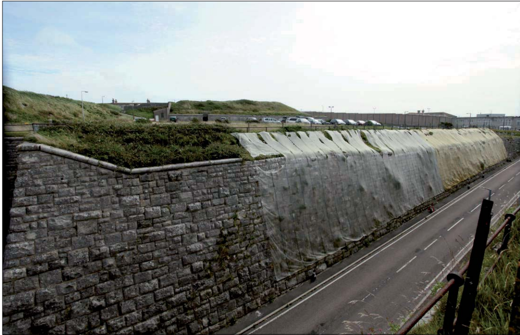
Plate 15: East revetting wall viewed from north-west showing surviving bull-nosed coping stones to main wall
