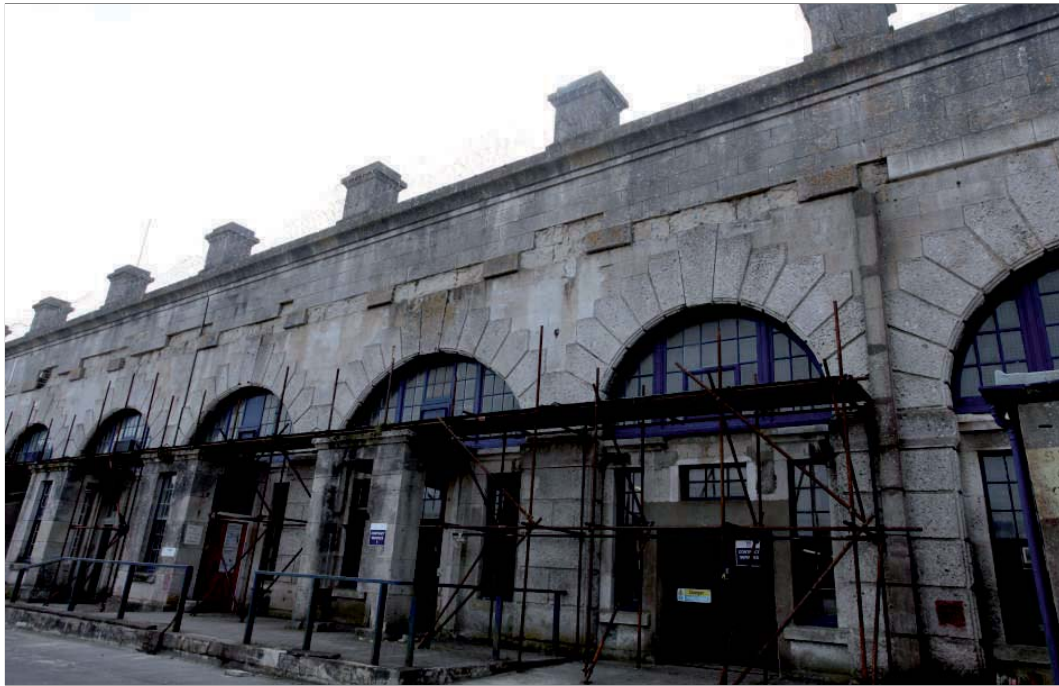
Plate 31: South casemates string course showing earlier concrete repair to top right of image
