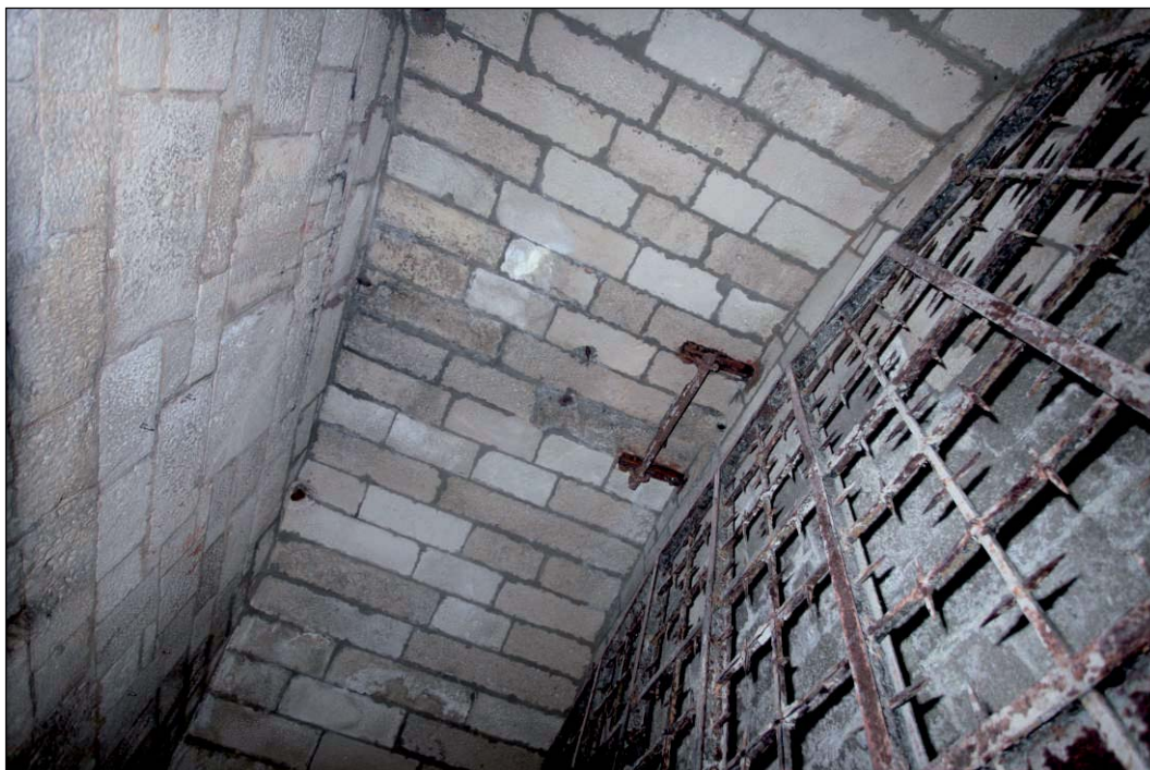
Plate 24: Vaulted ceiling of portcullis chamber showing remains of iron fixings for raising the portcullis
