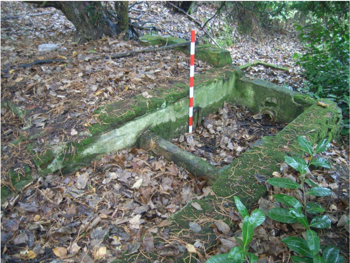
Plate 11 Pond overflow tank viewed from the east
