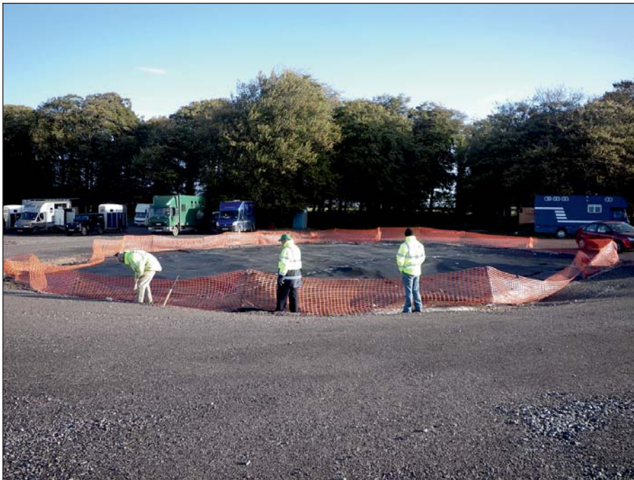
Plate 4: View of the Site from the south showing the protective fencing and geo-textile covering
