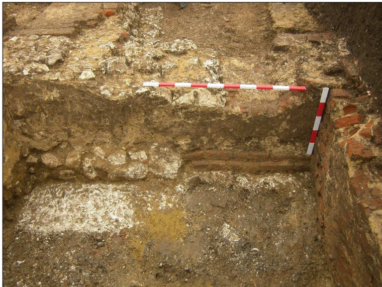
Plate 6: North facing elevation showing blocking wall 210 within the archway in wall 208 of cellar of Great Hall (scales 1m and 0.5m)
