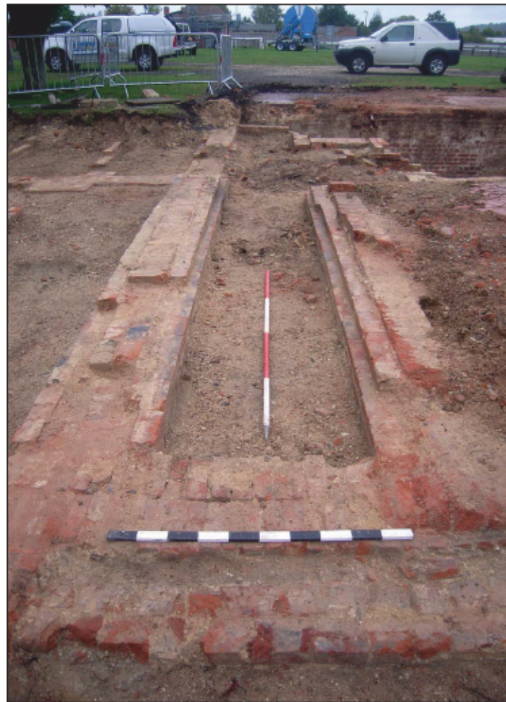
Plate 10: Corridor (Room 5) leading to the cellar (Room 1) and rear entrance, viewed from the south
