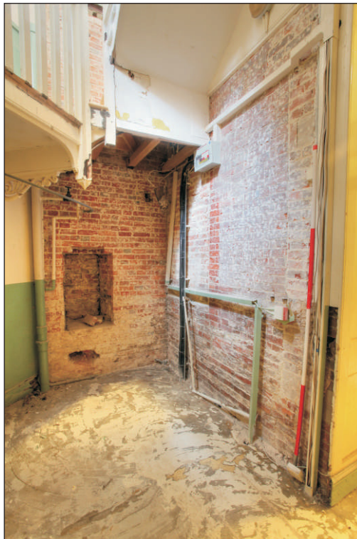
Plate 8: Room RG 07 – North and east walls of the Stairwell exposed following remedial works
