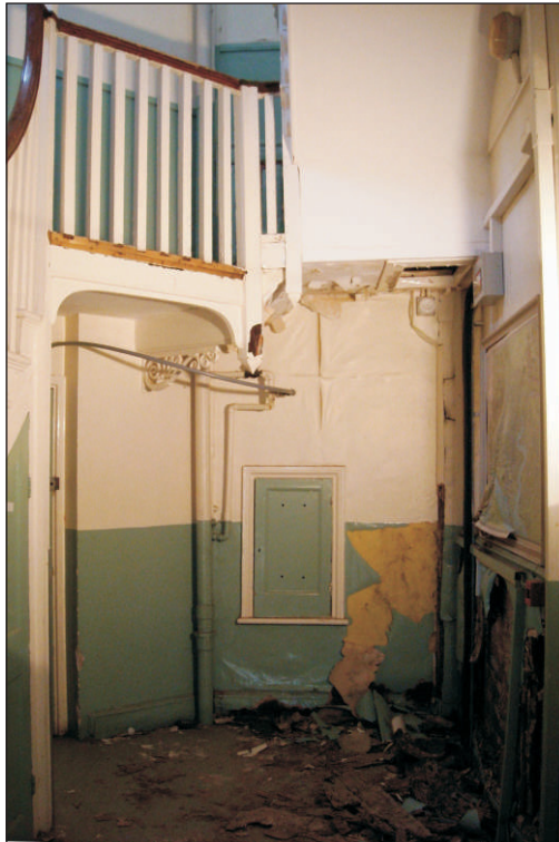
Plate 7: Room RG 07 – North and east walls of the Stairwell prior to remedial works
