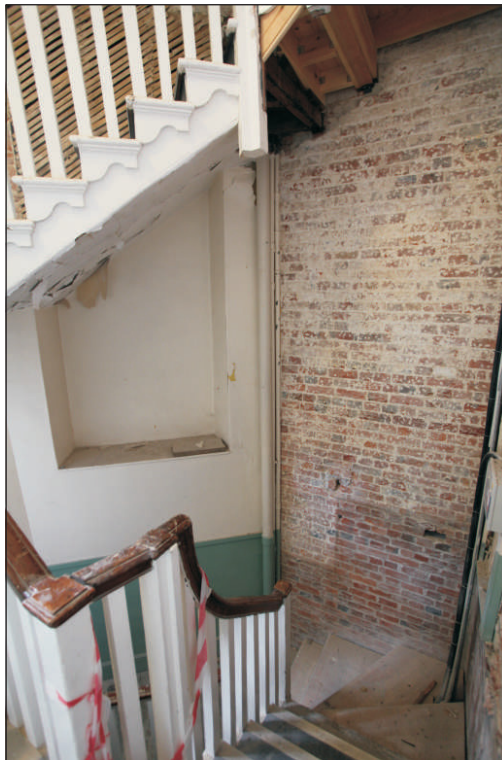
Plate 18: Room 108 – Niche in north-west representing the lower part of a blocked window
