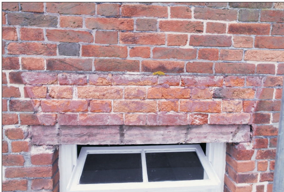
Plate 38: Second floor windows – exposed lintel and brickwork following removal of false cement arch
