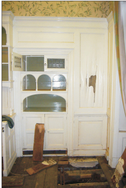
Plate 3: Room RG 04 – fitted cupboard and panelling prior to opening up works – viewed from the west
