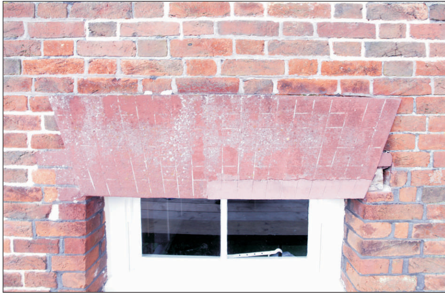
Plate 37: Second floor windows – false cement arch showing later repair
