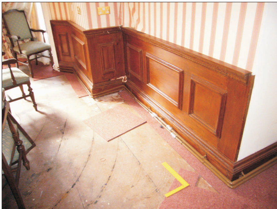
Plate 4: Room RG 03 – Wainscoting and panelling prior to opening up works – viewed from the north-east
