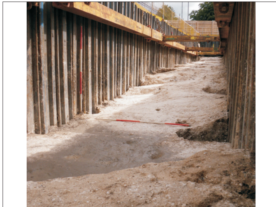
Plate 4: Post-excavation view of Trench 2. Note the drop in the natural chalk geology. View from west (scales: 2 m)
