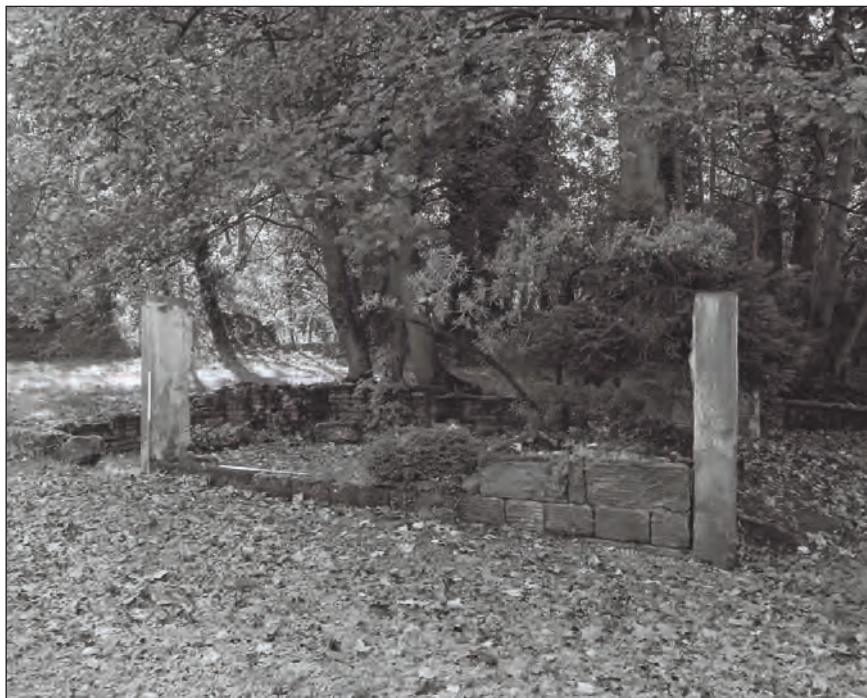
Plate 104: General view of the northern elevation of the eastern phase 3 and 4 ranges (Film 3.8)
