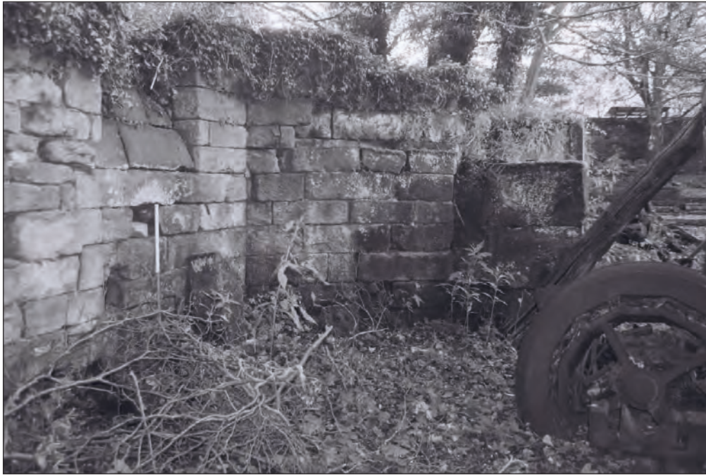
Plate 77: General view of the dam wall behind the east hammer, showing chamfered sill of former window and angled west corner (Film 9.31)
