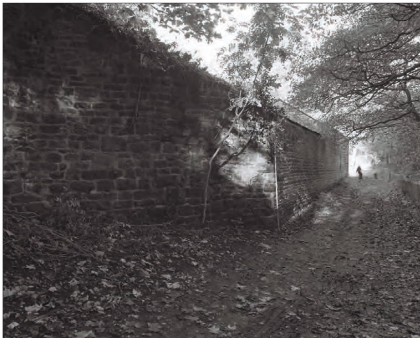
Plate 20: General view of the northeast elevation of the former anvil store and workshop range, showing the angled southeast corner (Film 2.2)
