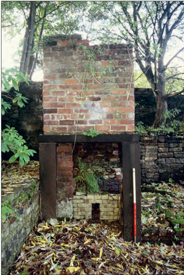
Plate 101: Detail of the chimney remains at the southwest corner of the western phase 3 range (Film CS. 1)
