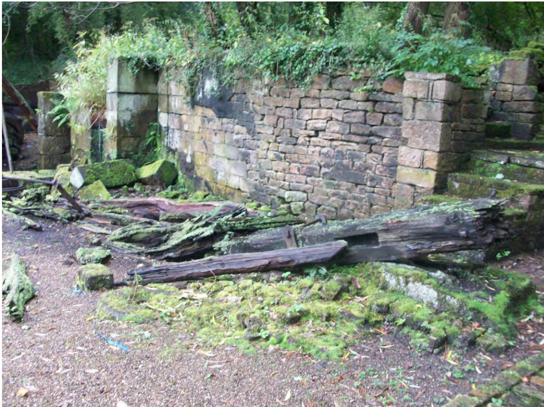
Shot of collapsed drop hammer (with dam wall behind)
