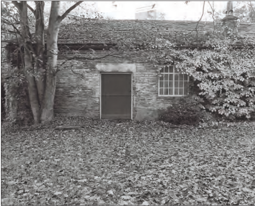
Plate 23: View of the north end of the southwest elevation of the former anvil store and workshop range (Film 1.3)
