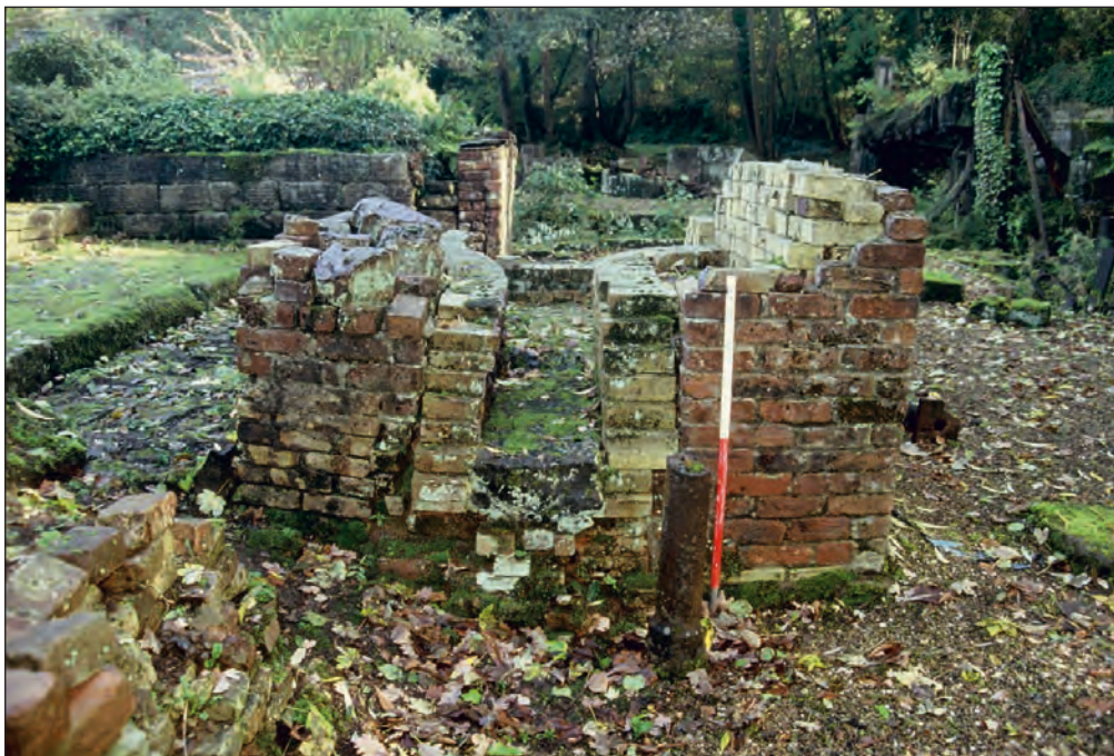
Plate 88: Detail of the northwest elevation/flue of the puddling furnace at the north side of the western phase 2 range (Film CS. 8)
