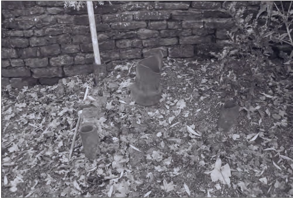
Plate 97: Detail of a former chimney base at the west side of the western phase 3 range (Film 10.31)
