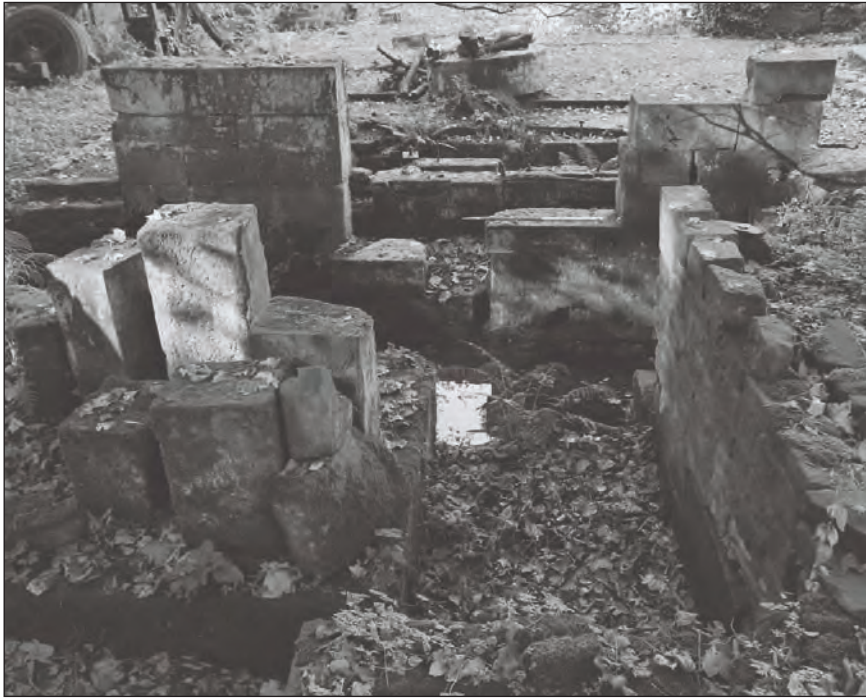
Plate 54: View of remains of wheel pit 4 adjacent to former grinding shop, south-eastern side of the central phase 1 former forge building (Film 5.4)
