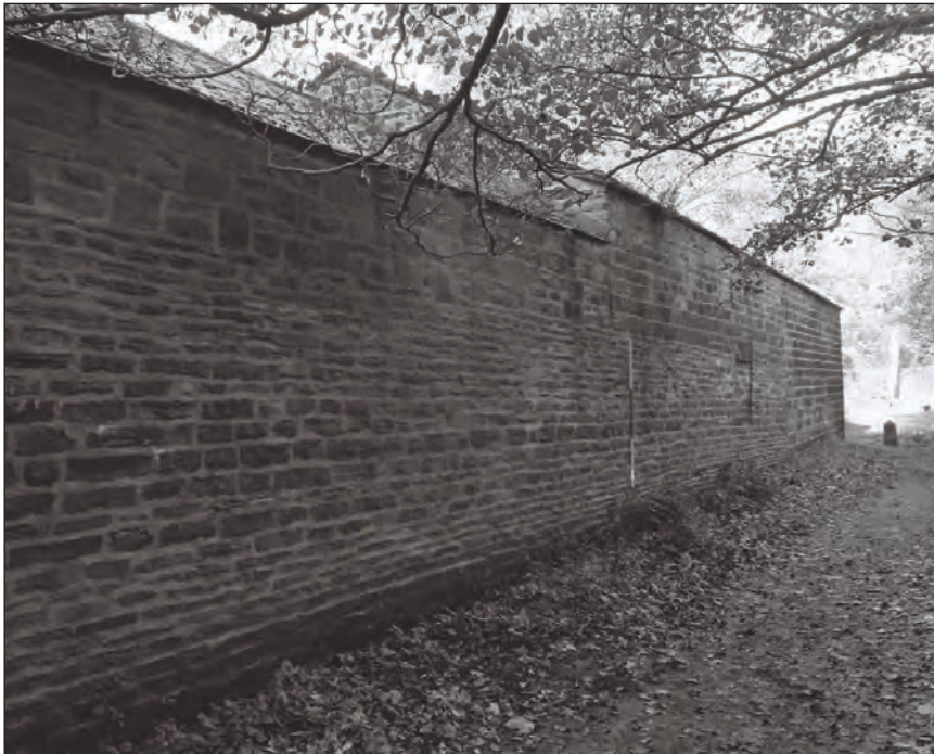
Plate 18: General view of the northeast elevation of the former anvil store and workshop range (Film 2.4)
