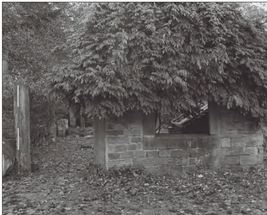
Plate 36: General view of the northeast elevation of the central phase 1 former forge building (Film 3.5)
