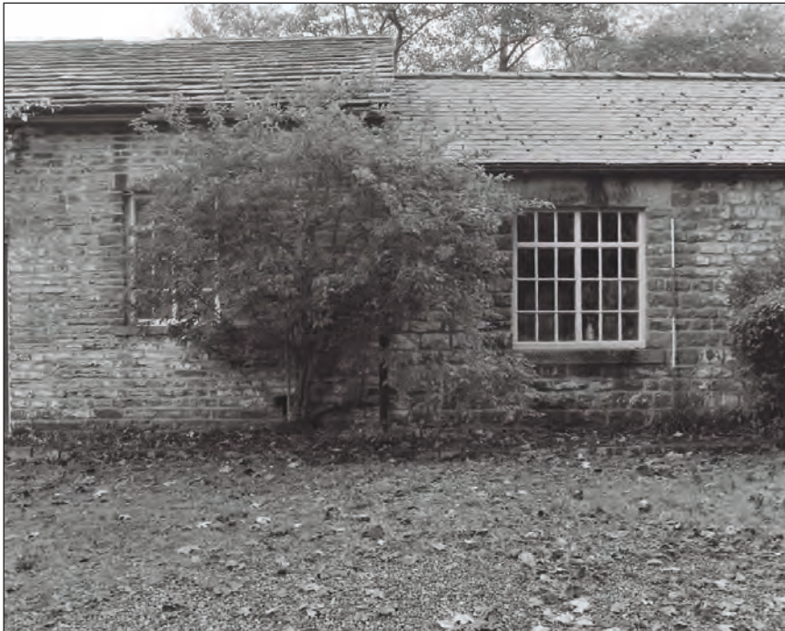
Plate 26: View of the southwest elevation of the former anvil store and workshop range (Film 1.5)
