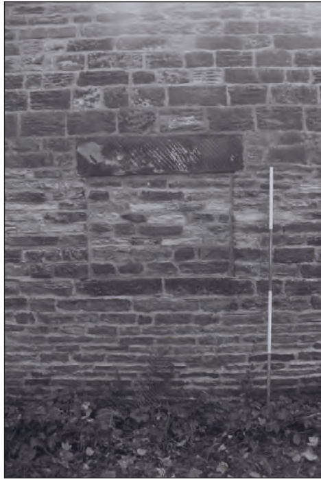
Plate 19: Detail of blocked window within the northeast elevation of the former anvil store and workshop range (Film 7.6)
