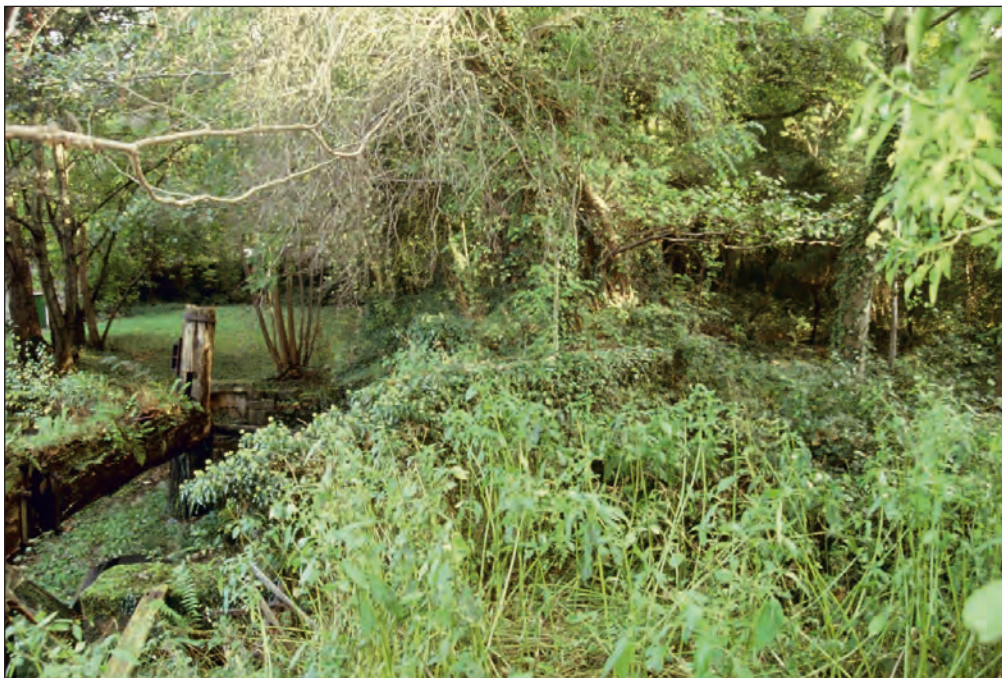
Plate 78: General view of the dam wall behind the east helve hammer, from the dam wall (Film CS. 42)
