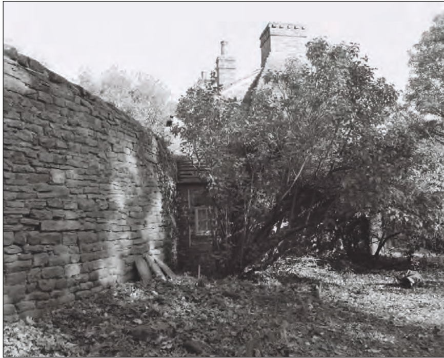
Plate 15: General view of the southwest gable elevation of the former Manager's House and attached furnace (Film 6.5)
