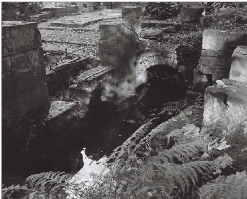
Plate 53: View of remains of wheel pit 4 adjacent to former grinding shop, south-eastern side of the central phase 1 former forge building, and tail goit (Film 5.3)
