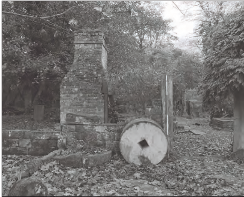
Plate 37: General view of the northeast elevation of the central phase 1 former forge building, showing truncated hearth and chimney stack (Film 3.6)
