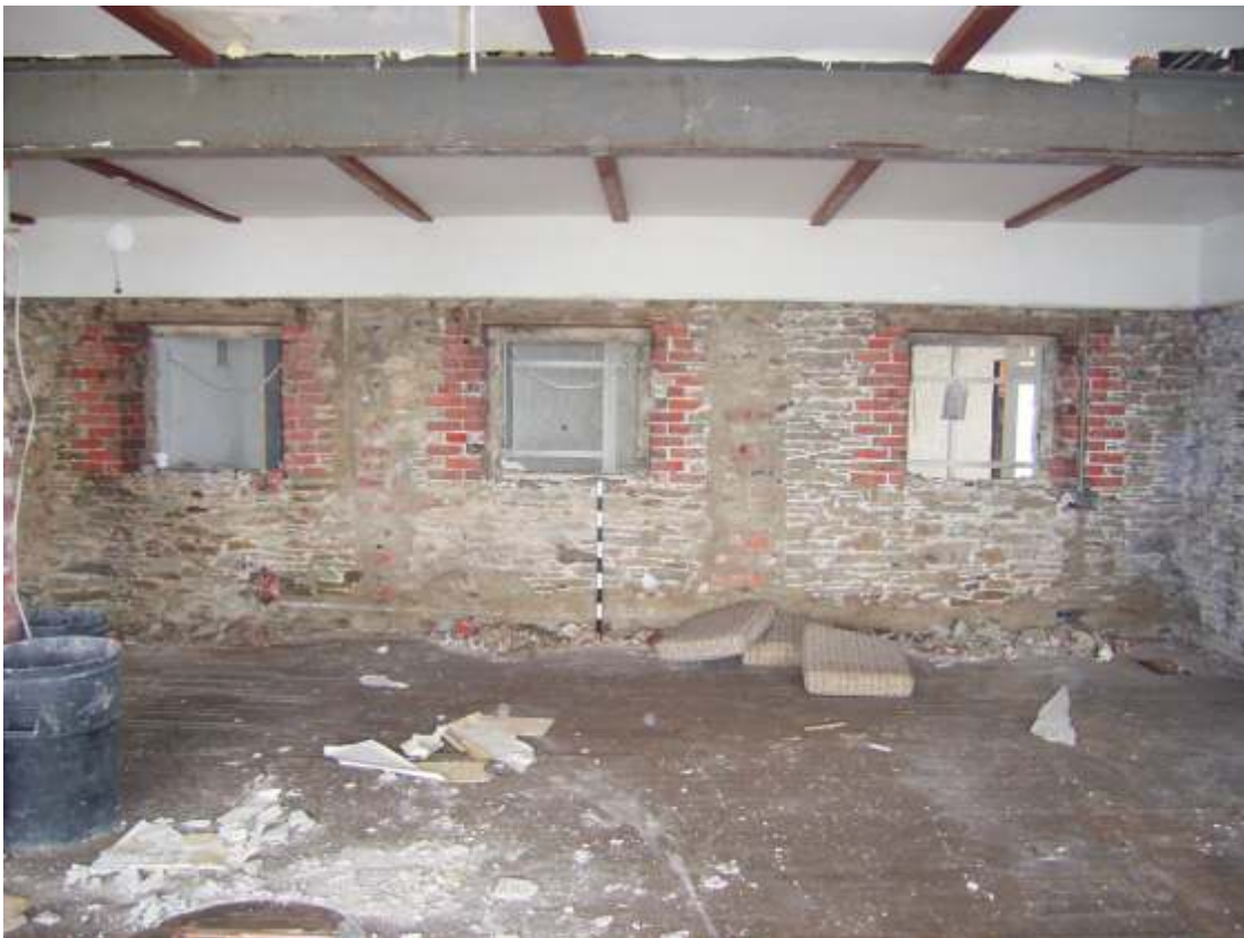
Plate 12. Ground floor lounge showing original window openings and vertical scarring on wall, indicating partitioning
