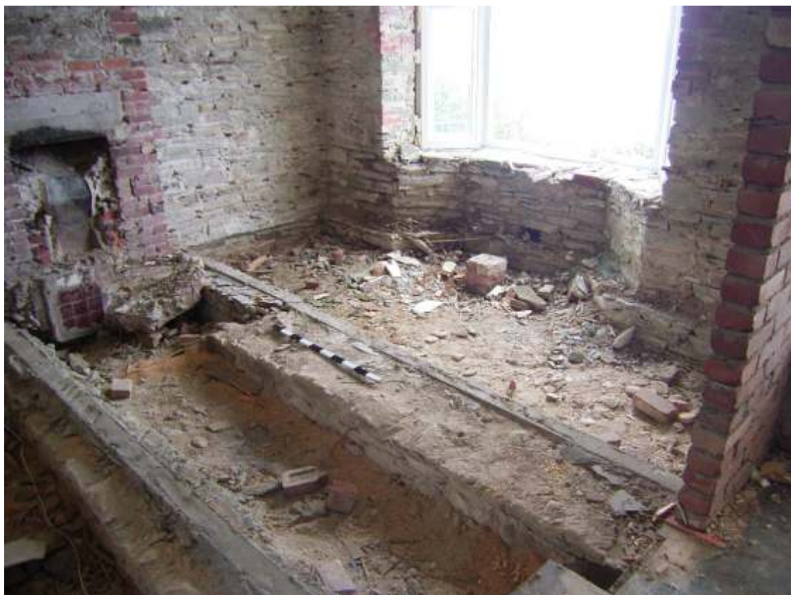
Plate 14. Exposed section of surviving 19th century front south wall foundation at east end of range
