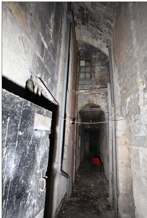
Plate 14: Sub-basement 10 Bridge Street. Line of Slippery Lane and high level window viewed from the east.
