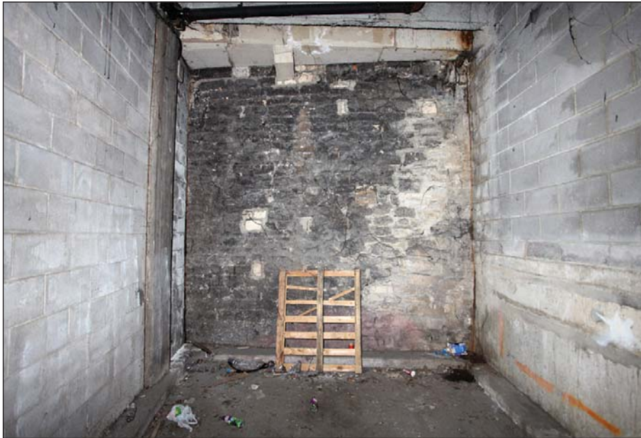
Plate 17: Sub-basement. Possible section of rubble stone north wall of 12 Bridge Street visible from underground car park
