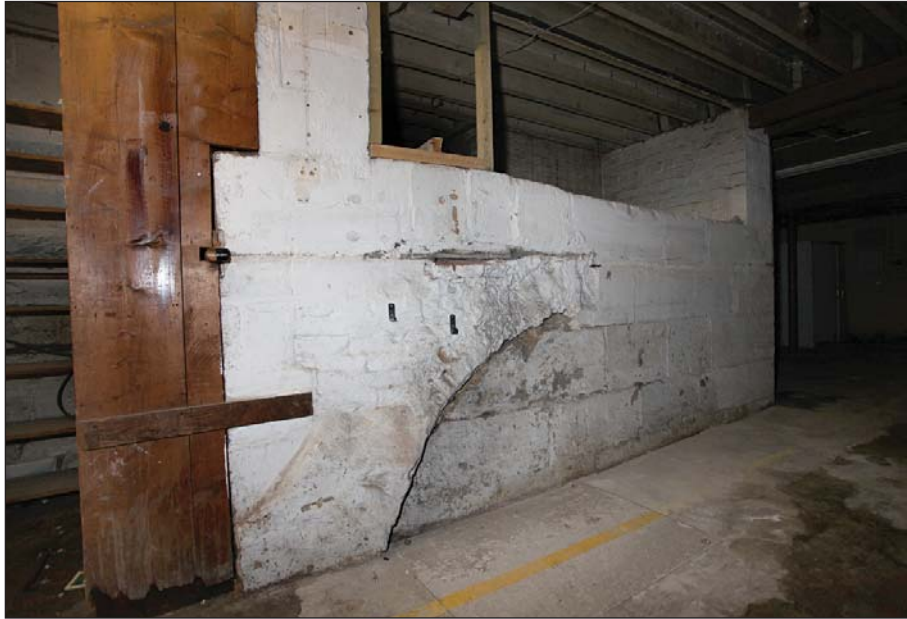
Plate 22: Earlier masonry arch incorporated into mid-19th century wall in 12 Northgate Street basement.
