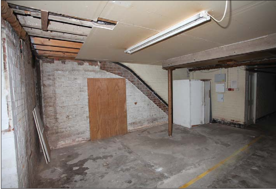
Plate 19: Basement 12 Northgate Street south wall brickwork indicating removed staircase to ground floor
