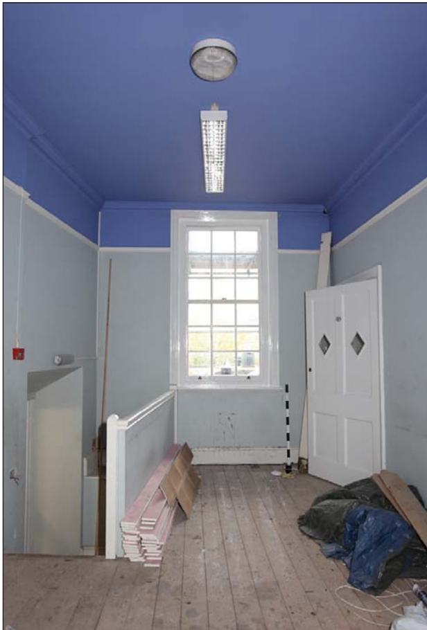
Plate 46: 1st floor, 12 Northgate Street, door to former lift shaft on right of image
