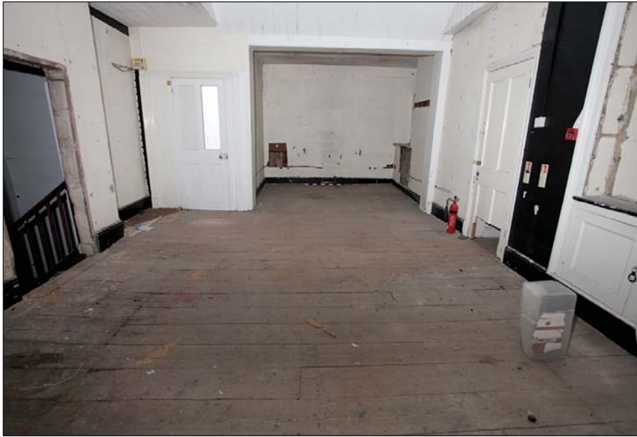
Plate 40: Ground floor SLe showing blocked door into SLd on right of image
