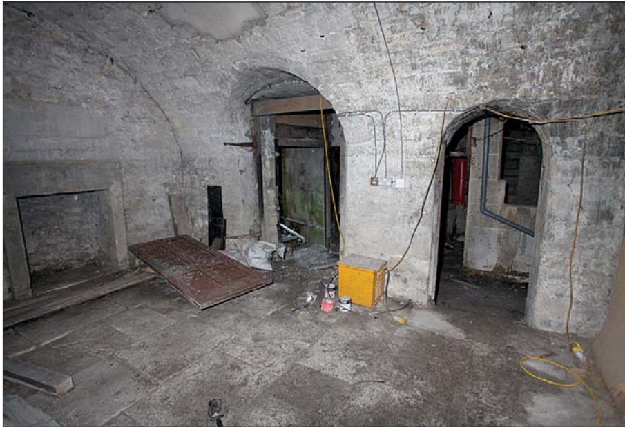
Plate 9: Sub-basement under number 8 Bridge Street showing original vaulting, fireplace and entrances onto Slippery Lane
