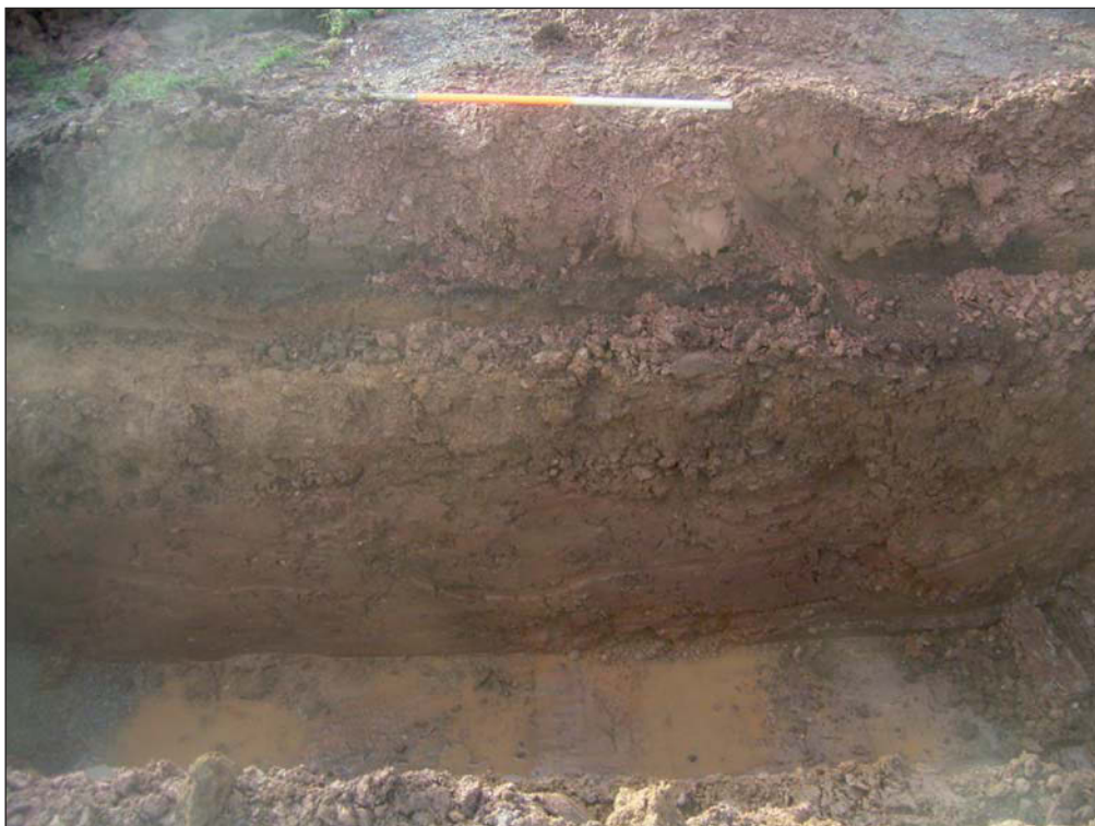
Plate 4: Sample section through ground exposed during manhole excavation, south of Peartree Close.
