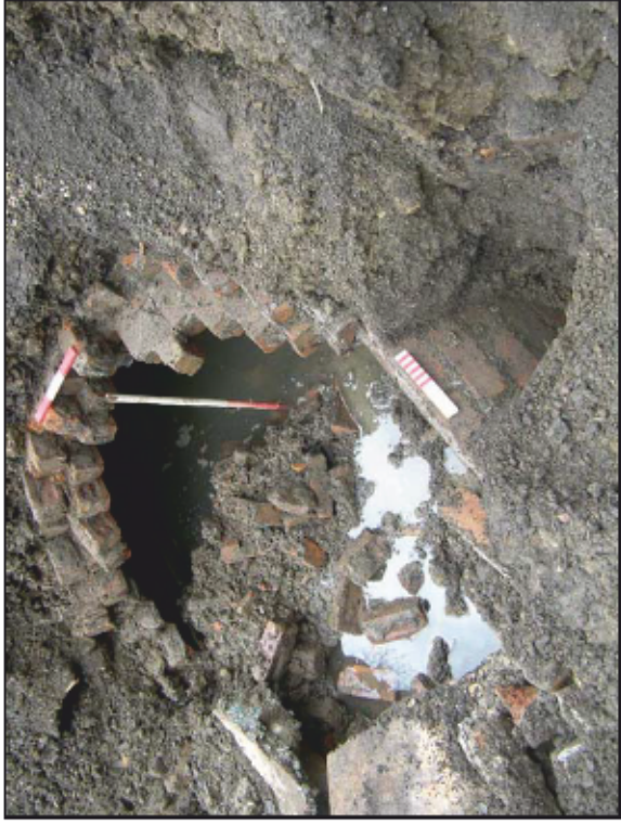
View of the Culvert exposed at the western side of the Site, looking south-west
