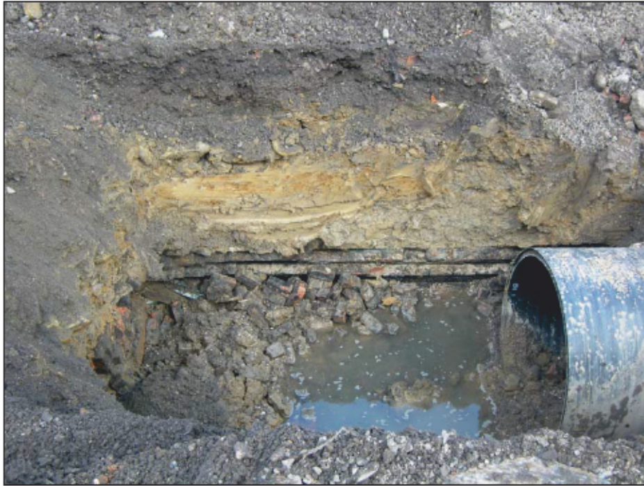
Plate 1: View of the Culvert exposed at the eastern side of the Site
