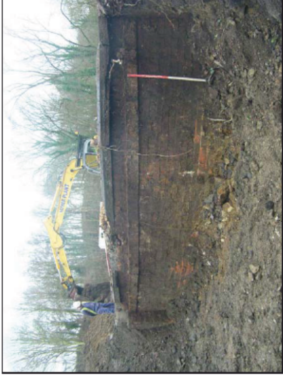
View of the external face of Gas Holder 1's cistern, looking west
