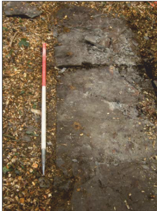
Plate 6: Detail of holes for former railing along coping stones 003 of Gas Holder 1's cistern
