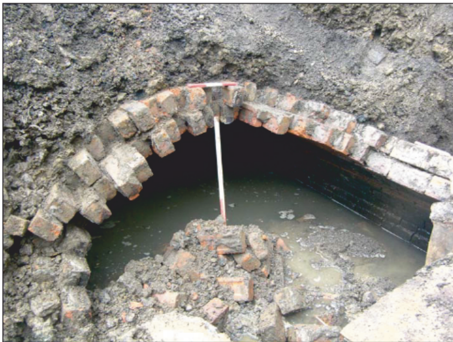
Plate 2: View of the Culvert exposed at the western side of the Site
