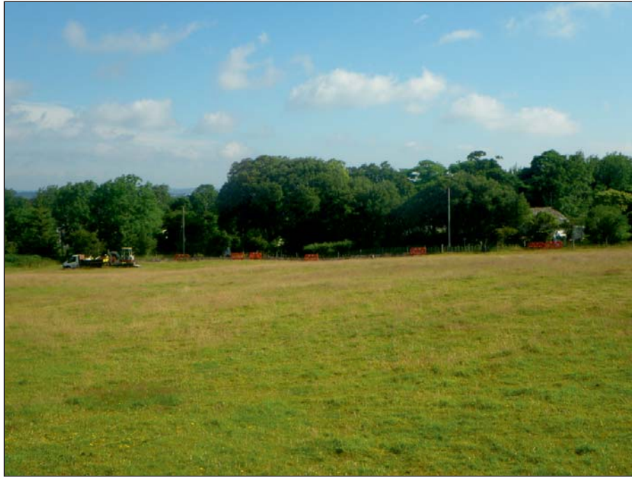
Plate 1: Working shot of the site showing the location of the cable trench
