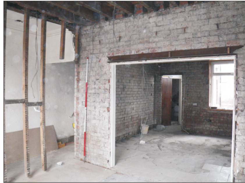
Plate 14: General view of rooms G4-6 forming ground floor of dwelling, looking west from room G4.
