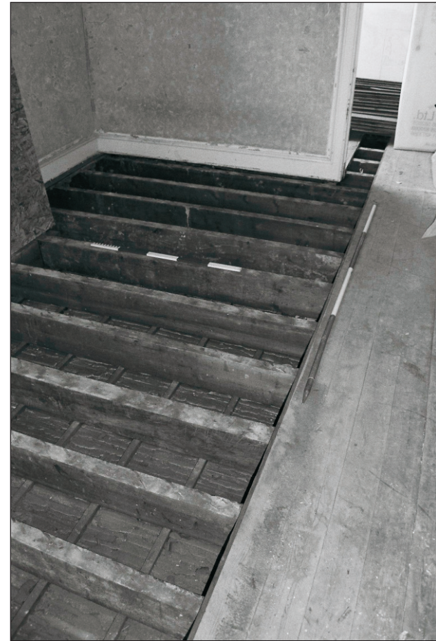
Plate 239: Detail of exposed timber floor structure, room F16, West Side of the North Range - OB. 42 (Film 53.20)
