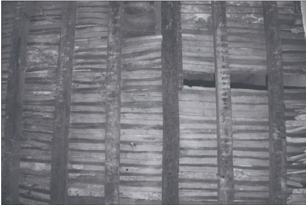
Plate 103: Detail of timber joists and laths of floor above, room G9/10, Central Entranceway of the North Range (Film 26.03)
