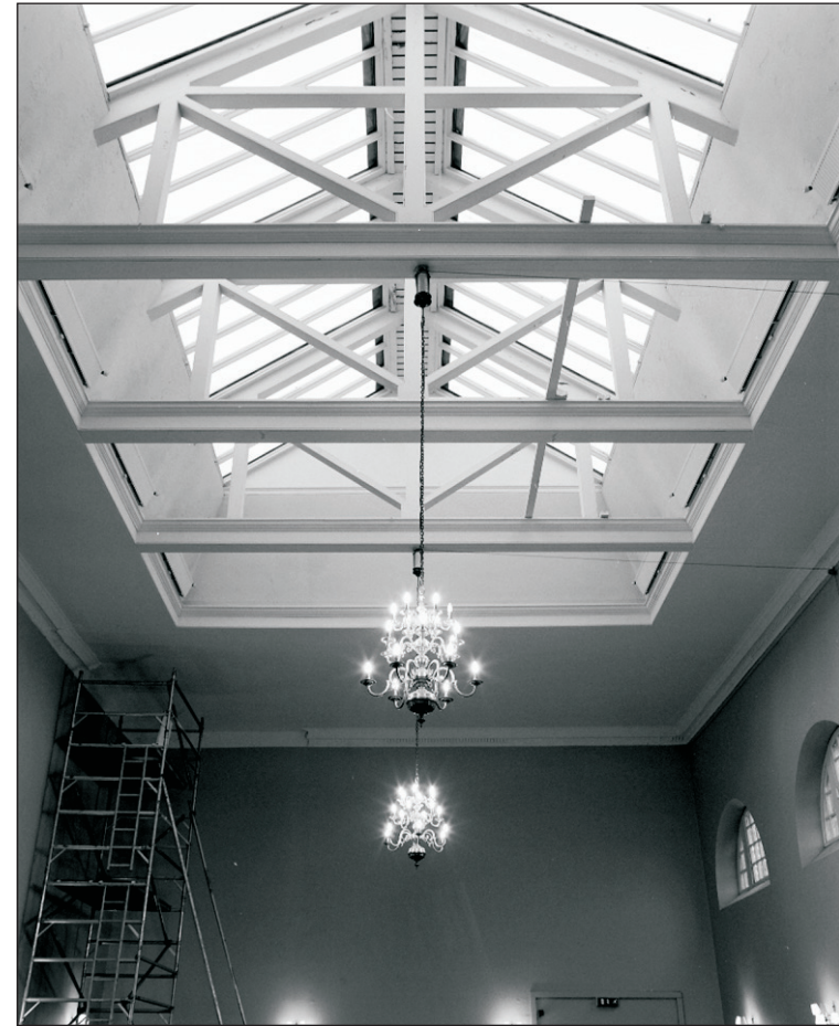
Plate 400: View of King-Post roof trusses and inserted skylights, G30, South Range (Film 09.06)
