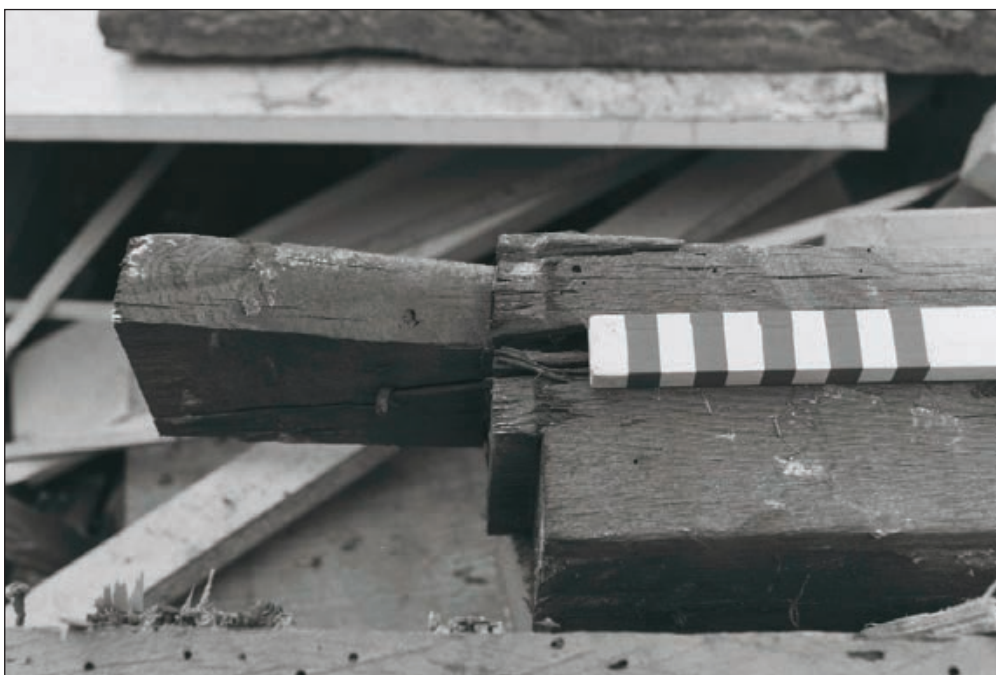
Plate 220: Detail of removed timber floor joists from room F13, Central Entranceway of the North Range, showing dovetail joint (Film 69.16)
