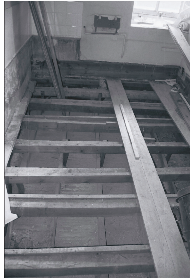
Plate 541: Detail of exposed timber floor and ceiling construction, F35, South Range - Agent's House - OB. 77 (Film 67.25)
