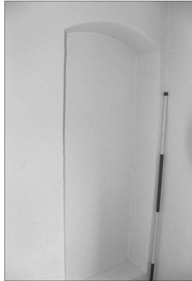
Plate 164: View of blocked door in west wall of room F8, Central Entranceway of the North Range (Film 15.30)
