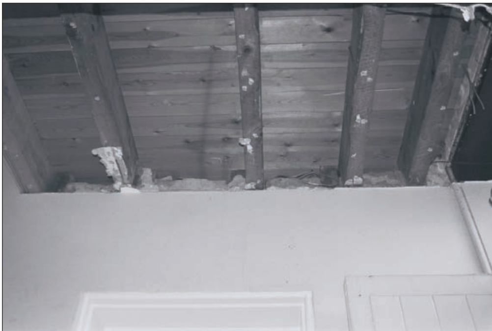
Plate 523: View of inserted modern joists for F41 above and position of removed inserted ceiling, G53, South Range - Agent's House (Film 46.07)
