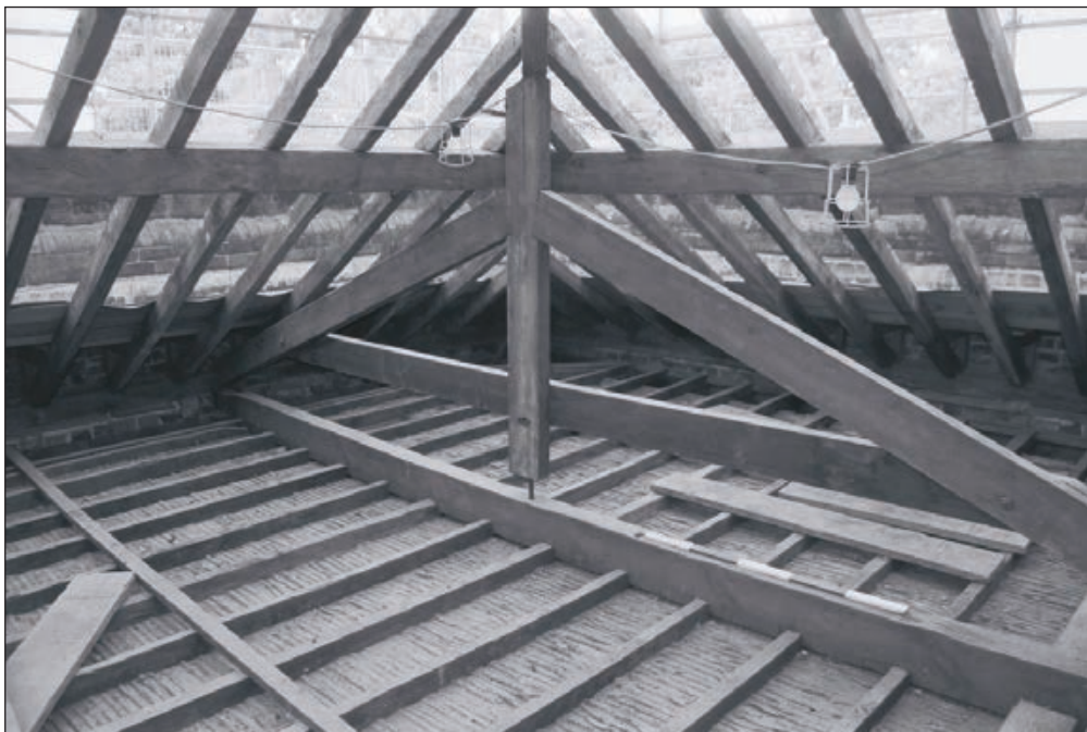
Plate 416: View of secondary roof truss of hipped roof structure of the Riding House, above G30, South Range - OB. 67 (Film 55.30)
