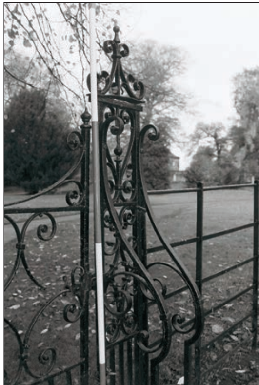
Plate 336: Detail of iron gates to the south rose garden, looking northwest (Film 12.25)
