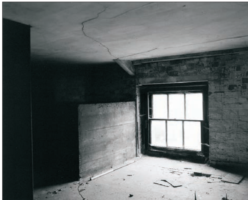
Plate 149: General view of room F4, East Side of the North Range, showing window and timber hoppers (Film 05.05)
