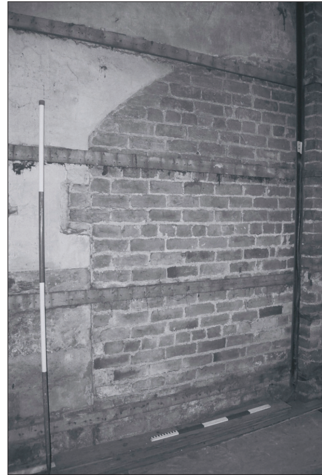
Plate 87: Detail of brick blocked arch, east wall of room G4, 'Tack Room', Central Entranceway of the North Range - OB.71 & 75 (Film 57.25)
