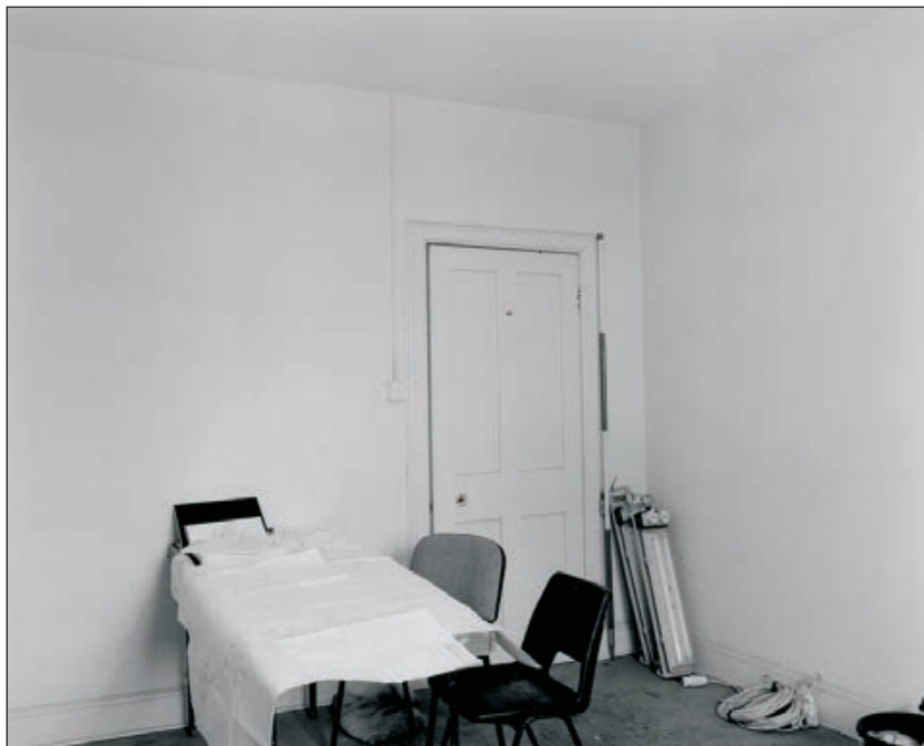
Plate 237: General view of room F16, West Side of the North Range (Film 30.10)
