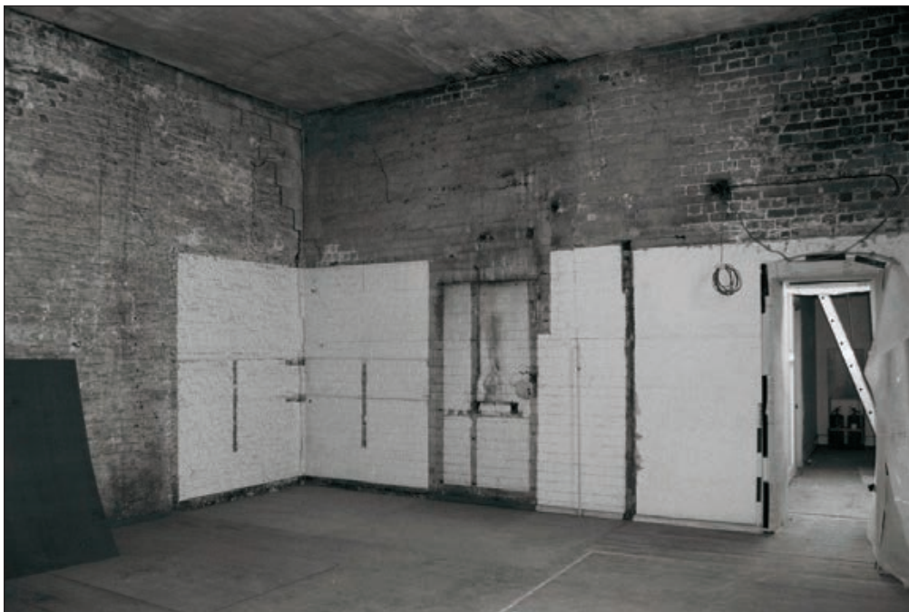
Plate 322: General view of F27 after removal of inserted rooms F23-F26, West Range (Film 52.03)
