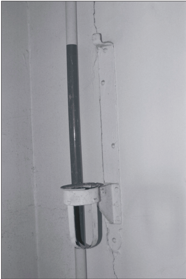
Plate 222: Detail of metal bracket on south wall of corridor F14, West Side of the North Range (Film 25.29)
