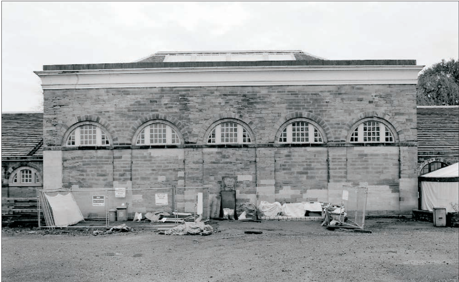
Plate 361: General view of the north courtyard elevation of the central Riding House, South Range (Film 18.08)
