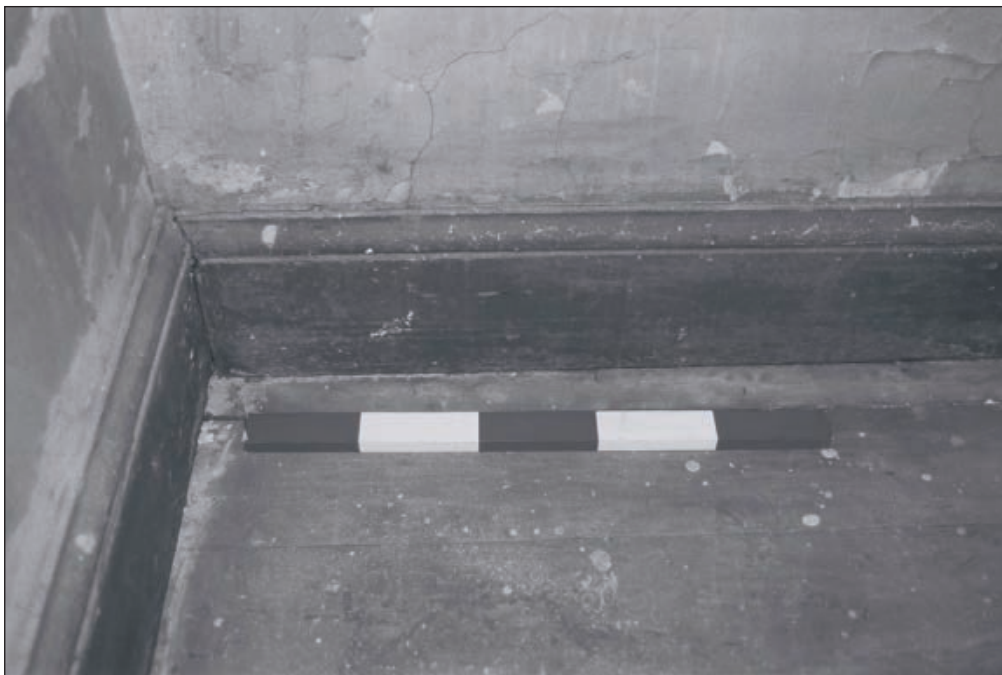
Plate 227: Detail of skirting boards, room F15, West Side of the North Range (Film 25.20)
