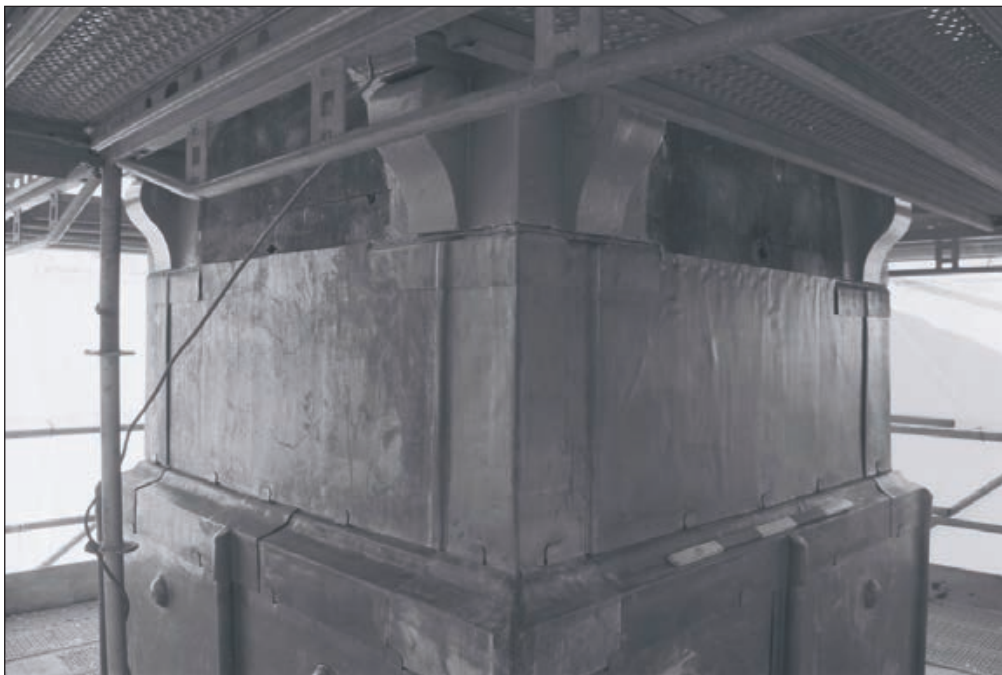
Plate 192: Detail of clock tower, F10a, Central Entranceway of the North Range - OB. 84 (Film 68.09)
