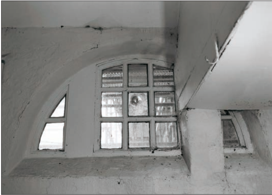
Plate 501: View of high window, north wall of G43, South Range - Agent's House - showing inserted tank above (Film 61.02)
