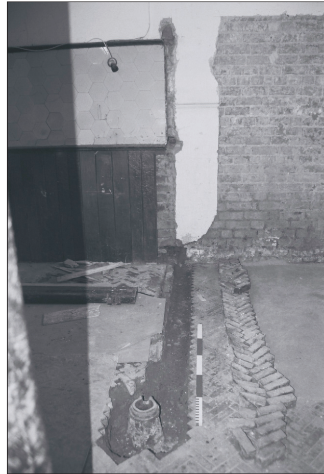
Plate 584: Detail of removed cast iron loose box column, partition and brick floor, G55, East Range (Film 45.25)
