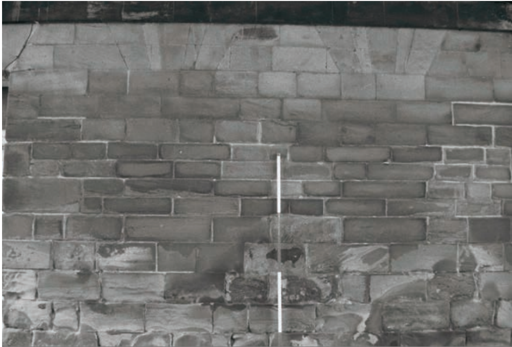
Plate 20: Detail of blocked windows within the east facing elevation of the North Range cart passage (G7) (Film 20.27)
