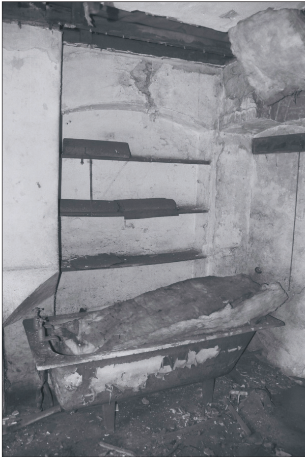
Plate 210: General view of northwest corner of F13, Central Entranceway of the North Range, showing blocked opening (Film 42.03)
