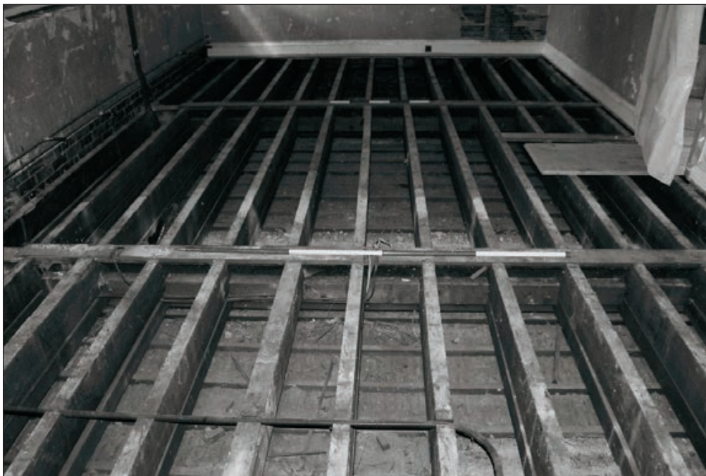
Plate 247: View of exposed timber and RSJ floor structure of rooms F17/19, West Side of the North Range - OB. 41 (Film 53.29)
