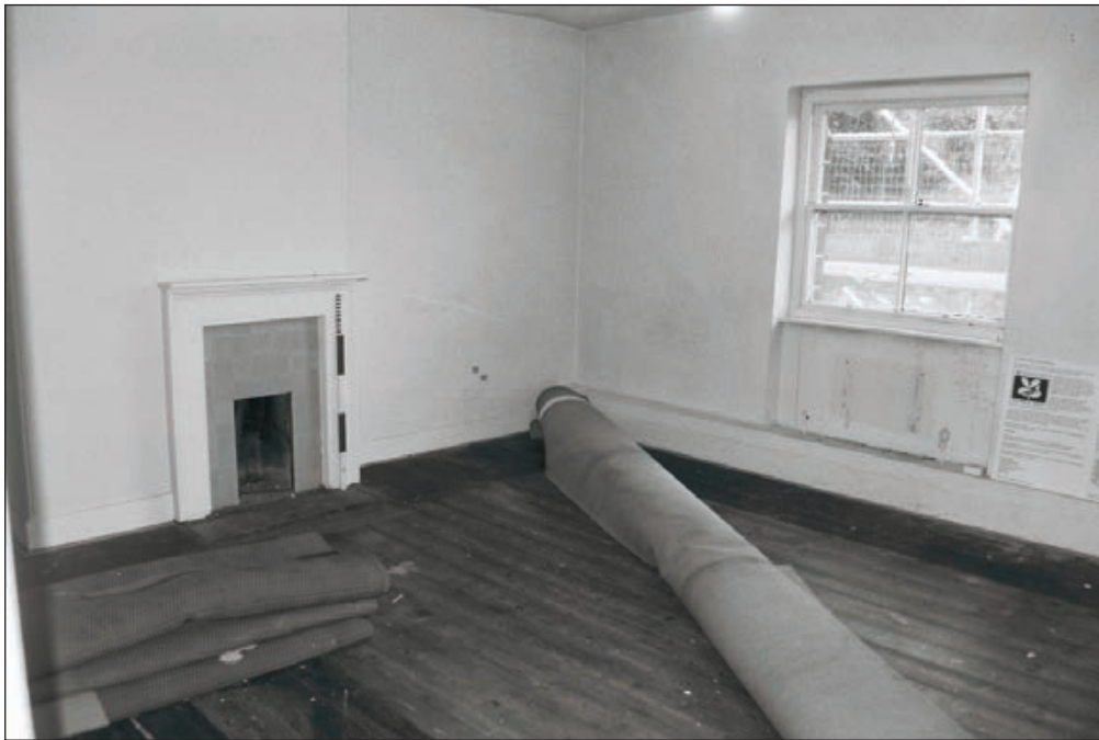
Plate 548: General view of F38, South Range - Agent's House - after removal of carpets (Film 66.31)
