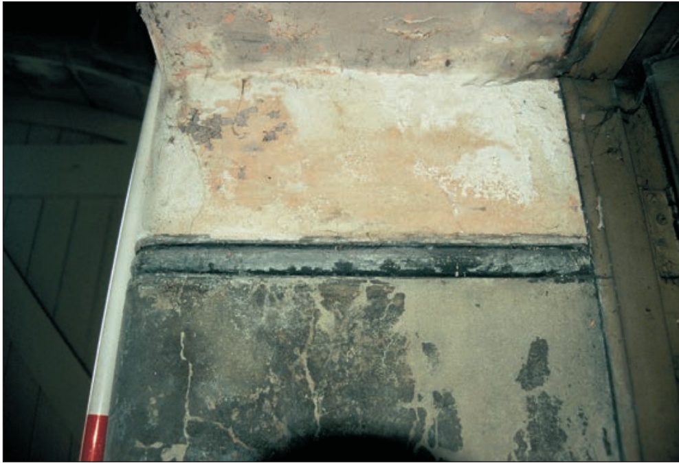
Plate 122: Detail of moulded plaster dado and paint scheme of room G15, West Side of the North Range (Film C.S. 24)
