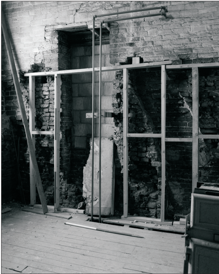
Plate 317: View of earlier south wall of F27, West Range, showing join with later north range, blocked doorway and flue (Film 36.08)
