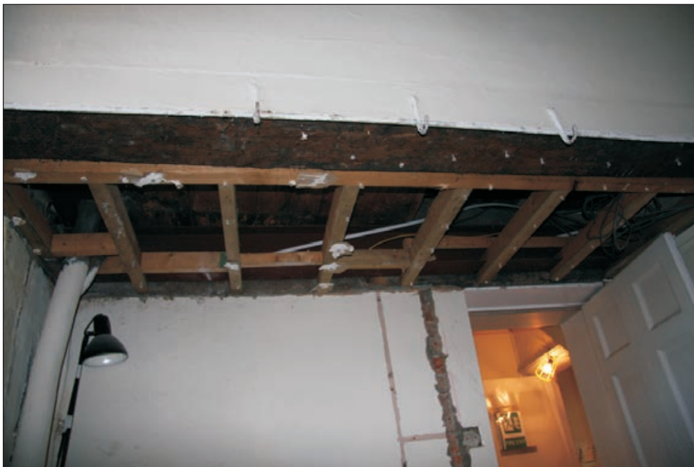
Plate 502: View of exposed reused timber beam and RSJ within G43, South Range - Agent's House - OB. 95 - for inserted floor and tank above (Film D. 20.10.10 1782)
