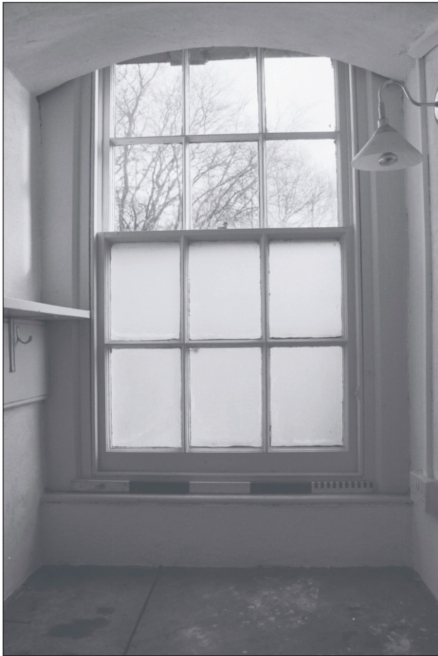
Plate 517: General view of G52, showing sash window in east wall, South Range - Agent's House (Film 44.35)
