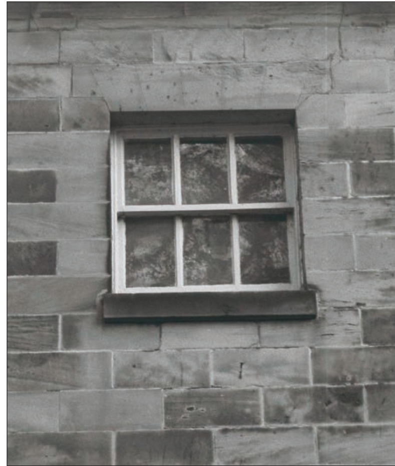
Plate 267: Detail of first floor window, west elevation of the West Range (Film 12.14)
