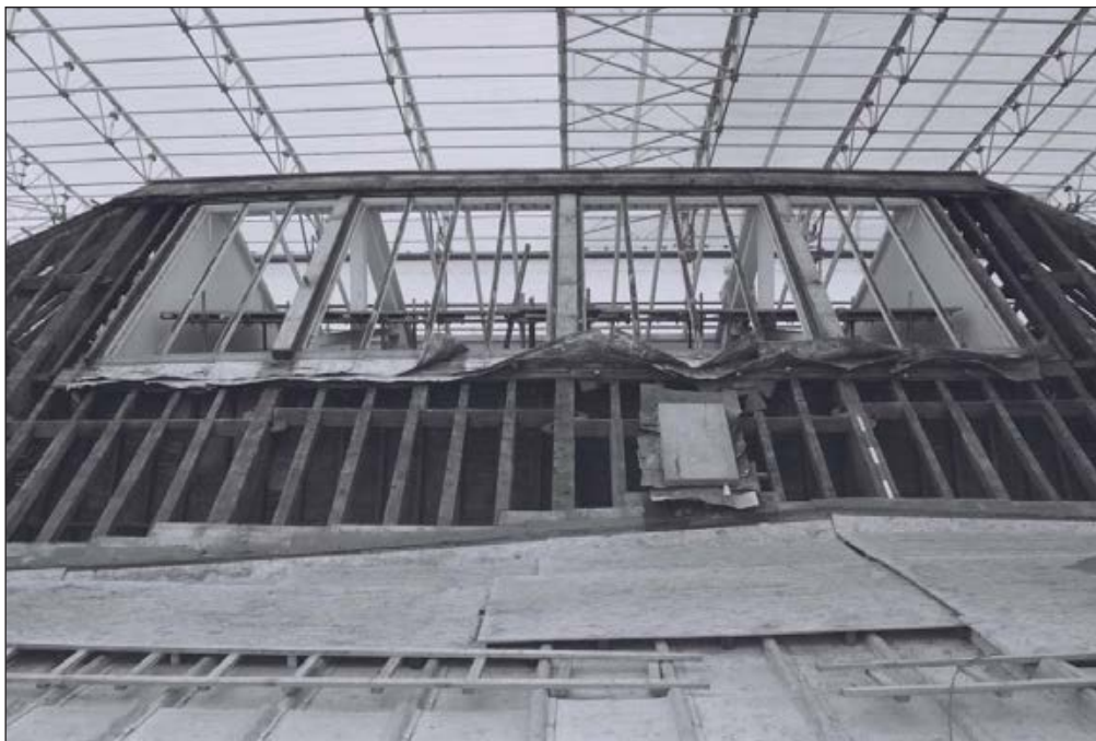
Plate 414: View of timber roof structure of the Riding House, above G30, South Range - OB. 104 - showing inserted skylights (Film 55.08)
