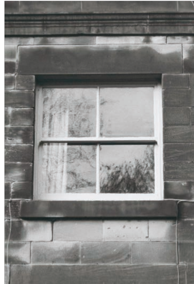
Plate 368: Detail of a first floor window at the south end of the east elevation of the South/East Range (Agent's House) (Film 11.30)
