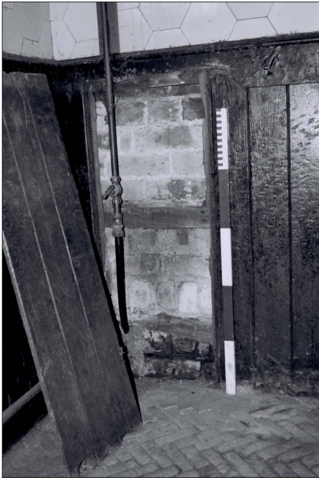
Plate 581: Detail of removed tongue and groove boarding, east wall of G55, East Range - OB. 12 (Film 43.5)
