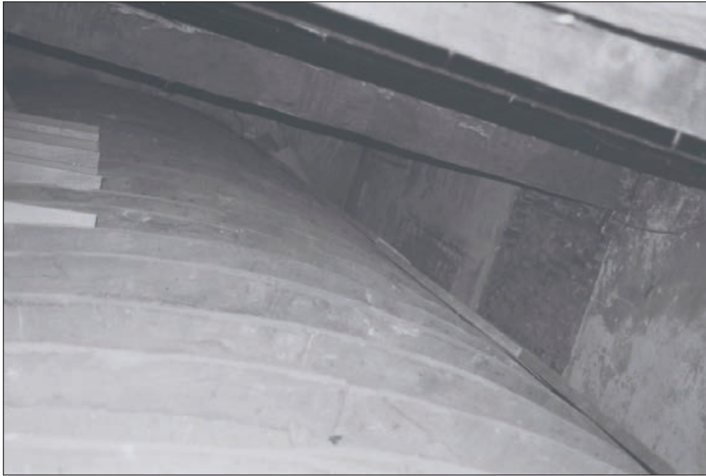
Plate 165: View of floor void F10b, Central Entranceway of the North Range - OB. 87 - showing inserted arch and blocked openings in west wall (Film 75.22)
