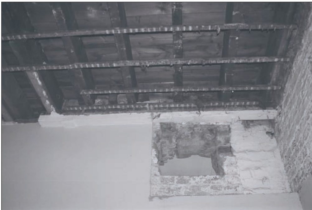
Plate 278: Detail of floor and ceiling structure above G17/19, West Range, after the removal of ceiling and - OB. 80, and inserted opening within wall - OB. 83 (Film 67.17)
