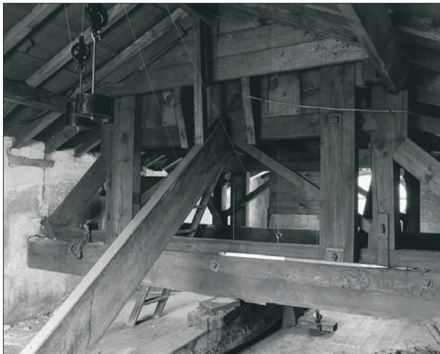
Plate 170: General view of F10, Central Entranceway of the North Range, showing clock tower structure (Film 33.03)
