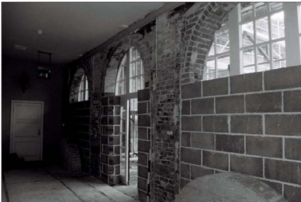
Plate 394: View of exposed brickwork, north wall of G29, South Range - OB. 105 (Film 72.07)
