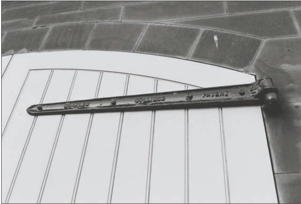
Plate 36: Detail of large cast iron hinges of the timber double doors of the west end of the south courtyard elevation of the North Range: 'CHARLES COLLINGS PATENT' (Film 20.23)
