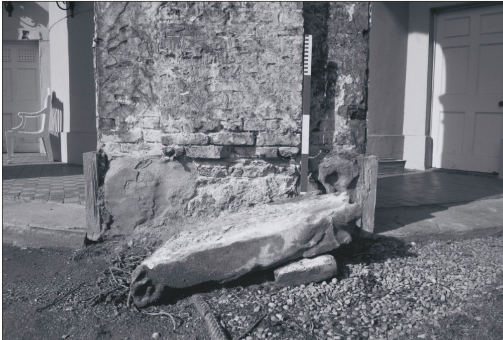
Plate 346: Detail of the exposed brick and stone fabric of the south elevation of the South Range - OB. 32 (Film 51.12)
