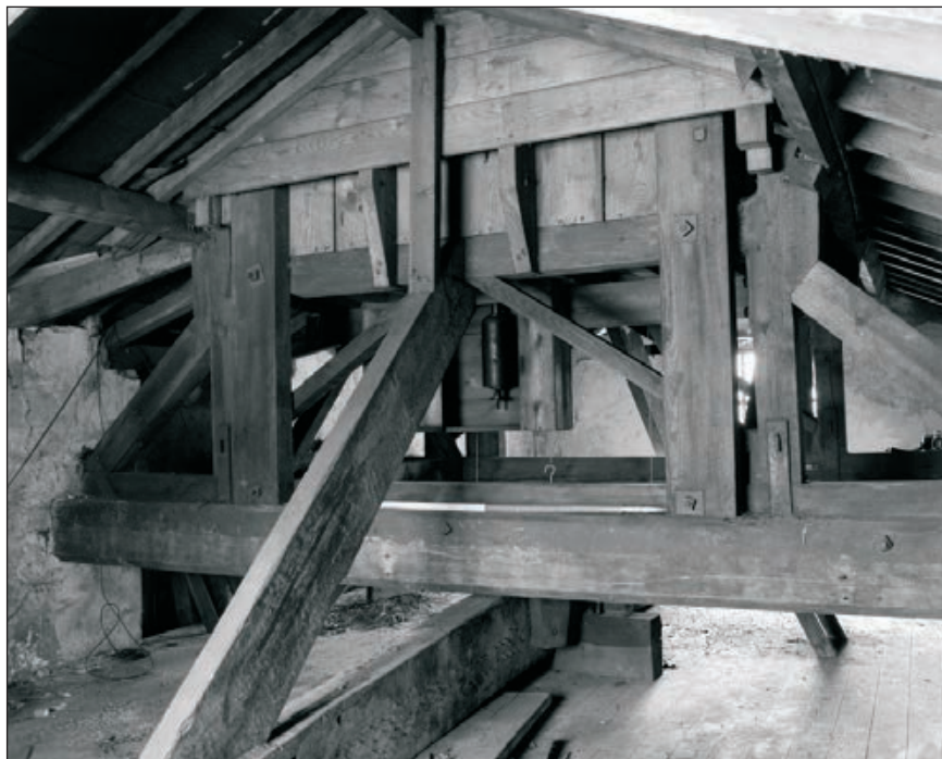
Plate 172: General view of F10, Central Entranceway of the North Range, showing clock tower structure (Film 33.08)
