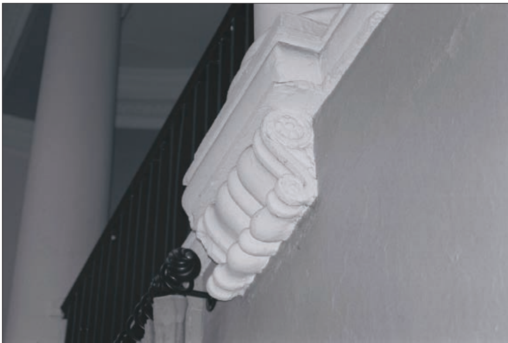
Plate 406: Detail of decorative plaster mouldings at base of balcony columns, south wall of G30, South Range (Film 23.01)
