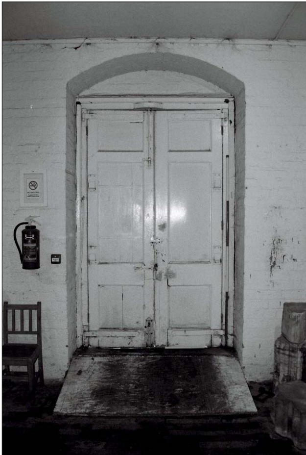
Plate 44: Detail of main doorway in north wall of G1, East Side of the North Range (Film 13.36)
