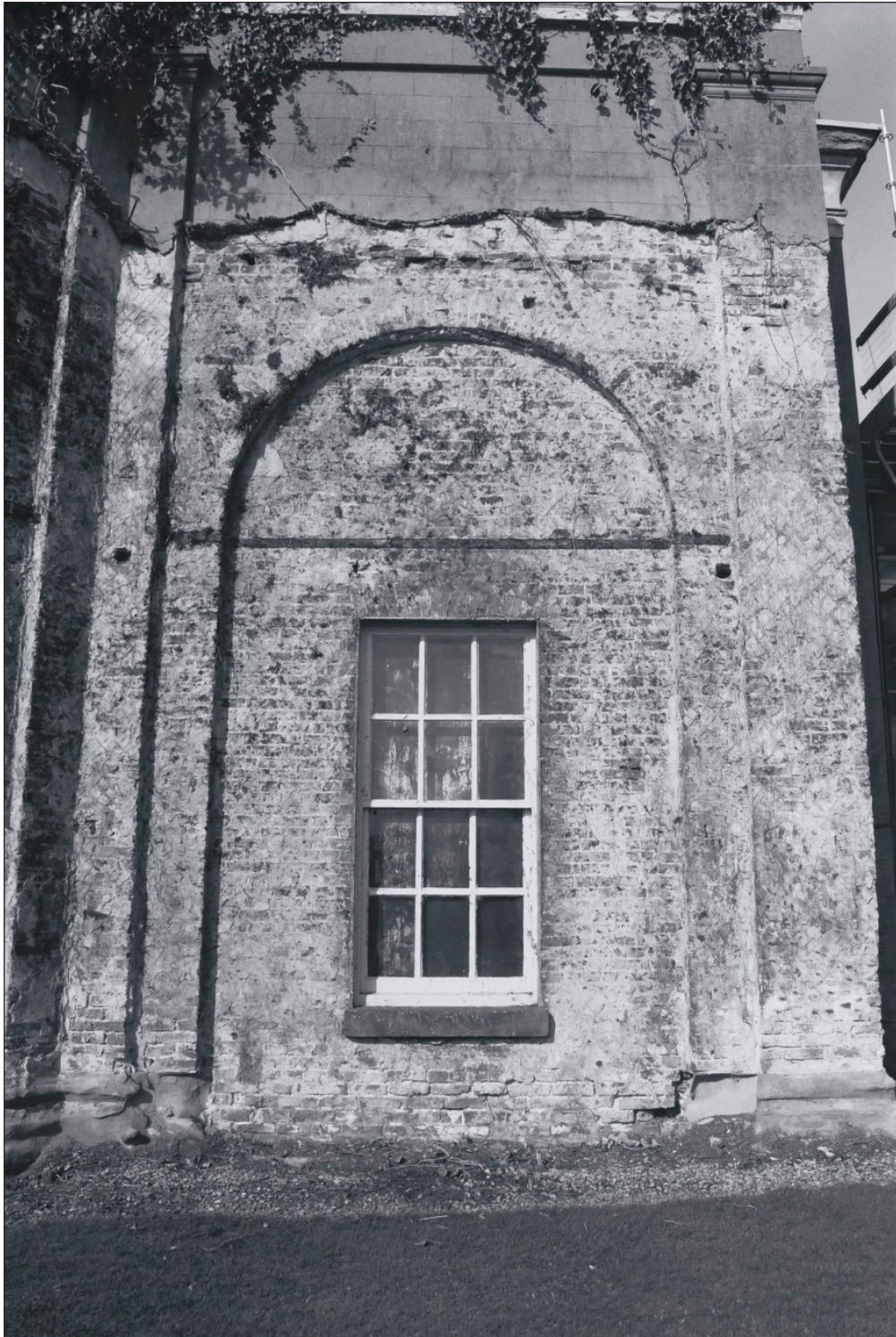
Plate 348: Detail of the exposed brick and stone fabric of the south elevation of the South Range, after the removal of vegetation - OB. 32 (Film 51.10)
