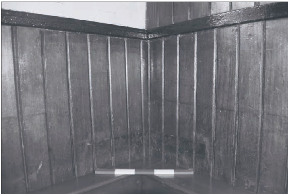
Plate 292: Detail of scar from removed trough or manger, northwest corner of loose box within G22, West Range (Film 23.22)
