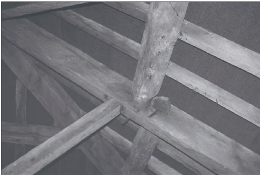
Plate 388: Detail of pegged timber purlins and trusses, roof void above F28, South Range - OB. 127 (Film 78.31)
