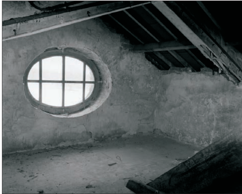
Plate 171: General view of the north side of F10, Central Entranceway of the North Range, showing oeil-de-boeuf window and hatch in floor to F10b below (Film 33.06)
