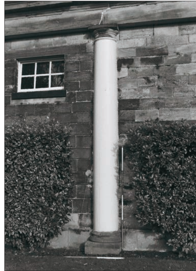
Plate 341: Detail of column with adjacent stone infills, south elevation of the Garden Room, South Range (Film 12.29)
