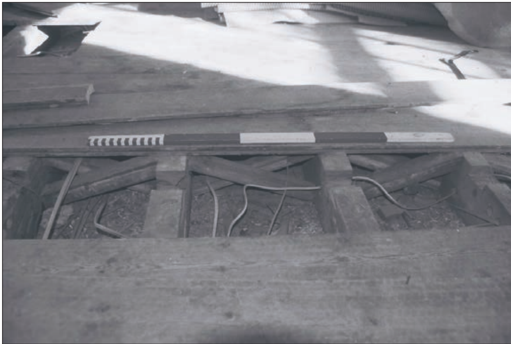
Plate 558: Detail of exposed noggins between joists, F40, South Range - Agent's House - OB. 82 (Film 67.27)
