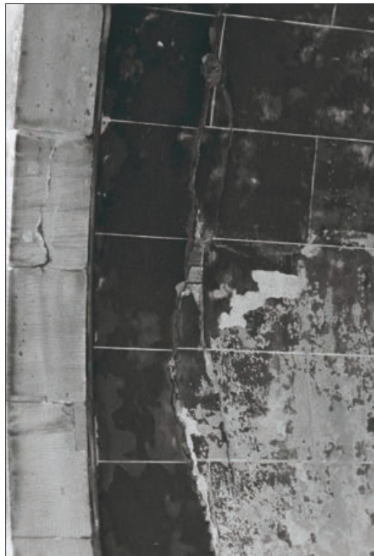
Plate 21: Detail of inserted lath and plaster arched ceiling of the North Range cart passage (G7) (Film 20.31)
