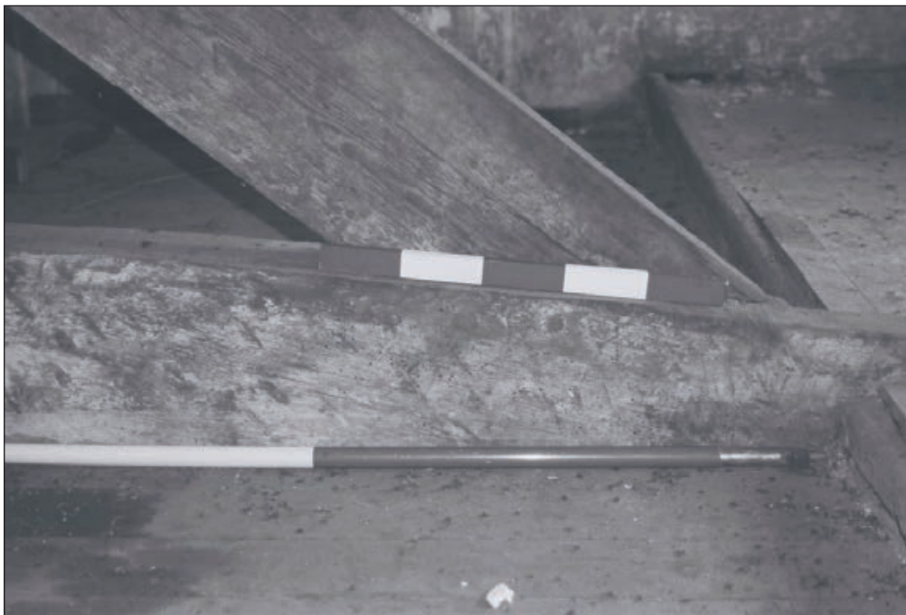
Plate 178: Detail of pegged trusses of timber clock tower structure, F10, Central Entranceway of the North Range (Film 42.24)
