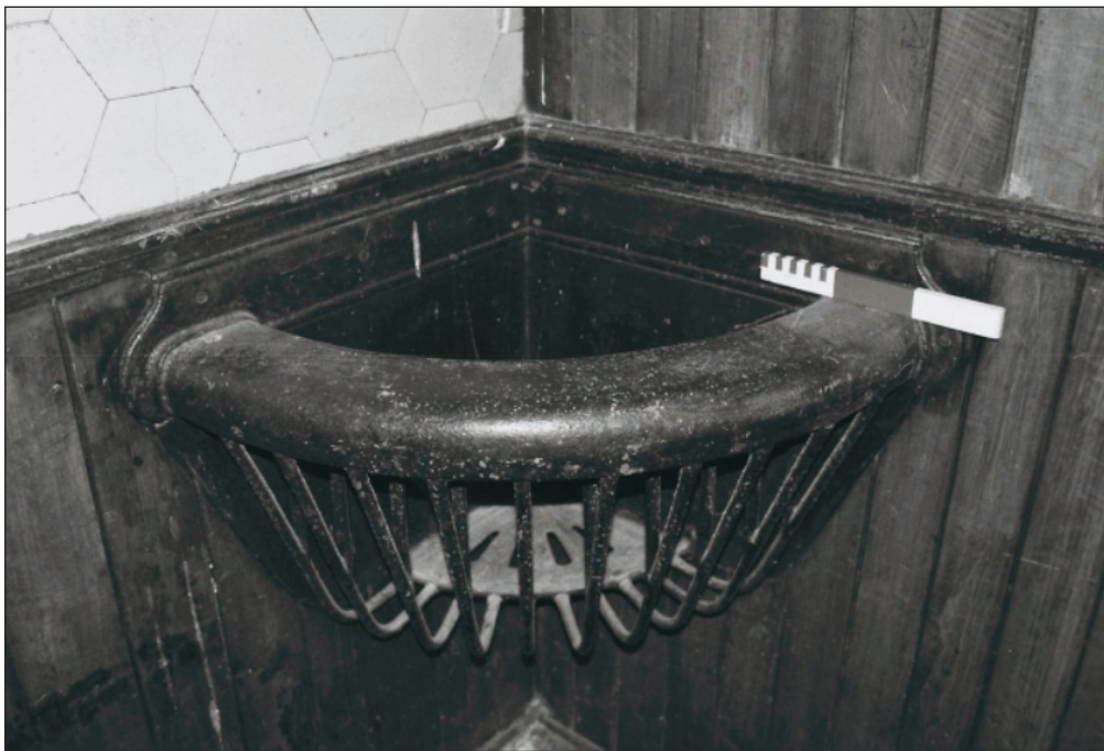
Plate 51: Detail of original Musgrave corner hay rack, room G2, East Side of the North Range (Film 14.22)
