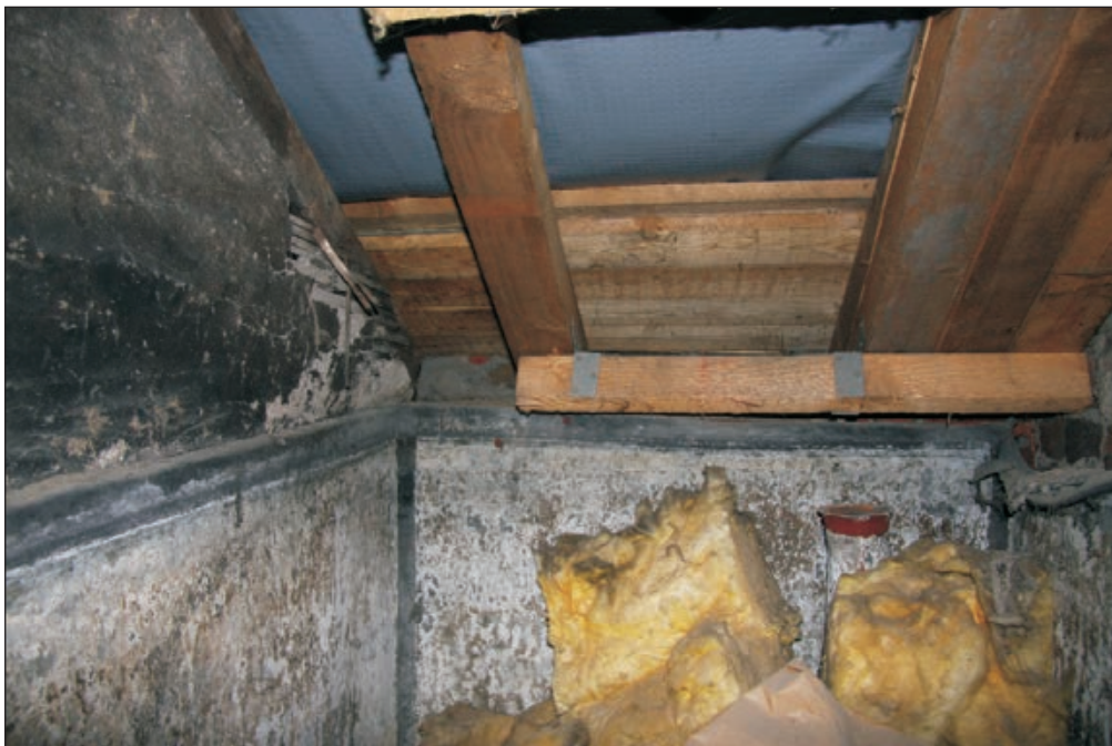
Plate 543: View into inserted tank within east end of Roof Void 13, above G43, from F34/39, South Range - Agent's House - OB. 103 (Film D. 25.08.11 4798)
