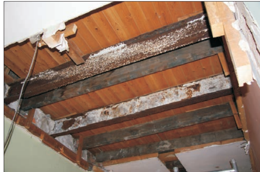
Plate 284: View of exposed modern timber and RSJ joists of ceiling and floor above G20/21, West Range - OB. 81 (Film D. 14.10.10. 1596)
