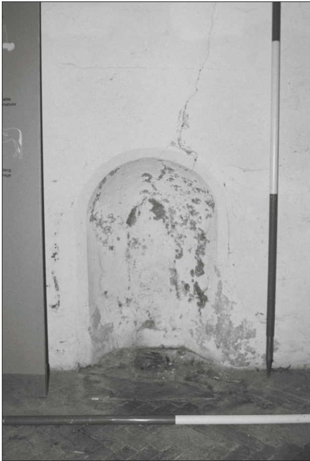
Plate 60: Detail of drainage recess within the south wall of room G2, East Side of the North Range (Film 14.13)
