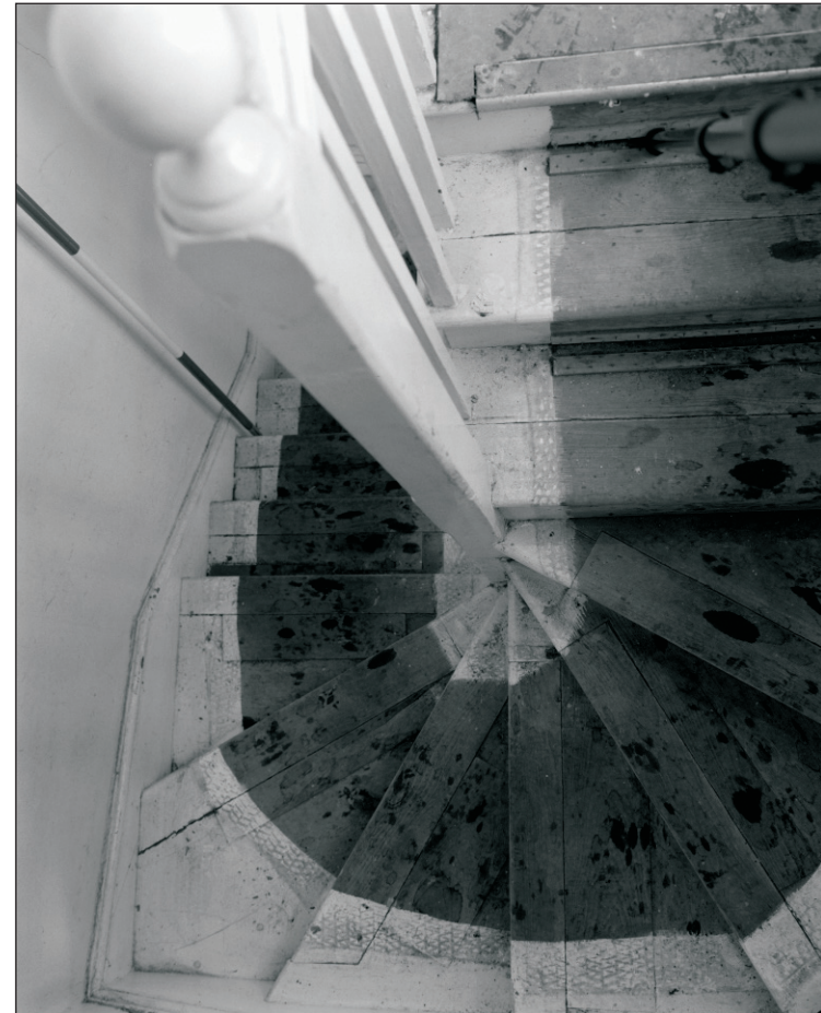
Plate 94: General view of staircase G8 to F11, Central Entranceway of the North Range (Film 32.02)
