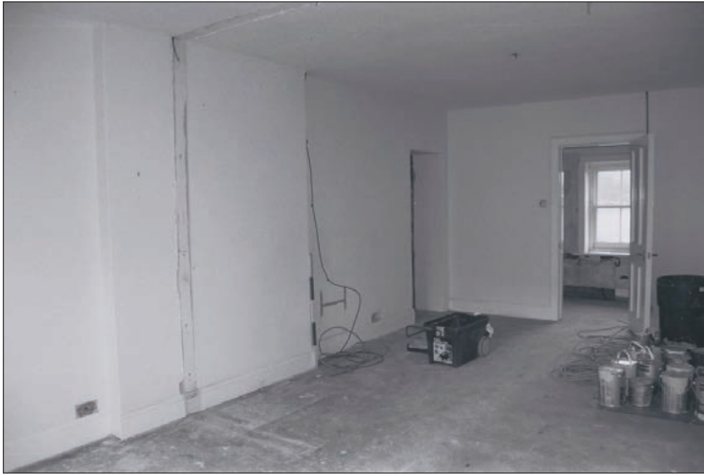
Plate 156: General view of rooms F7 and F6, East Side of the North Range, after removal of modern partitions - OB. 123 - showing limeash floor and blocked fireplace (Film 77.18)
