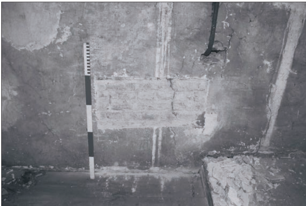
Plate 184: Detail of removed plaster on west wall of F10, Central Entranceway of the North Range, showing exposed brick fabric of wall - OB. 19 (Film 47.24)
