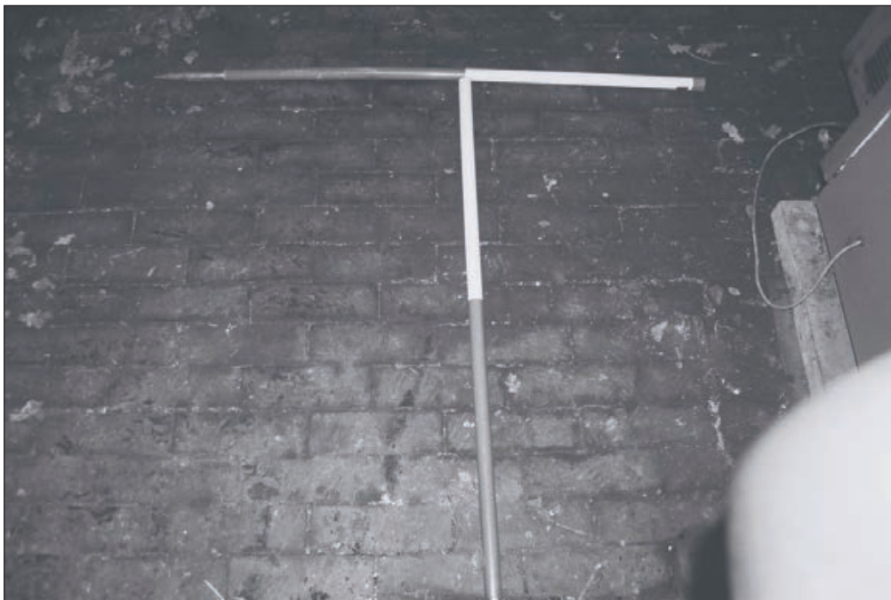
Plate 129: Detail of brick floor of room G16, West Side of the North Range (Film 26.23)
