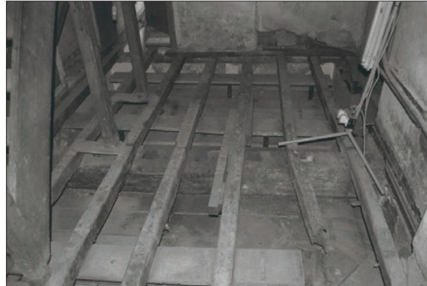
Plate 205: General view of exposed floor joists and beam after removal of limeash, F12, Central Entranceway of the North Range (Film 69.03)
