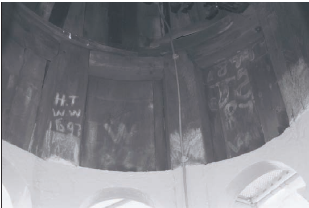
Plate 196: Detail of graffiti within clock tower, F10a, Central Entranceway of the North Range - OB. 84 (Film 68.13)
