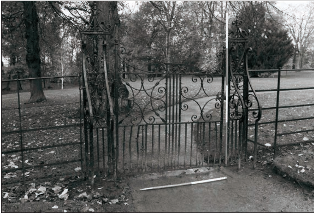
Plate 335: Detail of iron gates to the south rose garden, looking northwest (Film 12.23)
