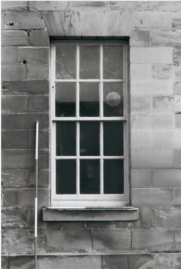
Plate 266: Detail of ground floor window, west elevation of the West Range (Film 12.11)
