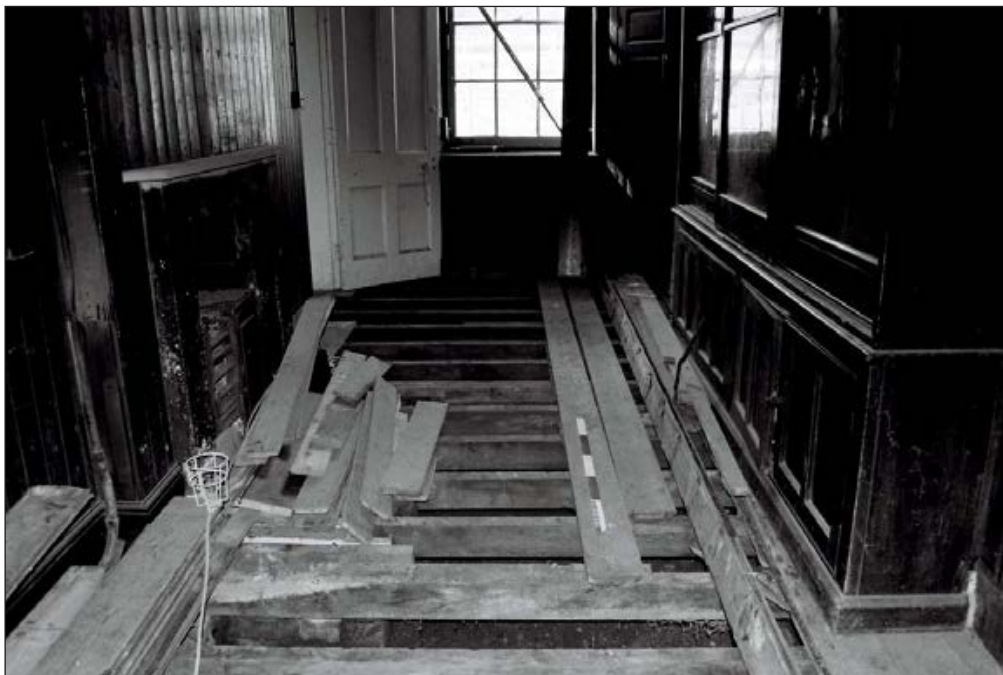
Plate 83: View of exposed floor structure, room G4, 'Tack Room', Central Entranceway of the North Range - OB. 34 (Film 52.29)
