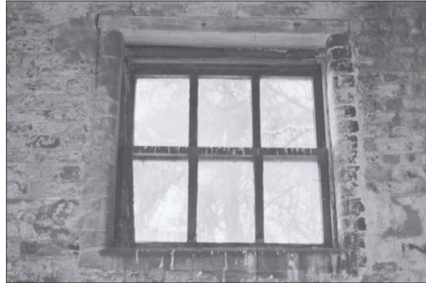
Plate 320: View of inserted window in phase 3 west wall of F27, West Range (Film 26.29)
