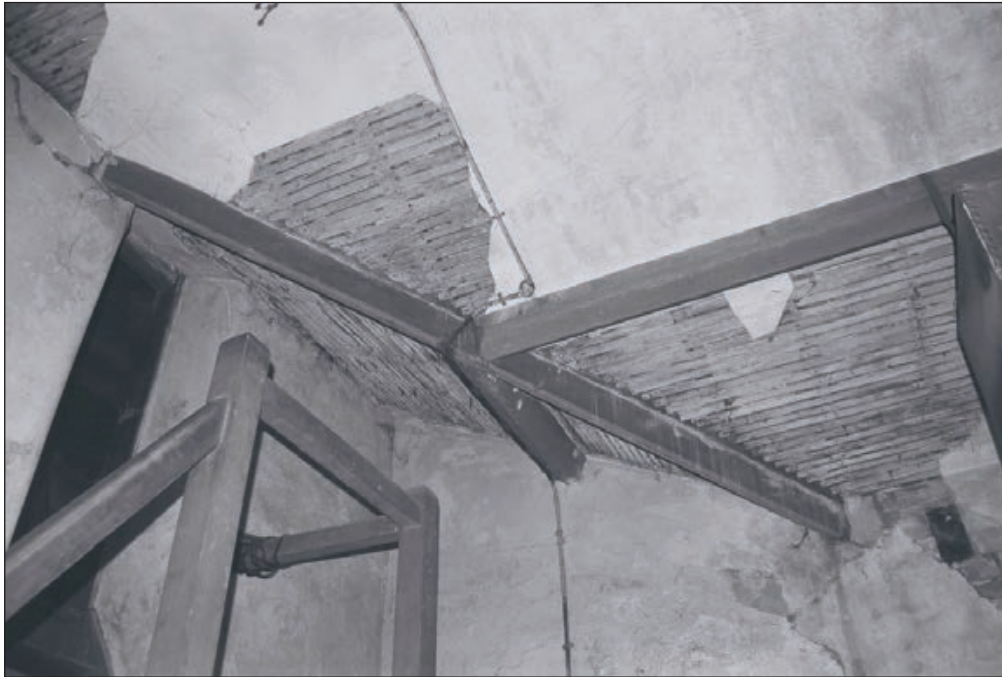
Plate 202: View of ceiling/roof structure of F12, Central Entranceway of the North Range (Film 42.01)
