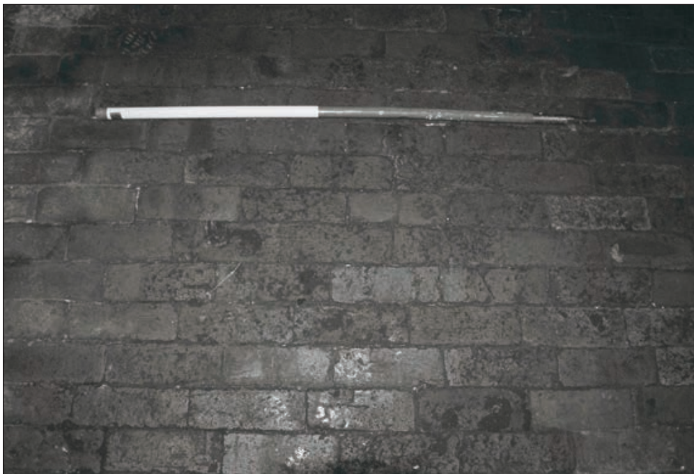
Plate 43: Detail of brick floor surface, room G1, East Side of the North Range (Film 14.05)
