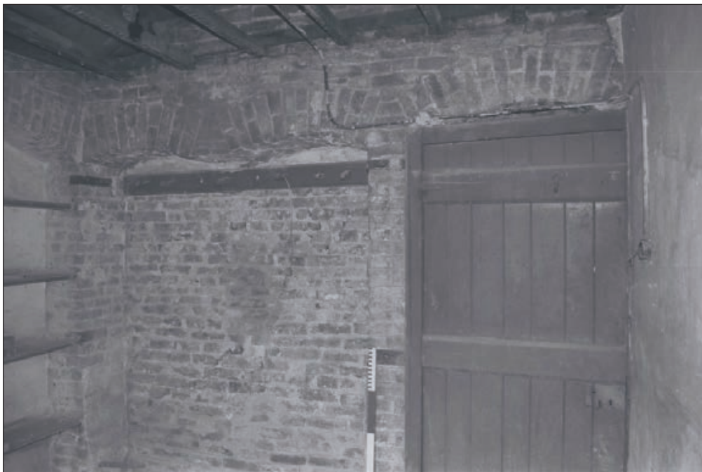
Plate 215: General view of F12 after removal of bathroom fittings and plaster from walls, Central Entranceway of the North Range (Film 76.25)
