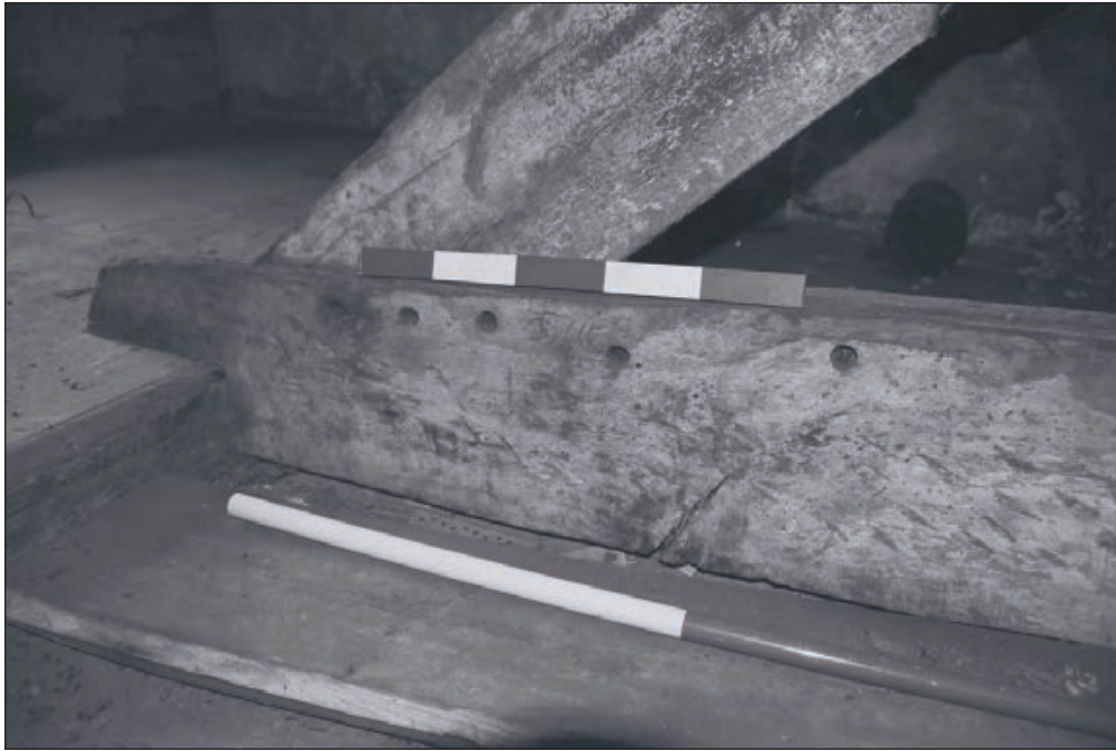
Plate 177: Detail of pegged trusses of timber clock tower structure, F10, Central Entranceway of the North Range (Film 42.15)
