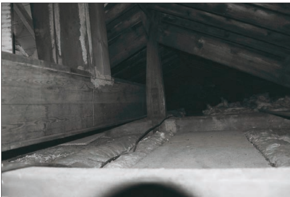
Plate 144: View of King-Post roof trusses and vents within roof void above room F2, East Side of the North Range (Film 16.13)
