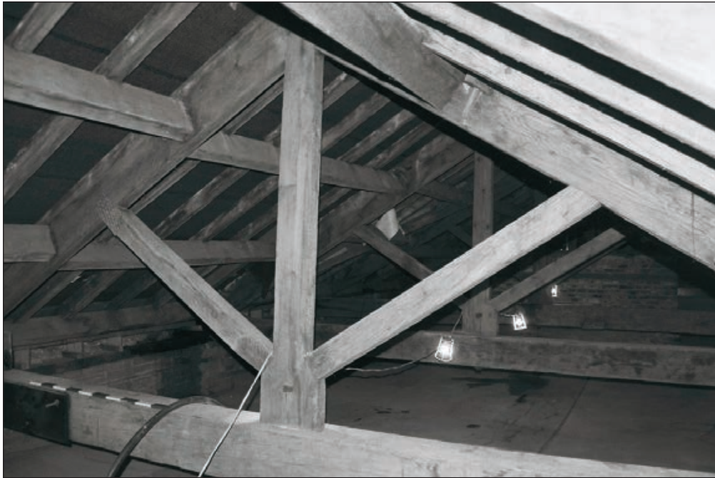
Plate 327: General view of Roof Void 8, showing timber King-Post truss, West Range - OB.98 (Film 71.10)
