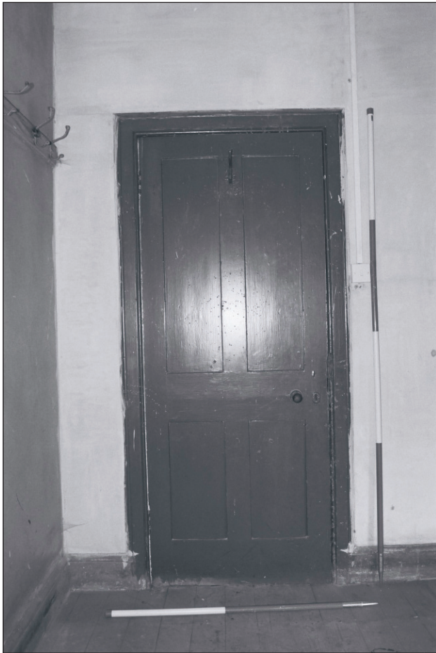
Plate 228: Detail of door from corridor F14, north wall of room F15, West Side of the North Range (Film 25.19)
