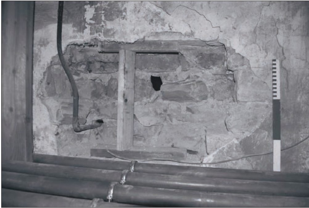
Plate 185: Detail of inserted opening within the east wall of F10, Central Entranceway of the North Range, showing exposed stone fabric of wall - OB. 20 (Film 51.30)
