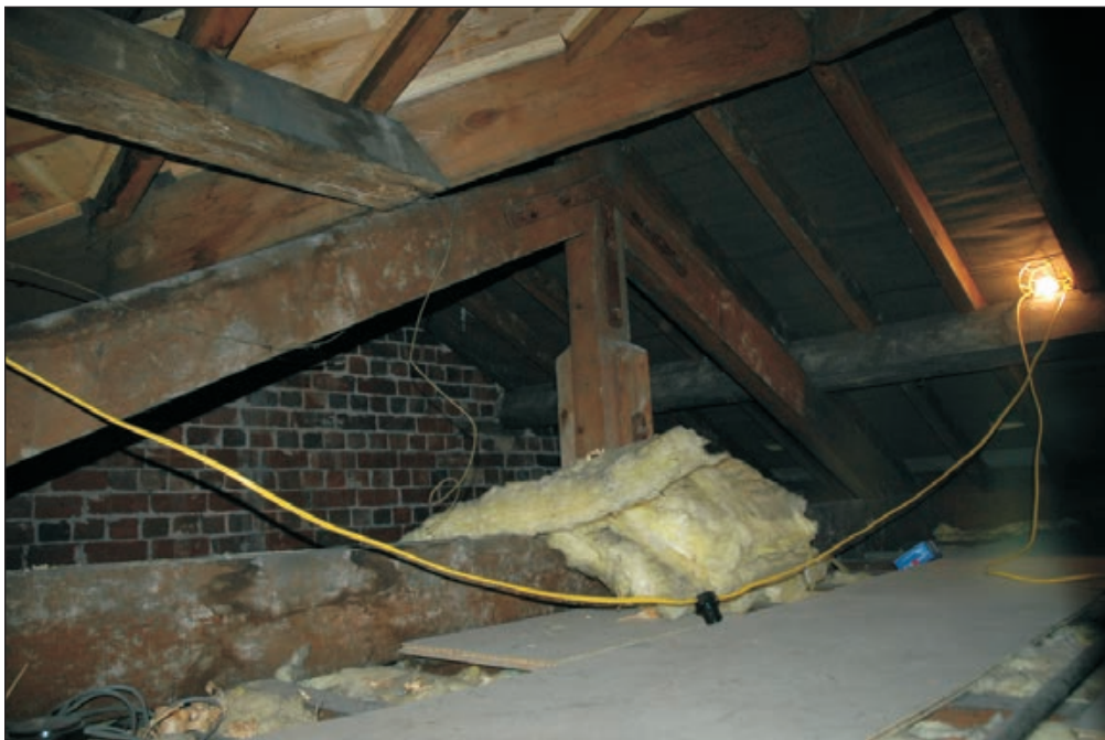
Plate 256: View of timber trusses, roof void above F21 and F22, West Side of the North Range (Film D. 18.02.10 7029)
