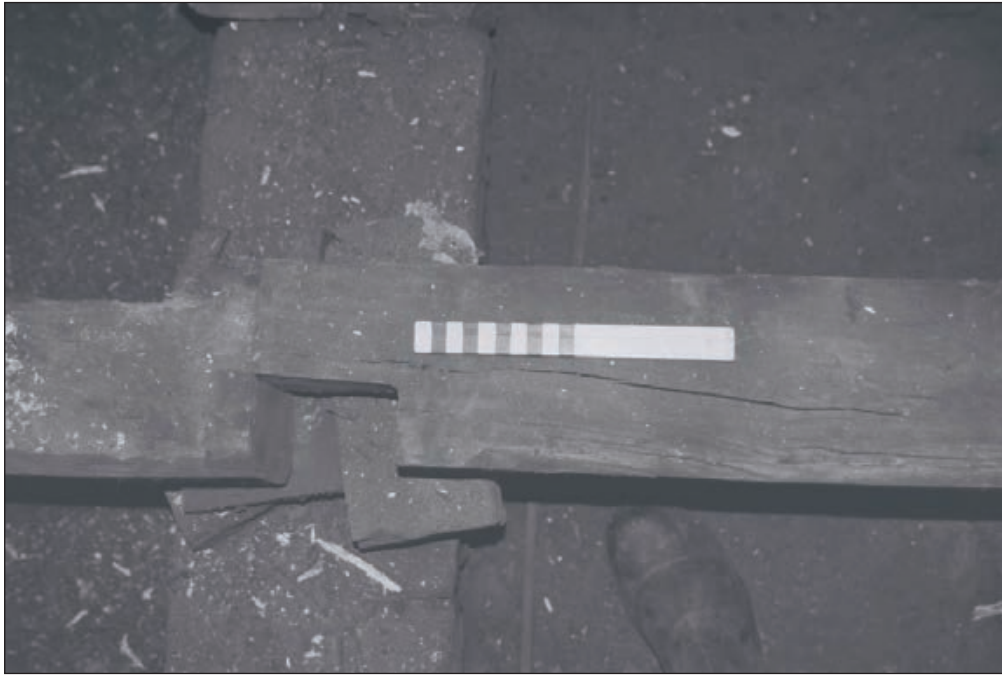
Plate 483: Detail of reused timber beam as floor joist, G47, South Range - Agent's House - OB.118, showing chamfer and stop (Film 75.10)
