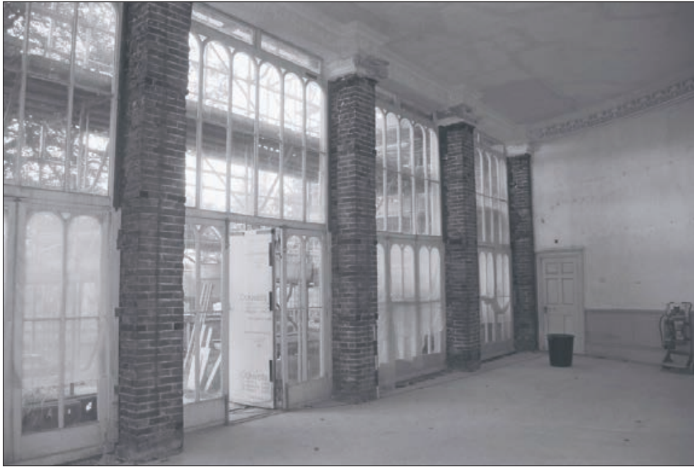
Plate 466: General view of G41, South Range, after removal of timber column surrounds - OB. 106 (Film 74.17)
