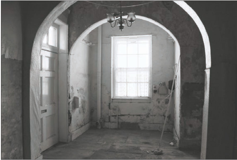
Plate 105: General view of rooms G10/11, Central Entranceway of the North Range, after removal of modern partitions (Film 52.15)
