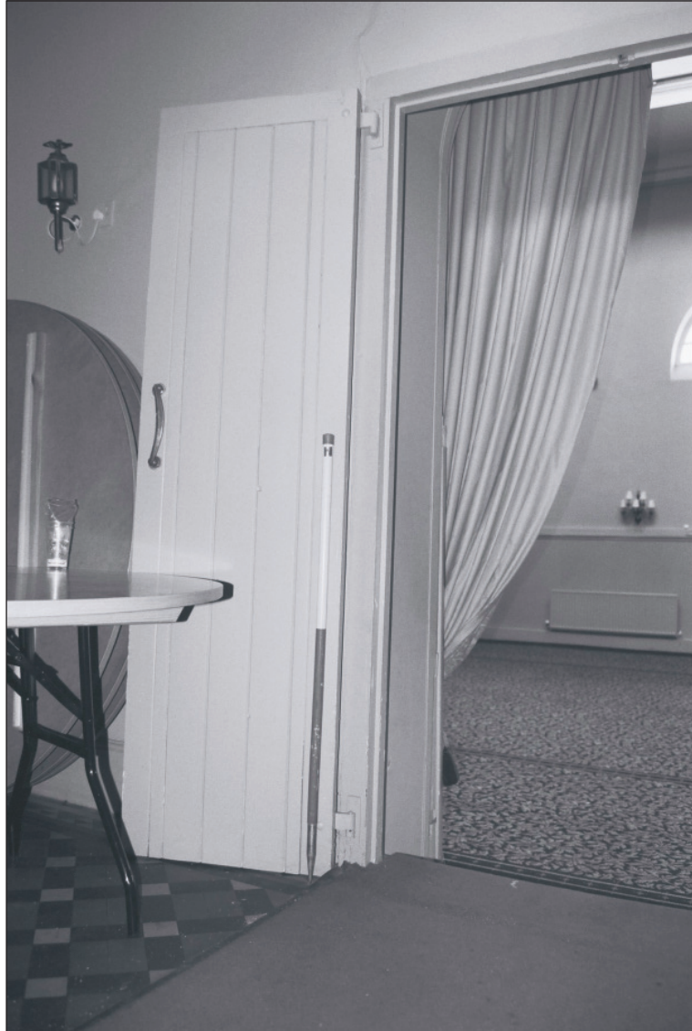
Plate 417: View of timber double door between G33 and G30, South Range (Film 24.10)
