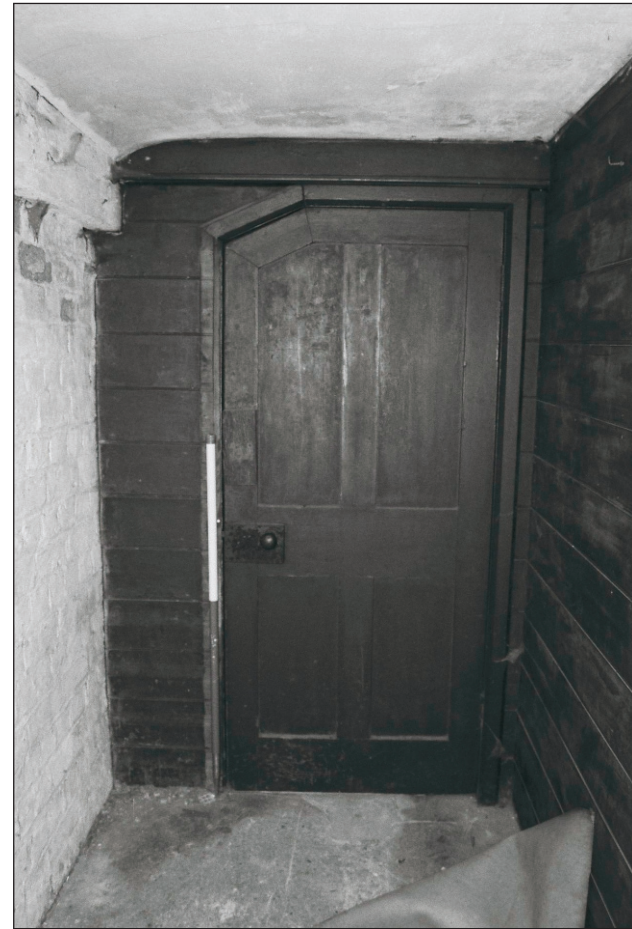
Plate 147: View of room F3 showing doorway to F2, East Side of the North Range (Film 15.36)
