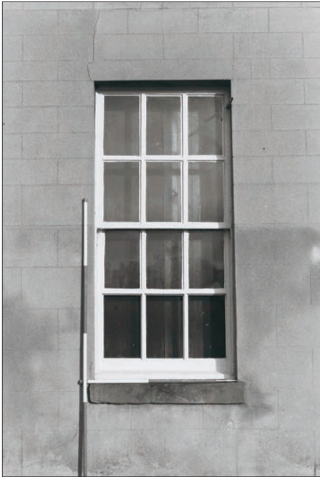
Plate 349: Detail of ground floor window, south elevation of the Riding House, South Range (Film 12.33)
