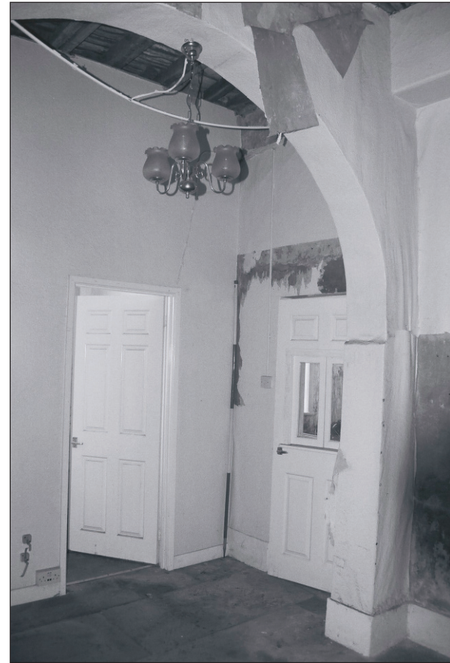
Plate 96: General view of room G10, Central Entranceway of the North Range, showing modern partition with G11 and doorway to G12 (Film 26.01)
