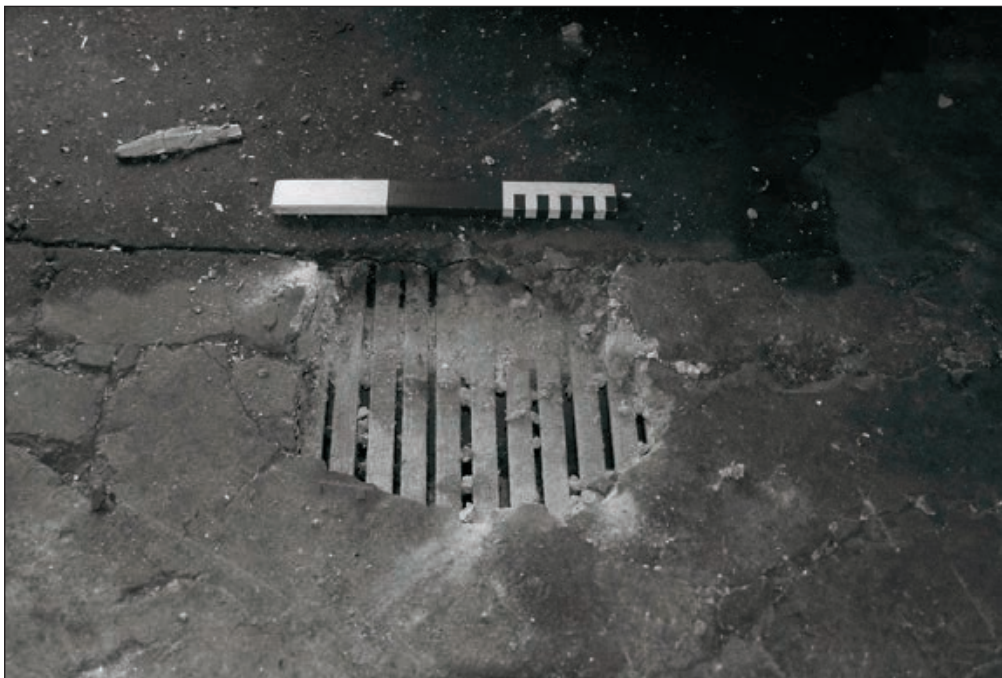
Plate 151: Detail of limeash floor on timber joists and laths, room F4, East Side of the North Range (Film 16.06)
