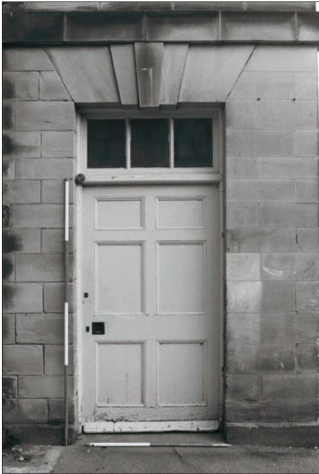
Plate 34: Detail of timber panelled doorway within the west elevation of the projecting section of the west end of the North Range (Film 20.26)
