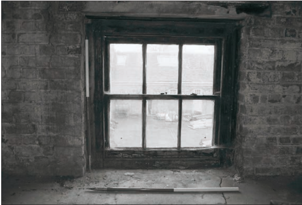
Plate 140: Detail of window, room F2, East Side of the North Range (Film 16.19)
