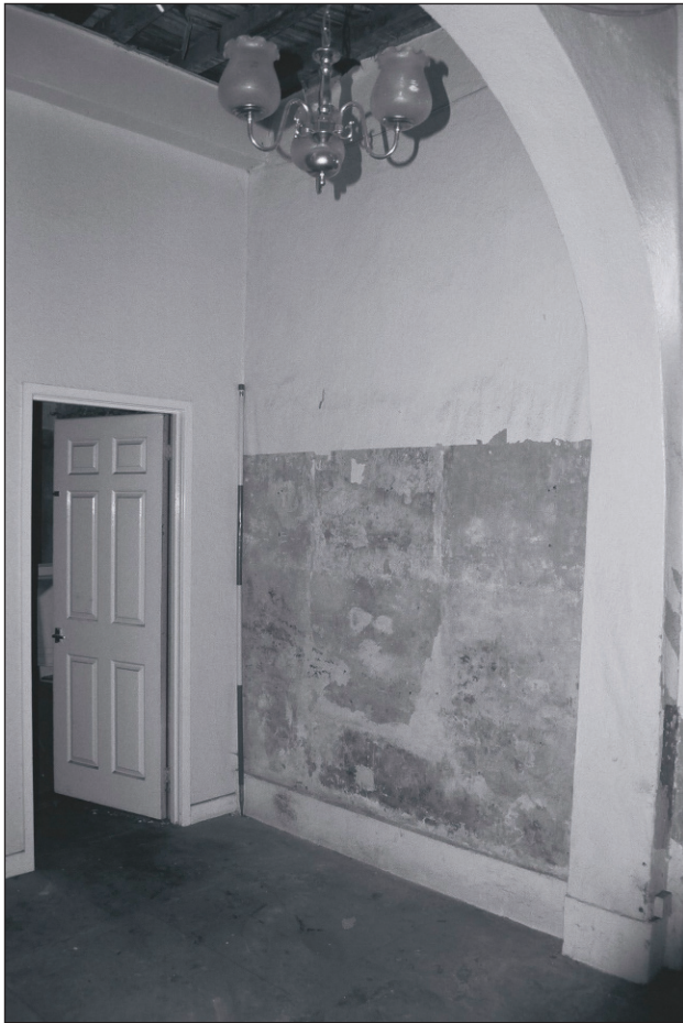
Plate 95: General view of room G10 showing modern partition with G9, Central Entranceway of the North Range (Film 26.04)
