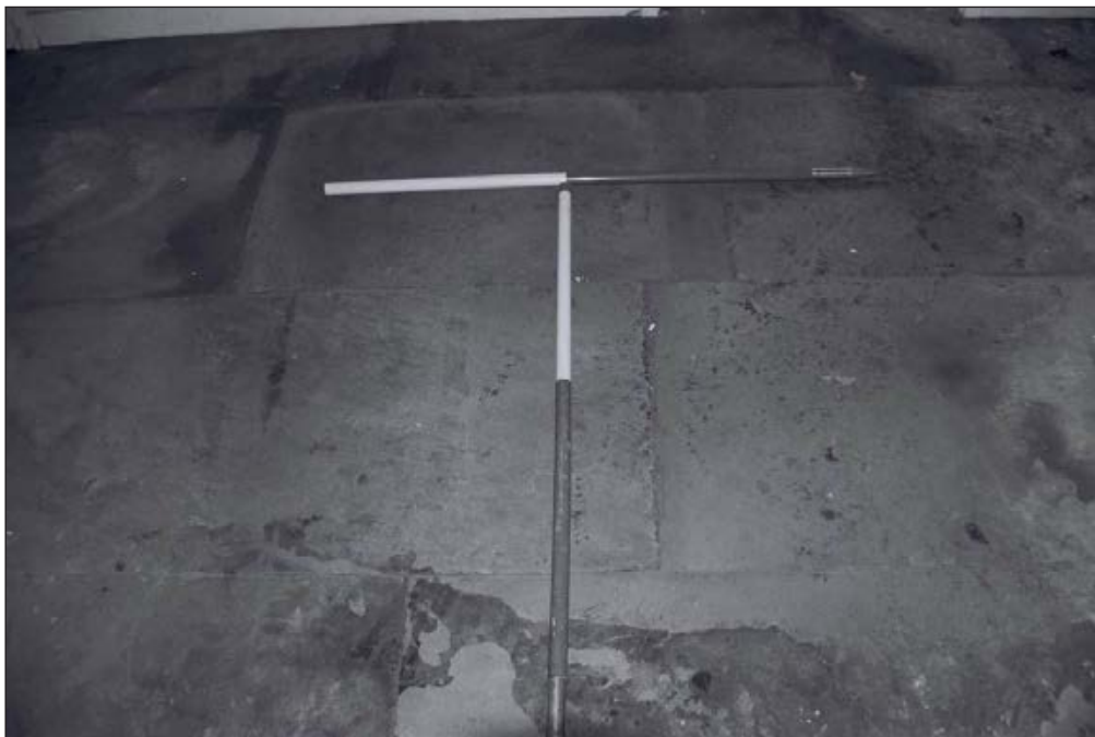
Plate 102: Detail of stone flag floor, room G9, Central Entranceway of the North Range (Film 41.35)
