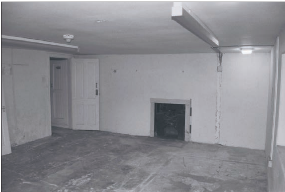
Plate 386: General view of F28, South Range, after removal of modern partitions and fittings - OB. 126 (Film 77.03)
