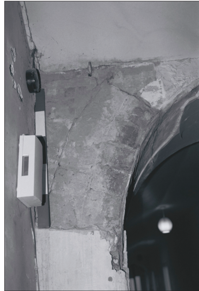
Plate 254: Detail of removed plaster exposing brickwork beneath, corridor F21, West Side of the North Range (Film 25.01)
