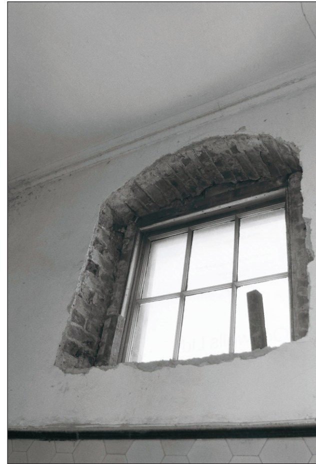
Plate 588: Detail of opened up former blind windows, east wall of G56, East Range (Film 52.25)
