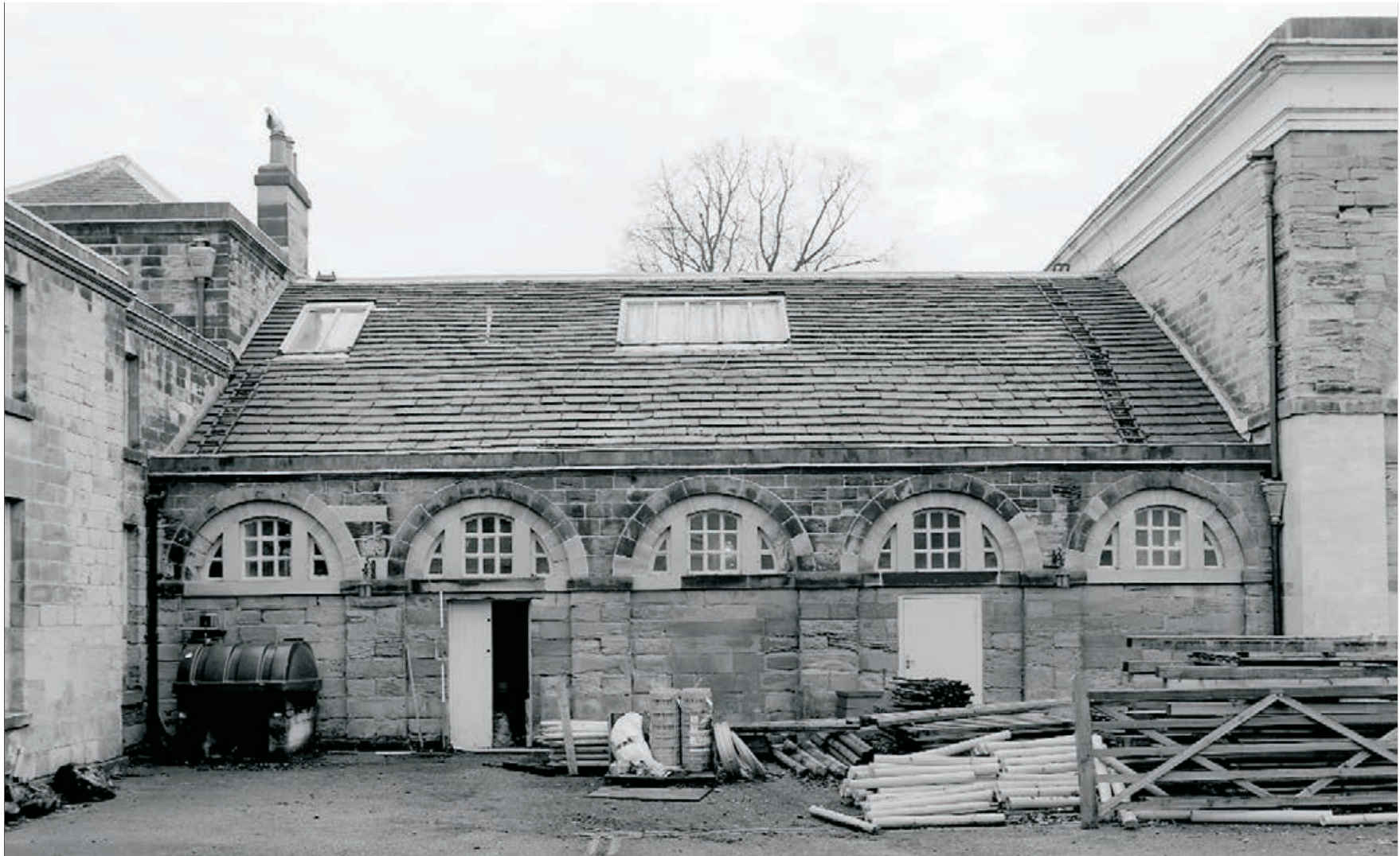
Plate 364: General view of the north courtyard elevation of the former corridor to the rear of the Greenhouse, South Range (Film 18.06)
