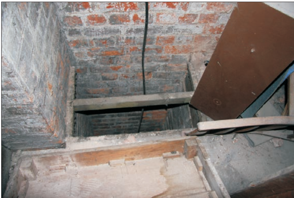
Plate 139: View of chute in floor of room F2, East Side of the North Range, leading to G1 below - OB. 59 (Film D. 14.10.10 1640)
