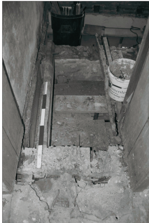
Plate 219: General view of exposed timber floor joists, room F13, Central Entranceway of the North Range, after removal of limeash (Film 69.35)
