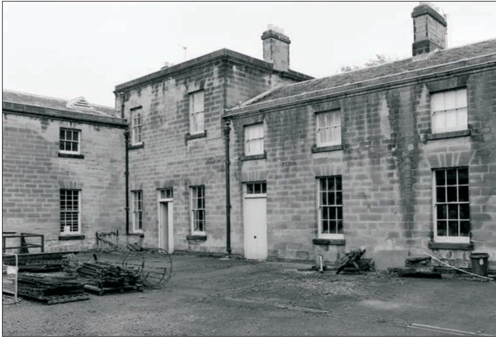
Plate 569: View of the north end of the west courtyard elevation of the Range, showing junction with the North Range, looking northeast (Film 17.09)
