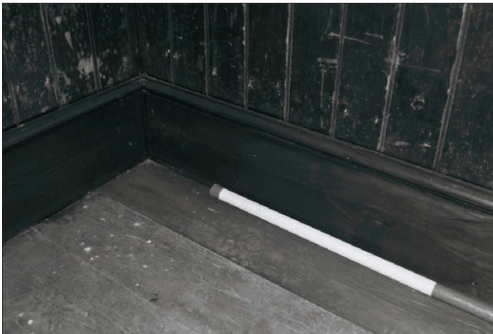
Plate 79: Detail of timber floor boards, skirting boards, match boarding, room G4, 'Tack Room', Central Entranceway of the North Range (Film 15.24)
