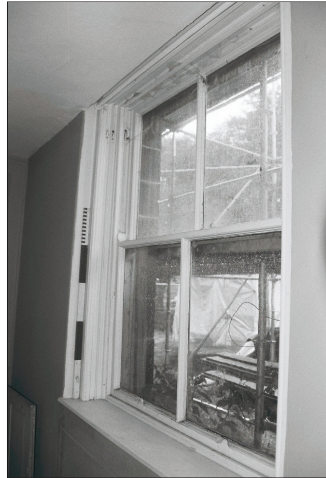
Plate 506: Detail of sash window with former lifting shutter, G43, South Range, Agent's House (Film 65.23)
