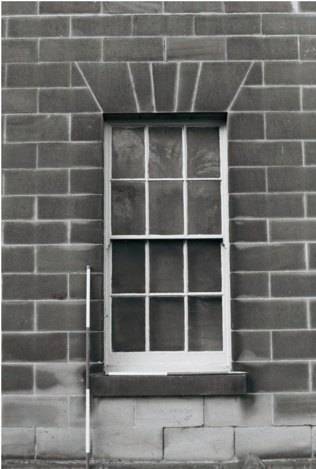
Plate 567: Detail of a 1905 blind window at the north end of the east elevation of the East Range (Film 11. 26)
