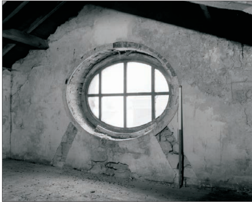
Plate 169: General view of the south side of F10, Central Entranceway of the North Range, showing oeil-de-boeuf window (Film 33.01)
