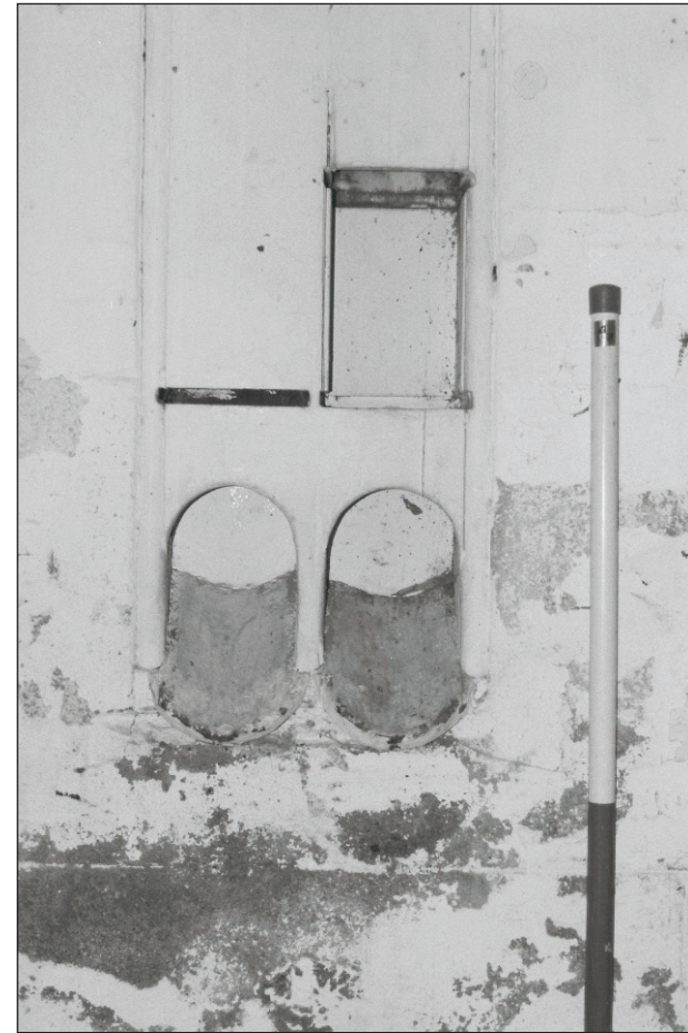
Plate 61: Detail of grain chutes from hay loft above, south wall of room G2, East Side of the North Range (Film 14.33)
