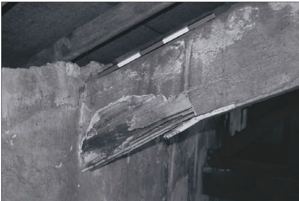
Plate 180: Detail of original phase 2 timber truss with lath and plaster covering, F10, Central Entranceway of the North Range (Film 42.23)
