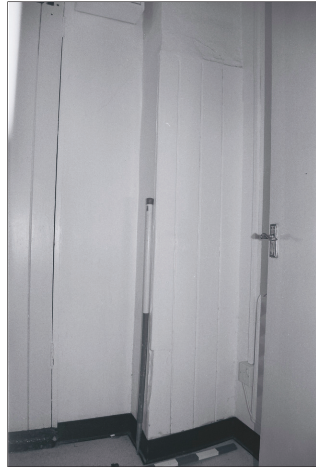
Plate 443: Detail of original tongue and groove match boarding on south wall of G38, South Range (Film 24.29)
