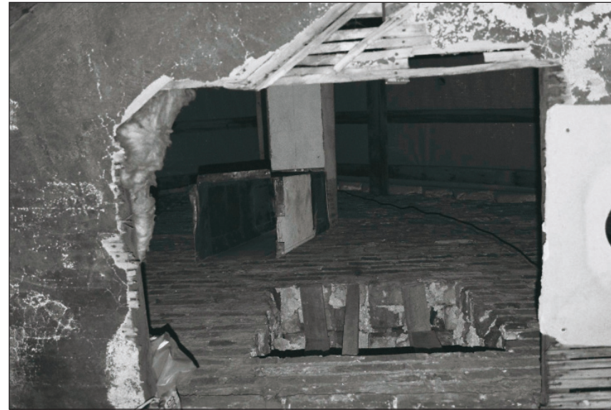
Plate 474: Detail of ceiling construction and inserted opening within west wall, roof void above G36, South Range (Film 13.24)
