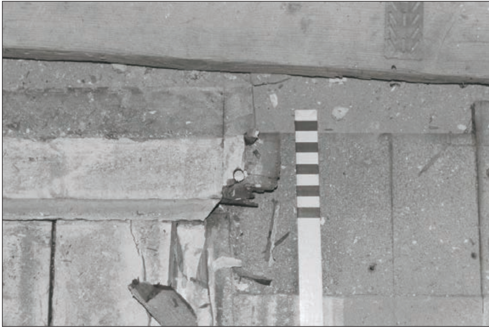
Plate 470: Detail of timber pegged joints of removed column panelling, G41, South Range - OB. 106 (Film 73.30)
