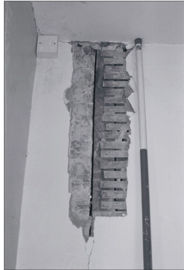
Plate 223: Detail of exposed join in brick and stud wall, south wall of corridor F14, West Side of the North Range (Film 25.30)
