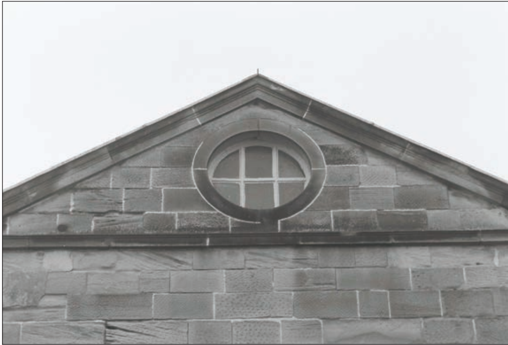
Plate 272: Detail of the oeil-de-boeuf window within the pedimented entrance of the east facing courtyard elevation of the West Range (Film 20.13)
