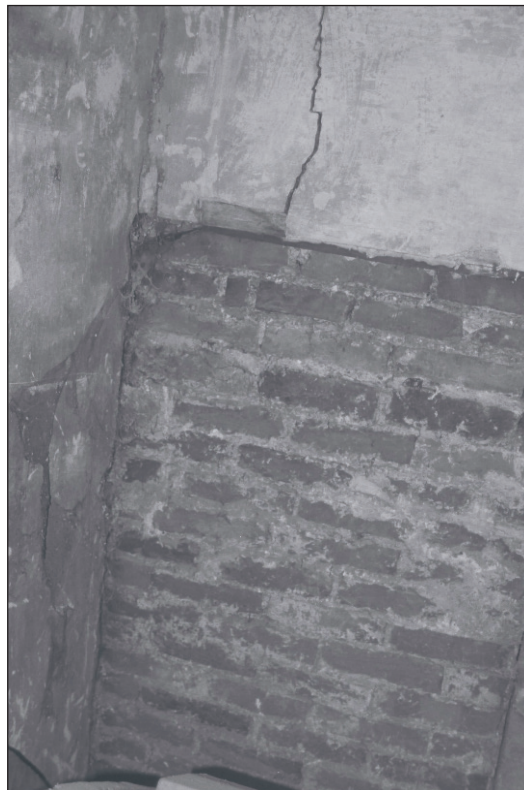
Plate 168: View of blocked doorway with F8 in east wall of F10b, Central Entranceway of the North Range - OB. 87 (Film 75.35)
