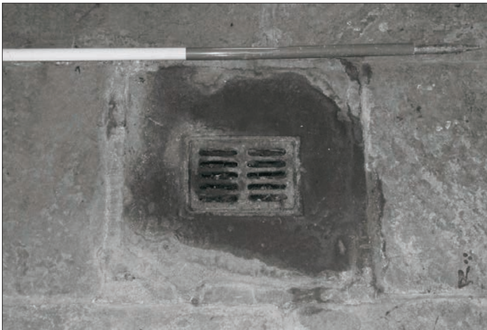
Plate 65: Detail of drain in floor of room G3, 'Wash Room', East Side of the North Range (Film 15.07)
