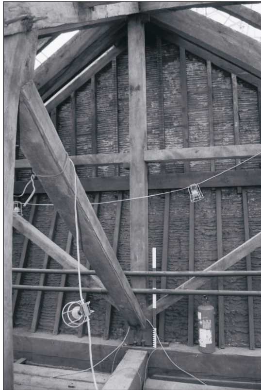
Plate 415: View of original hipped truss, roof structure of the Riding House above G30, South Range - OB. 67 (Film 55.35)
