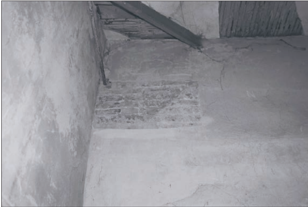
Plate 206: View of area of removed plaster exposing brick fabric, east wall of F12, Central Entranceway of the North Range - OB. 26 (Film 48.19)
