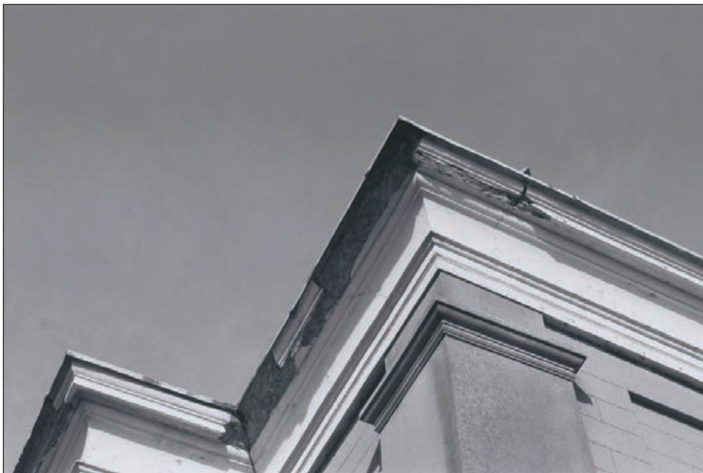
Plate 347: Detail of the cornice of the south elevation of the South Range - OB. 32 (Film 51.09)
