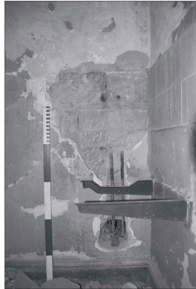
Plate 231: Detail southeast corner of room F15, West Side of the North Range, showing exposed stonework - OB. 30 (Film 51.24)
