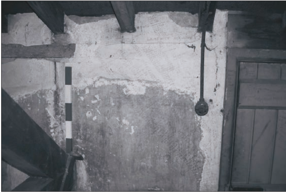
Plate 181: View of graffiti on west wall of F10, Central Entranceway of the North Range (Film 42.30)
