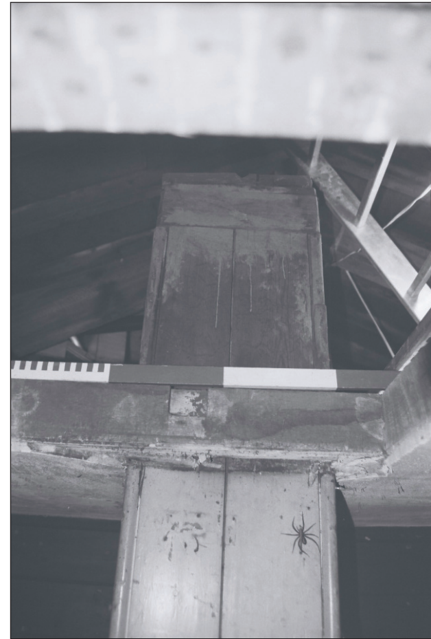
Plate 143: Detail of vent running into the roof void above F2, East Side of the North Range - also note lath and plaster ceiling - Observation 18 (Film 47.27)
