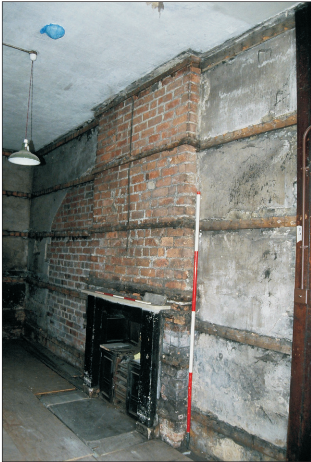
Plate 86: View of exposed east wall after removal of timber match boarding, room G4, 'Tack Room', Central Entranceway of the North Range, showing later brick blocking - OB. 71 & 75 (Film C.S. 32)
