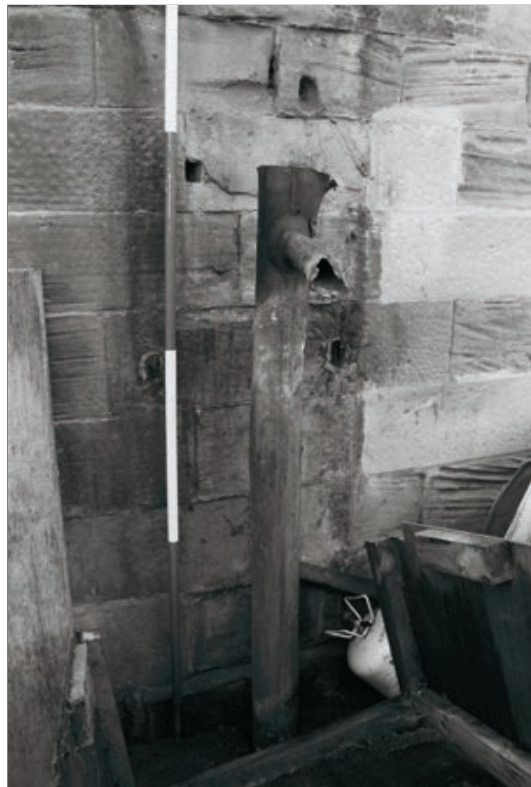
Plate 363: Detail of the pipework of the Adam designed water pump against the north elevation of the Riding House, South Range (Film 20.10)
