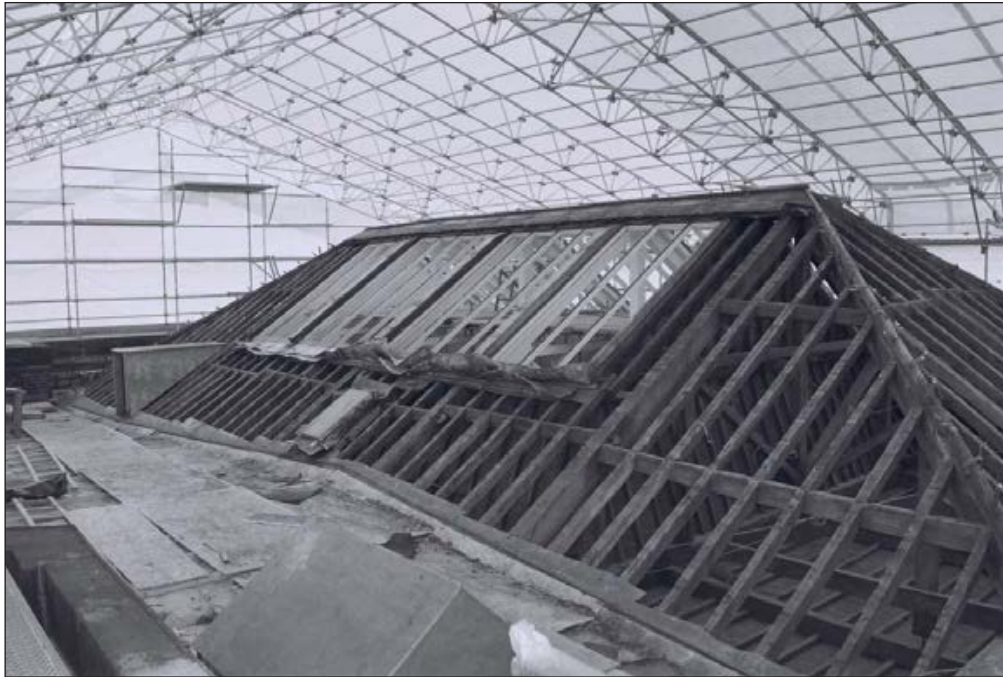
Plate 413: View of exposed timber roof structure of the Riding House above G30, South Range - OB. 67 (Film 54.05)
