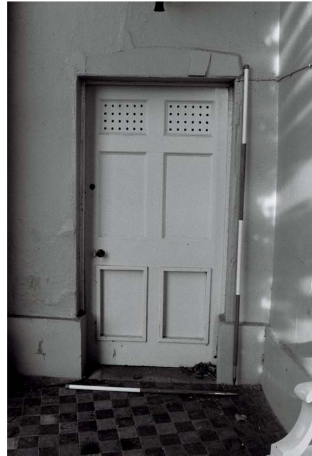
Plate 352: Detail of ground floor doorway within the west wall of the Riding House loggia (G34), south elevation of the South Range (Film 13.03)
