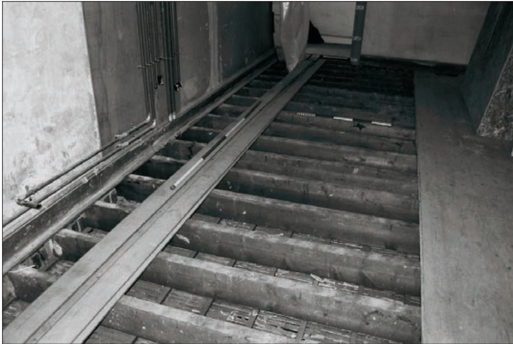
Plate 232: View of exposed timber floor structure, room F15, West Side of the North Range - OB. 43 (Film 53.17)
