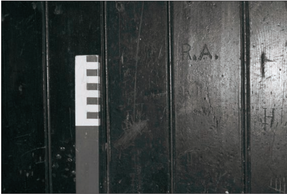
Plate 78: Detail of graffiti carved into tongue and groove match boarding on wall of room G4, 'Tack Room', Central Entranceway of the North Range (Film 15.28)
