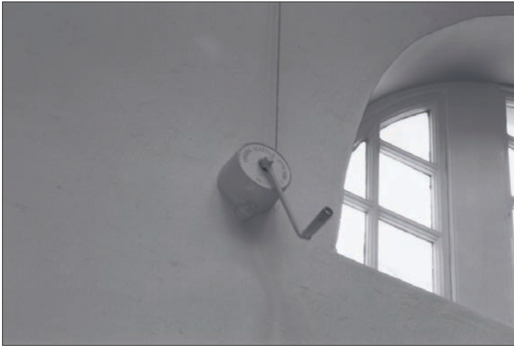
Plate 404: Detail of pulley mechanism for opening inserted skylights within roof, G30, South Range (Film 24.16)
