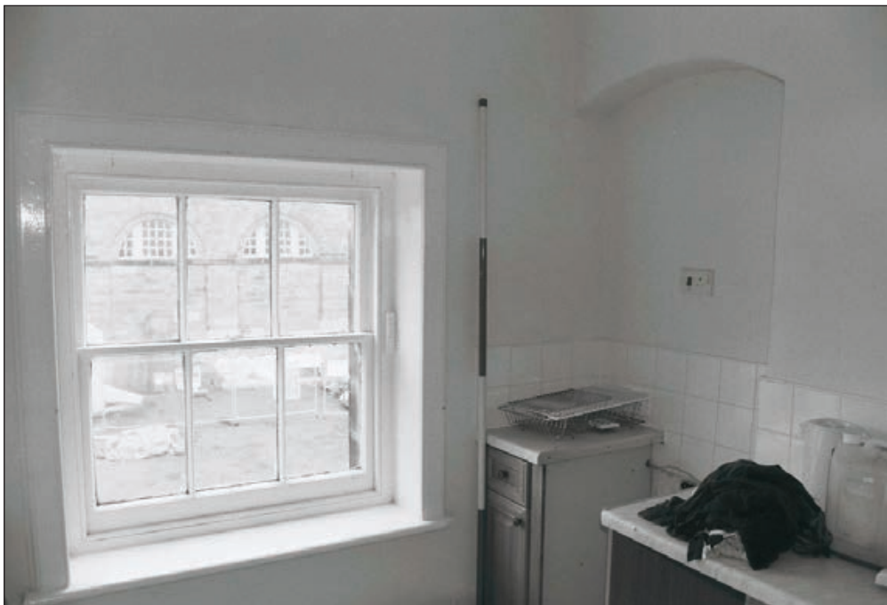
Plate 159: View of the southwest corner of room F9, Central Entranceway of the North Range, showing window and blocked doorway (Film 15.29)
