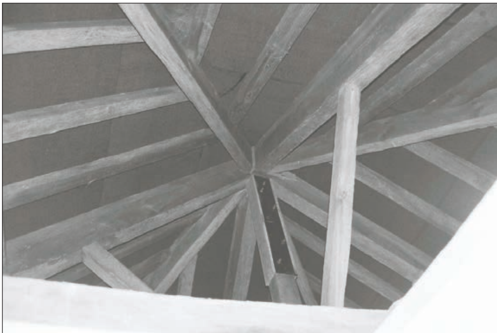
Plate 537: View of timber roof trusses above F35 and F36, South Range - Agent's House (Film 72.23)
