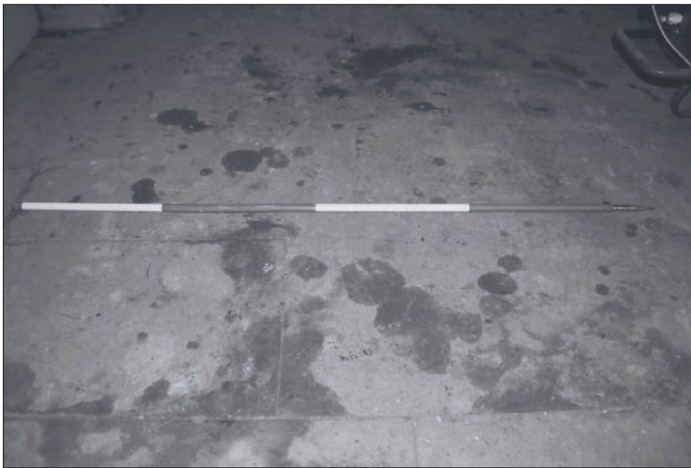
Plate 123: Detail of stone flag floor of room G15, West Side of the North Range (Film 26.13)
