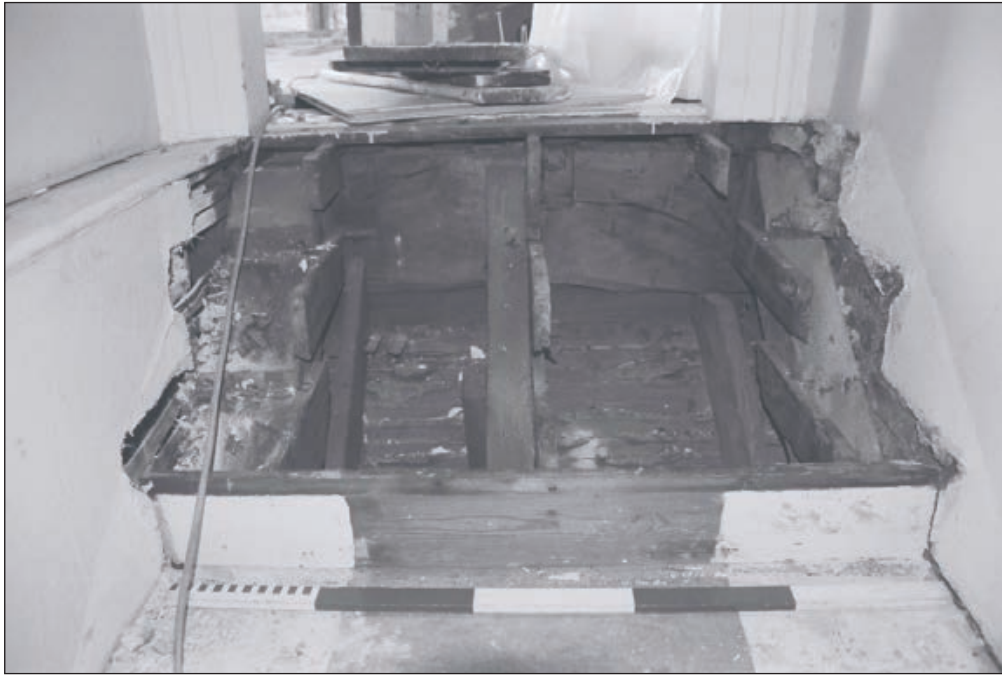
Plate 526: View of lifted stair treads exposing inserted staircase construction, F37, South Range - Agent's House - OB. 78 (Film 68.05)
