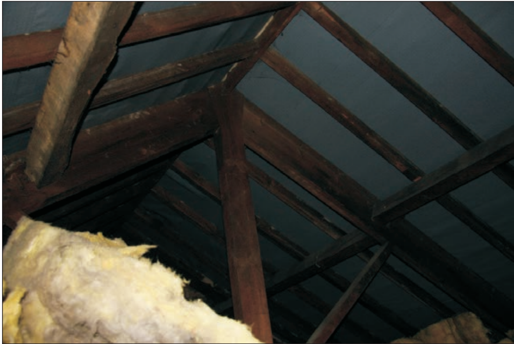
Plate 552: View of timber King-Post truss in roof above F38, South Range - Agent's House (Film D. 21.10.10 1860)
