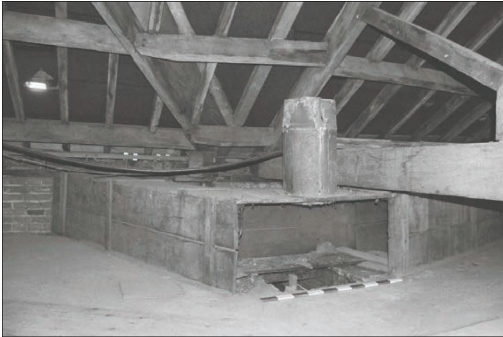
Plate 329: View of inserted timber vent within Roof Void 8, West Range - OB.98 (Film 71.07)
