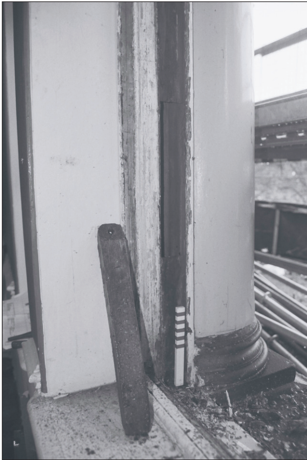
Plate 485: Detail of timber sash window with weight, G47, South Range - Agent's House - OB. 118 (Film 75.05)
