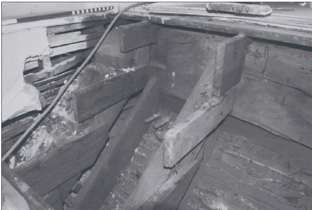
Plate 527: View of lifted stair treads exposing inserted staircase construction, F37, South Range - Agent's House - OB. 78 (Film 68.01)
