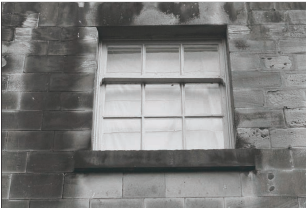
Plate 370: Detail of a first floor window at the south end of the west courtyard elevation of the South/East Range (Agent's House) (Film 20.04)
