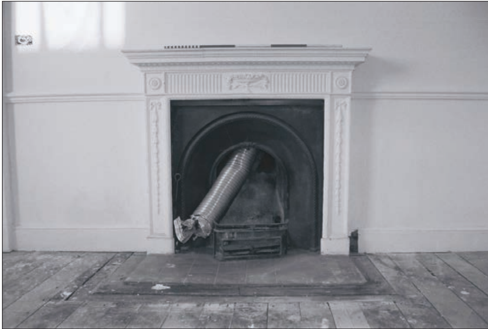
Plate 479: Detail of fireplace, west wall of G47, South Range - Agent's House (Film 77.35)
