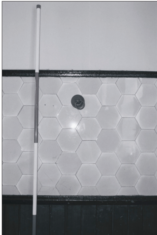
Plate 294: Detail of tiling and tether hook, south wall of loose box, G22, West Range (Film 23.23)
