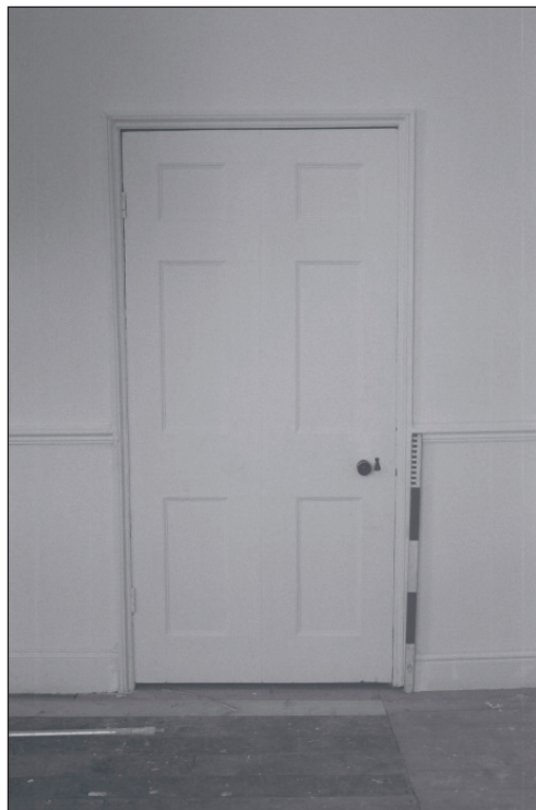
Plate 480: Detail of doorway to corridor G48, north wall of G47, South Range - Agent's House (Film 77.30)
