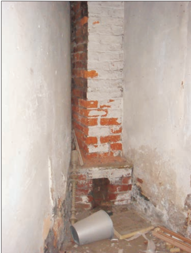
Plate 475: View of inserted brick flue within the south corner of G36, South Range - OB. 60 (Film D. 05.05.10 05166)
