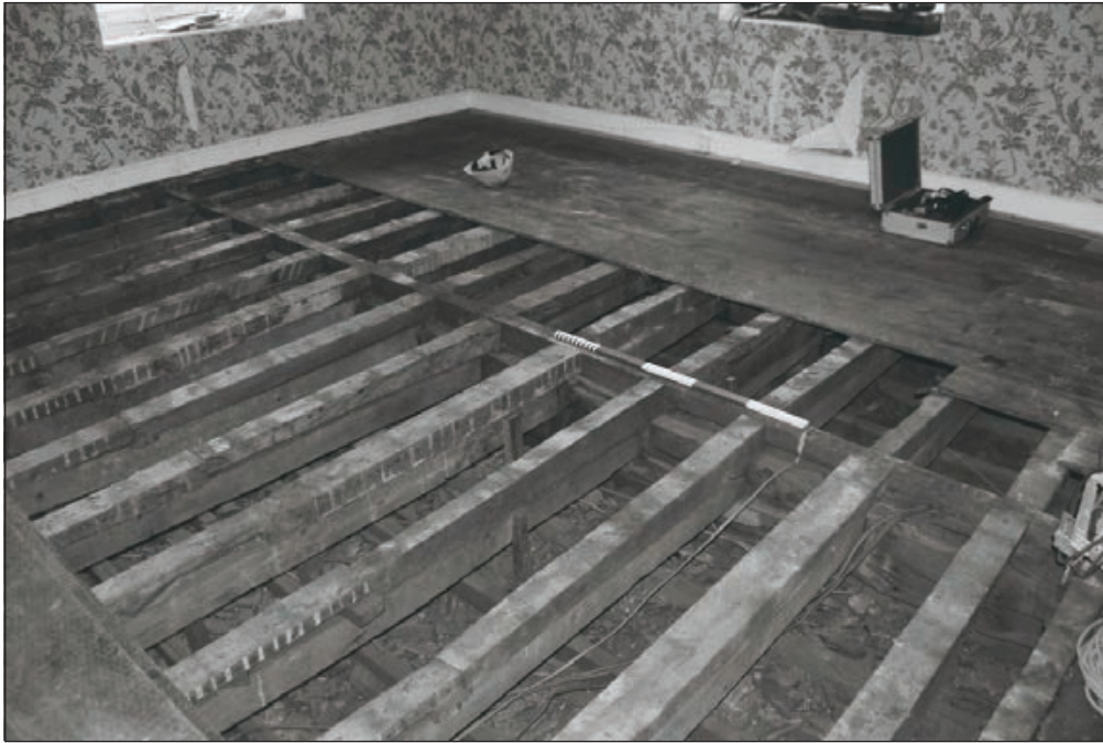
Plate 532: Detail of exposed timber floor and ceiling construction, F35, South Range - Agent's House - OB. 76 (Film 66.10)
