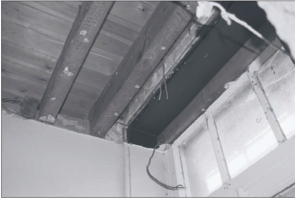
Plate 522: View of inserted modern joists for F41 above and position of removed inserted ceiling, G53, South Range - Agent's House (Film 46.05)
