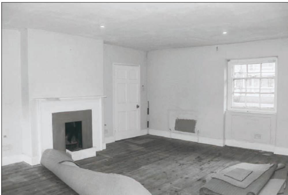
Plate 555: General view of F40, South Range - Agent's House - after removal of carpet (Film 66.26)
