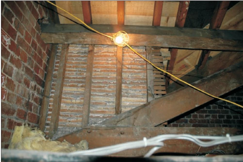
Plate 255: View of skylight construction, roof void above F21, West Side of the North Range (Film D. 18.02.10 7028)
