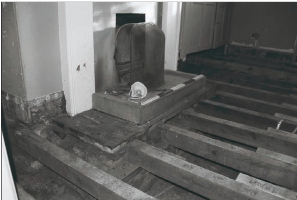
Plate 508: View of exposed timber joists and floor structure of G49, South Range - Agent's House - OB. 86 (Film 69.09)
