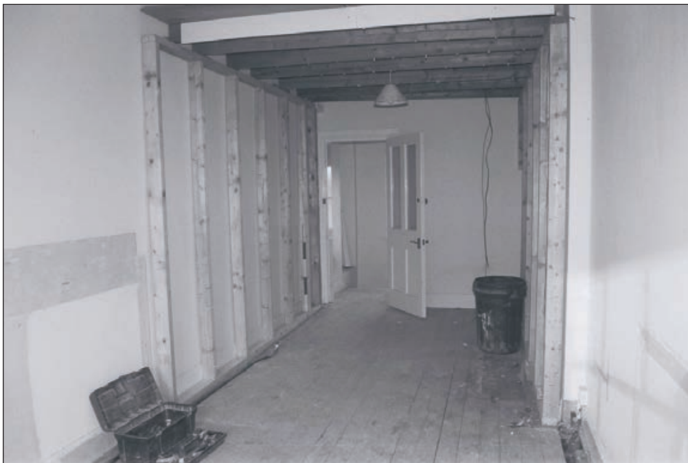
Plate 161: General view of room F9, Central Entranceway of the North Range after the removal of modern partitions etc. - OB. 122 - showing timber boarded floor and blocked fireplace (Film 77.12)
