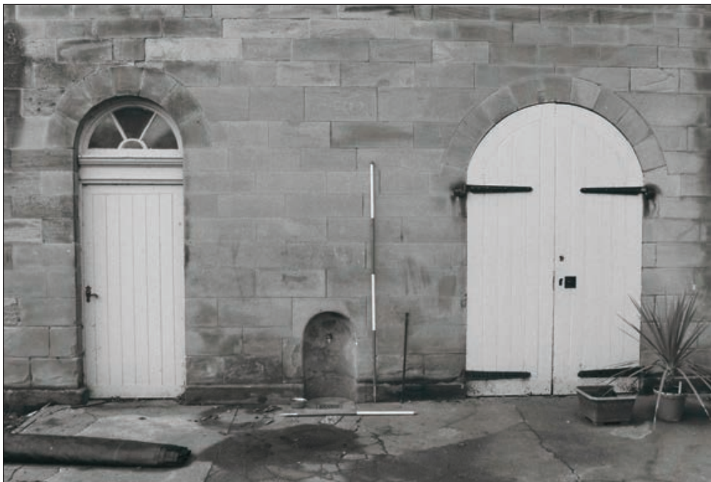
Plate 271: Detail of ground floor doorways at the north end of the east facing courtyard elevation of the West Range (Film 20.19)
