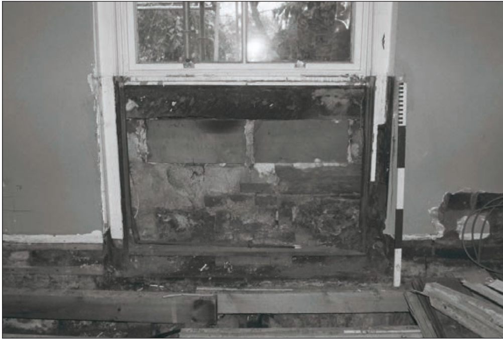
Plate 507: Detail of exposed former sash window shutter frame and east wall of G49, South Range - Agent's House - OB. 94 (Film 70.27)
