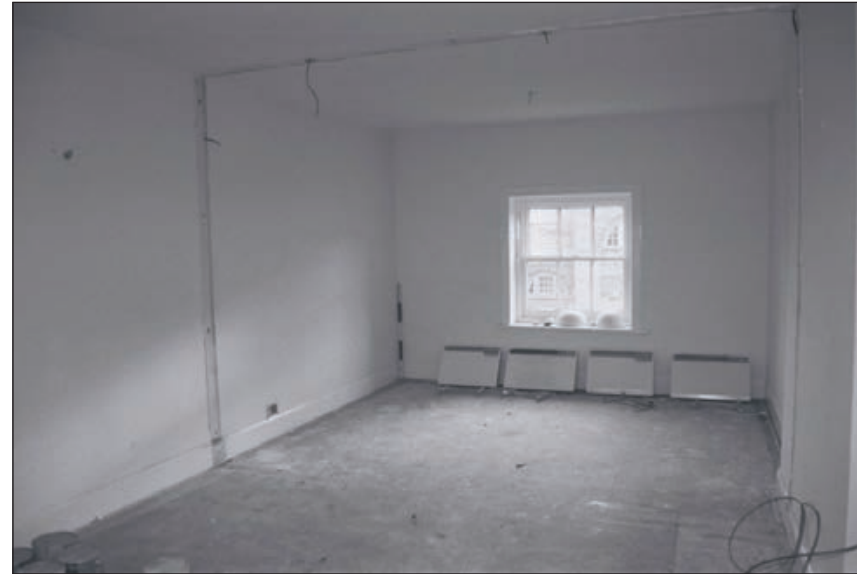
Plate 155: General view of rooms F6 and F7, East Side of the North Range, after removal of modern partitions - OB. 123 - showing limeash floor and blocked fireplace (Film 77.20)
