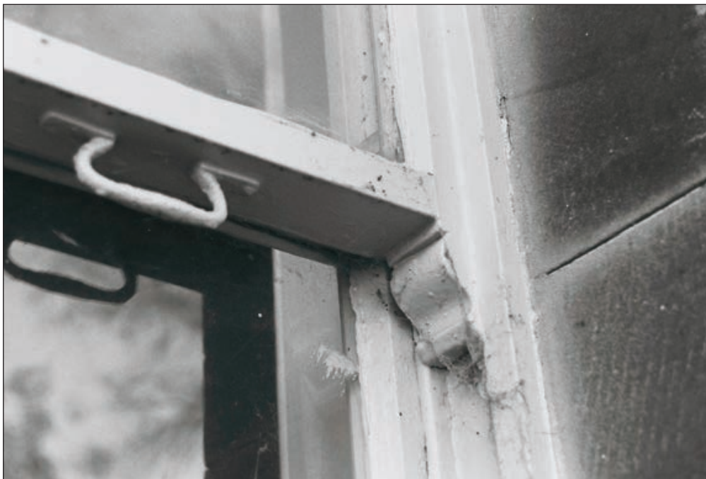
Plate 32: Detail of the moulded horn and attached handle of the ground floor timber sash window of the phase 7 west end of the north elevation of the North Range (Film 11.12)
