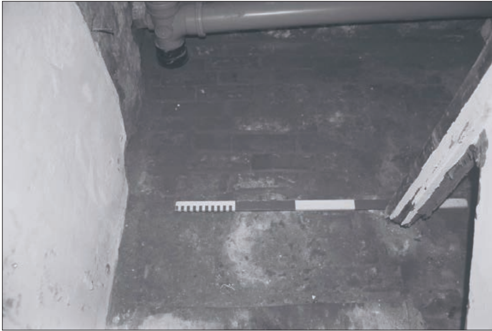
Plate 92: View of original brick floor of G5/6, Central Entranceway of the North Range - OB. 128 (Film 79.14)
