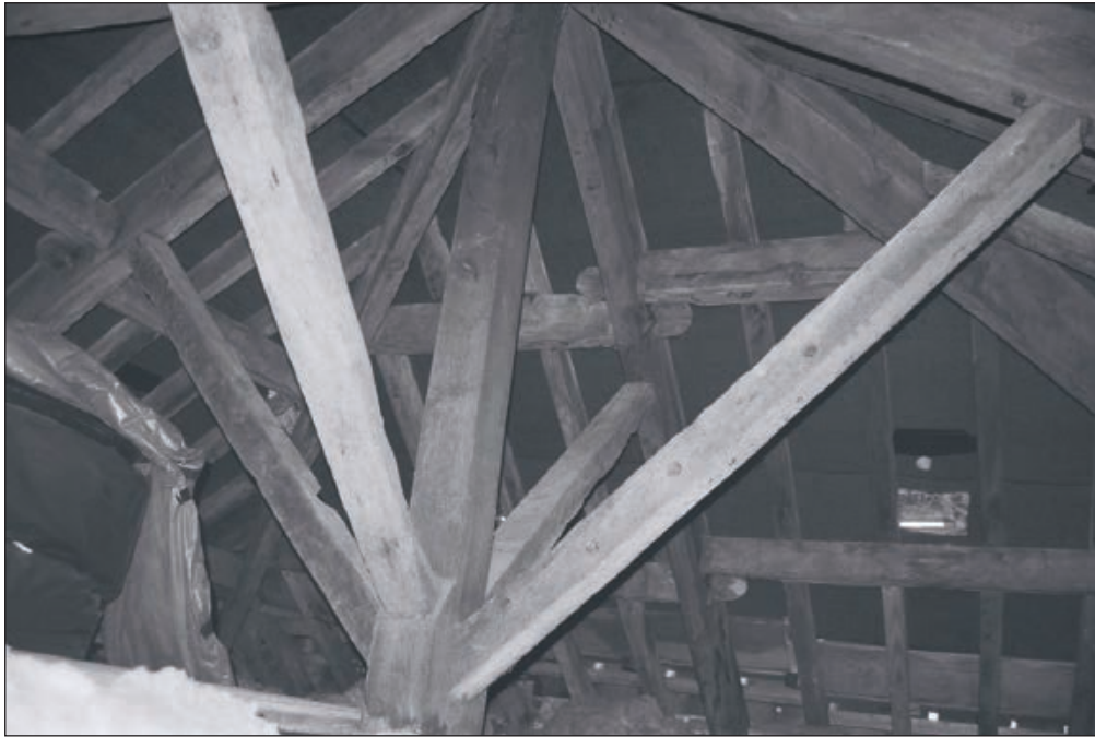
Plate 387: General view of timber trusses, roof void above F28, South Range, - OB. 127 (Film 78.26)
