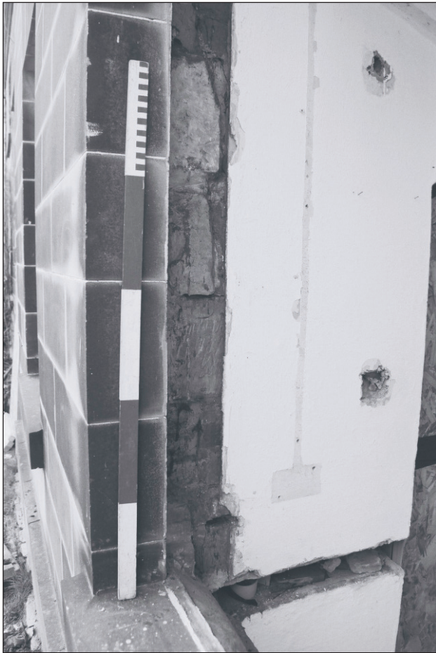
Plate 519: Detail of exposed wall fabric during insertion of door, G52, South Range - Agent's House - OB. 25 (Film 48.23)
