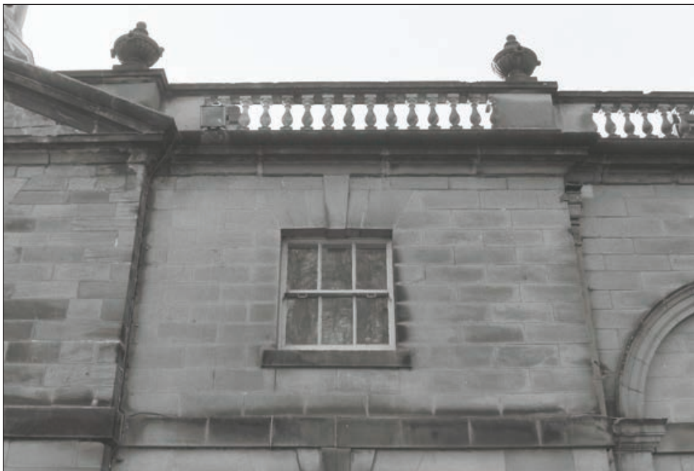
Plate 30: Detail of first floor window and upper balustrade, west end of the north elevation of the North Range, adjacent to the phase 2 Paine entranceway (Film 11.14)
