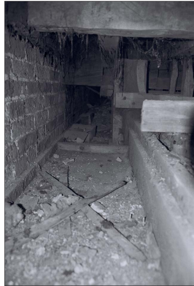
Plate 332: View below hatch in floor of Roof Void 8, West Range - OB. 98 - showing floor and ceiling construction and location of former grain chute (Film 78.20)
