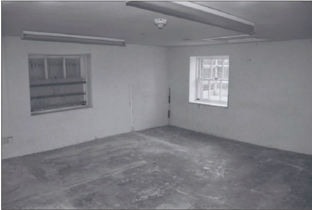
Plate 385: General view of F28, South Range, after removal of modern partitions and fittings - OB. 126 (Film 77.01)
