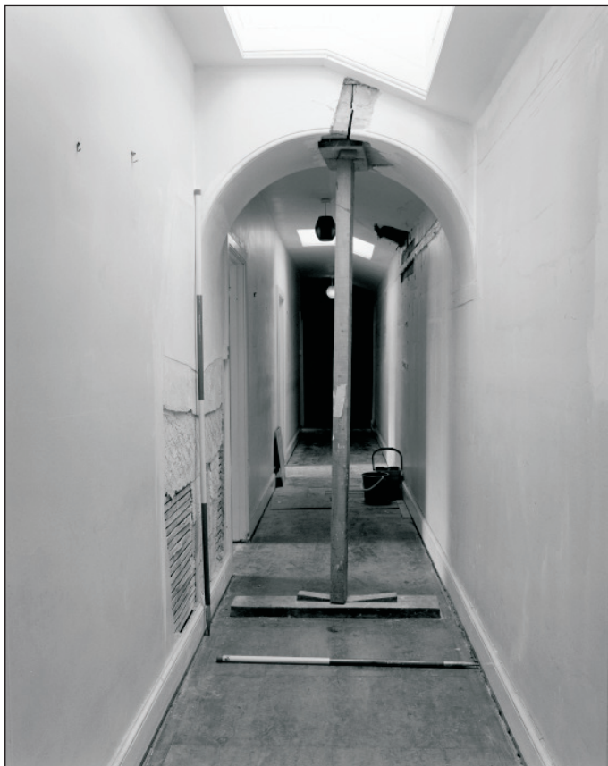
Plate 233: General view along corridor F18, West Side of the North Range (Film 33.09)
