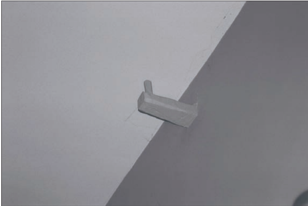
Plate 391: Detail of high timber bracket within east wall of G28, South Range (Film 24.01)
