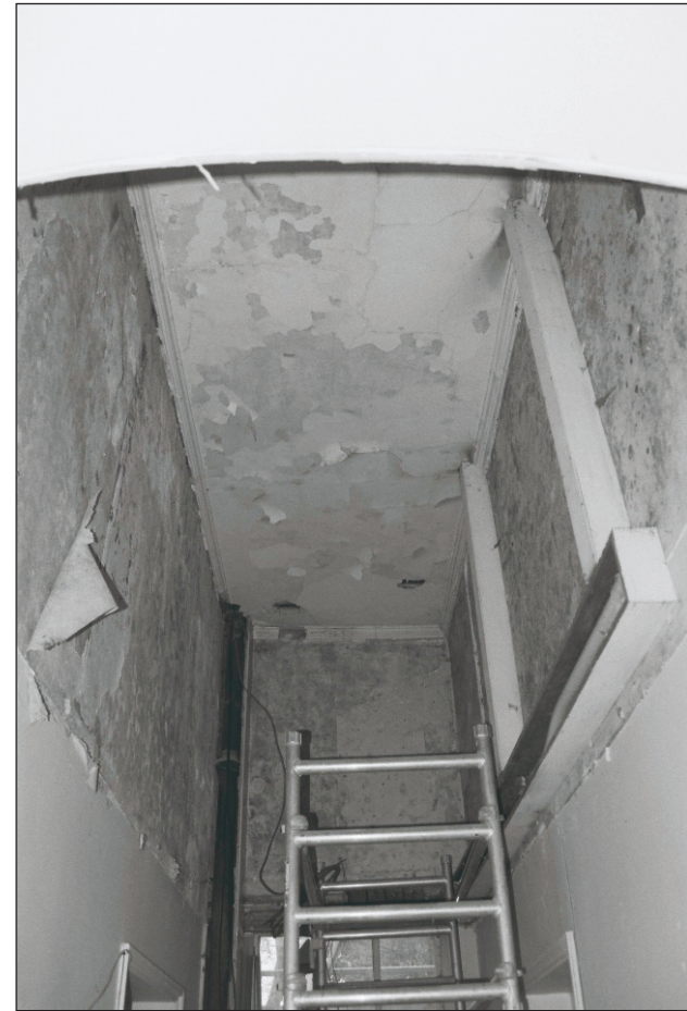
Plate 490: View of original ceiling after removal of modern insert, G48, South Range - Agents House (Film 70.33)
