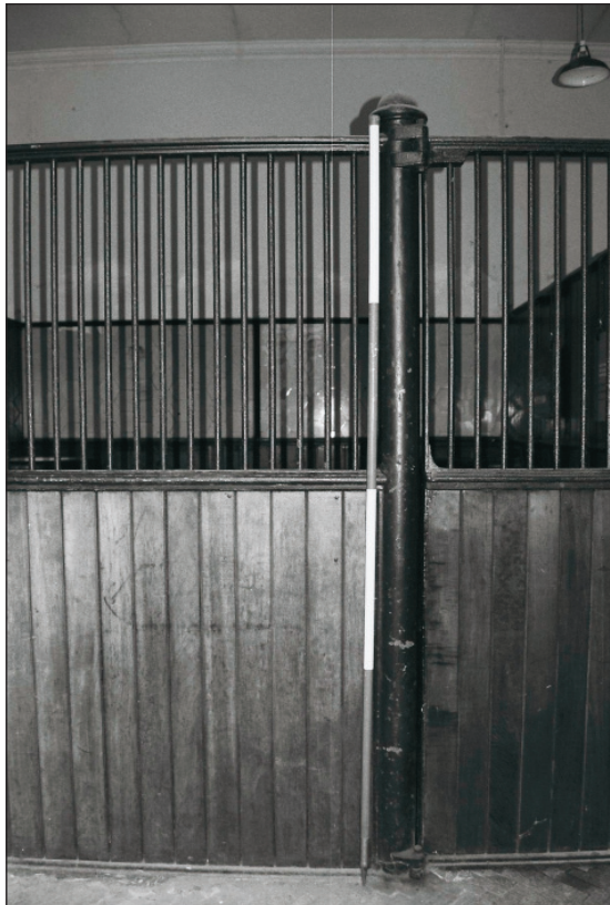
Plate 56: Detail of original cast iron column of loose boxes within room G2, East Side of the North Range (Film 14.29)
