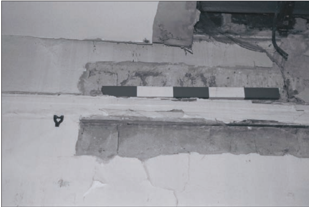
Plate 234: Detail of picture rail, north wall of corridor F18, West Side of the North Range (Film 25.13)
