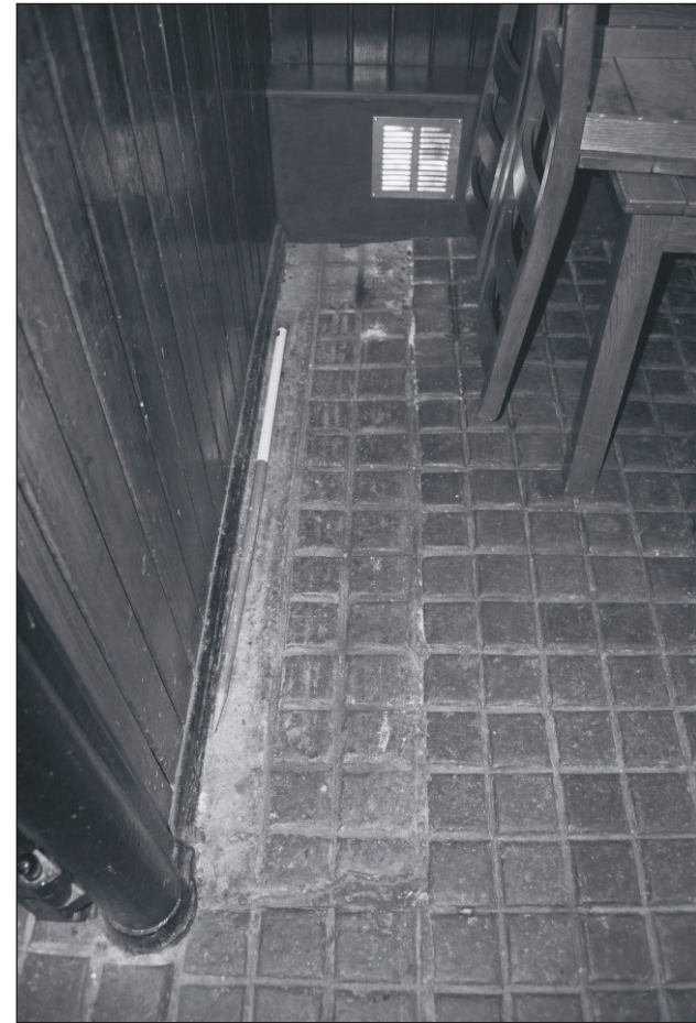
Plate 290: View of blocked stench trap surface drains in floor of loose box in G22, West Range (Film 23.19)
