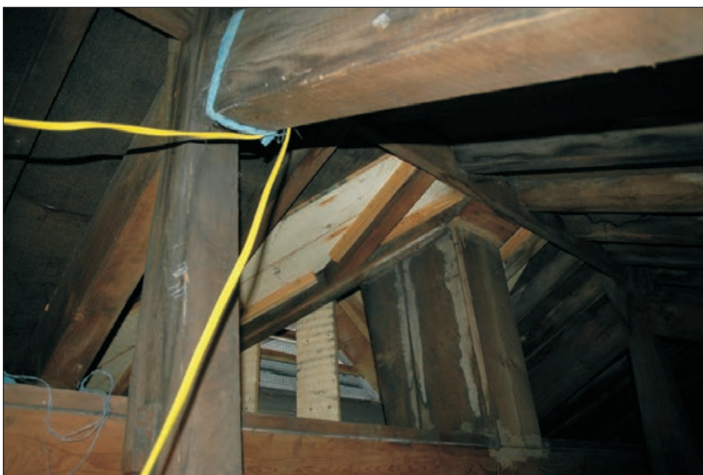
Plate 145: Detail of vent leading to raised roof vent in roof void above room F2, East Side of the North Range (Film D. 25.02.10 7533)
