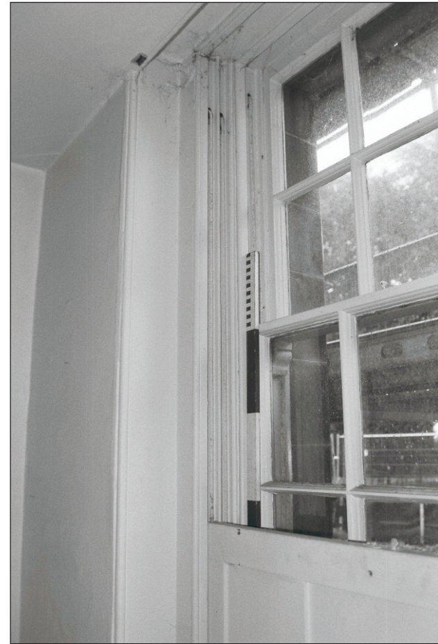
Plate 514: Detail of sash window with lifting shutter, G51, South Range - Agent's House (Film 65.27)
