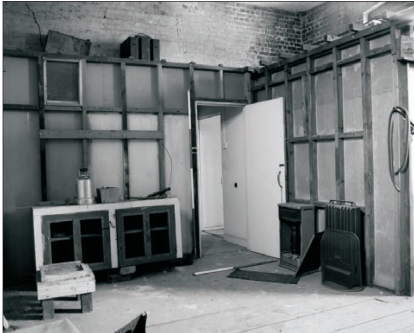
Plate 315: General view of inserted rooms F23-F26, within room F27 West Range (Film 36.04)
