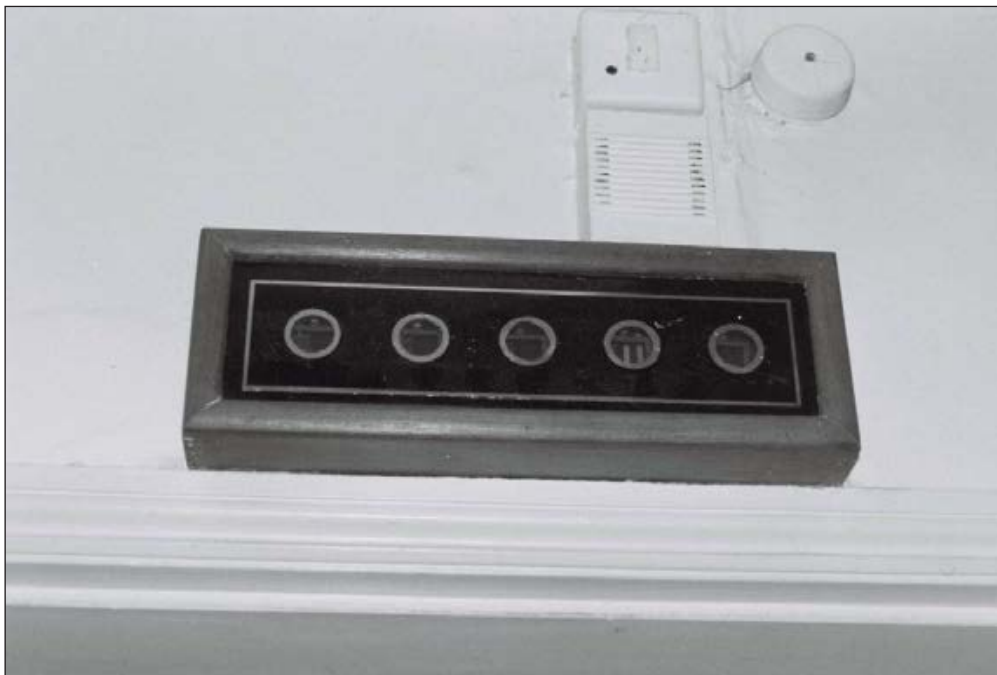
Plate 512: Detail of electric servant indicator board, above doorway with G50, G51 (Kitchen), South Range - Agent's House (Film 65.25)
