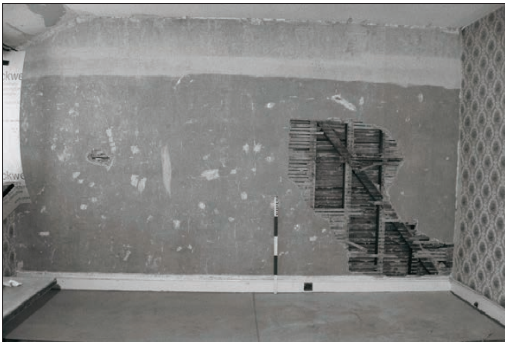
Plate 245: View of removed lath and plaster on west wall of room F19, West Side of the North Range - OB. 37 (Film 52.09)
