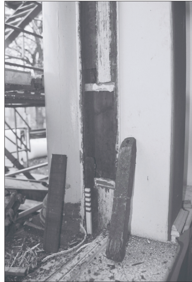
Plate 486: Detail of timber sash window with weight, G47, South Range - Agent's House - OB. 118 (Film 75.02)
