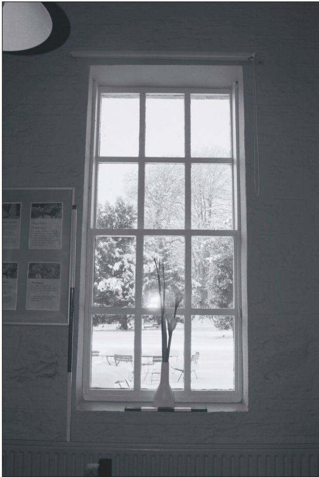
Plate 309: Detail of former blind window, west wall of G24, West Range (Film 22.06)
