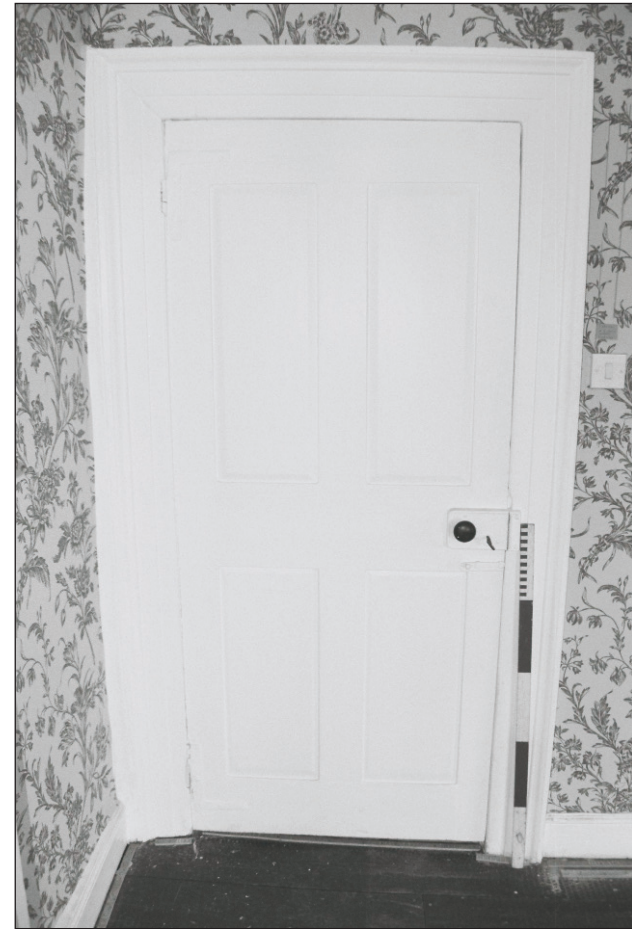
Plate 535: Detail of door, north wall of F35, South Range - Agent's House (Film 66.35)
