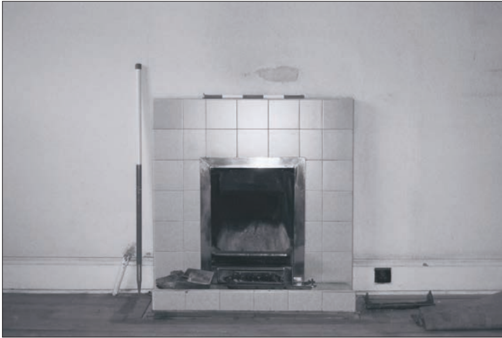
Plate 250: Detail of fireplace, room F20, West Side of the North Range (Film 25.06)
