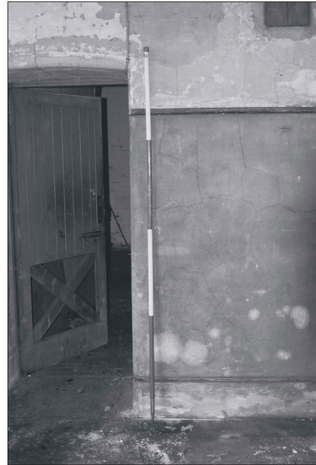
Plate 121: View of moulded plaster skirting and dado with paint scheme, G15, West Side of the North Range (Film 26.10)
