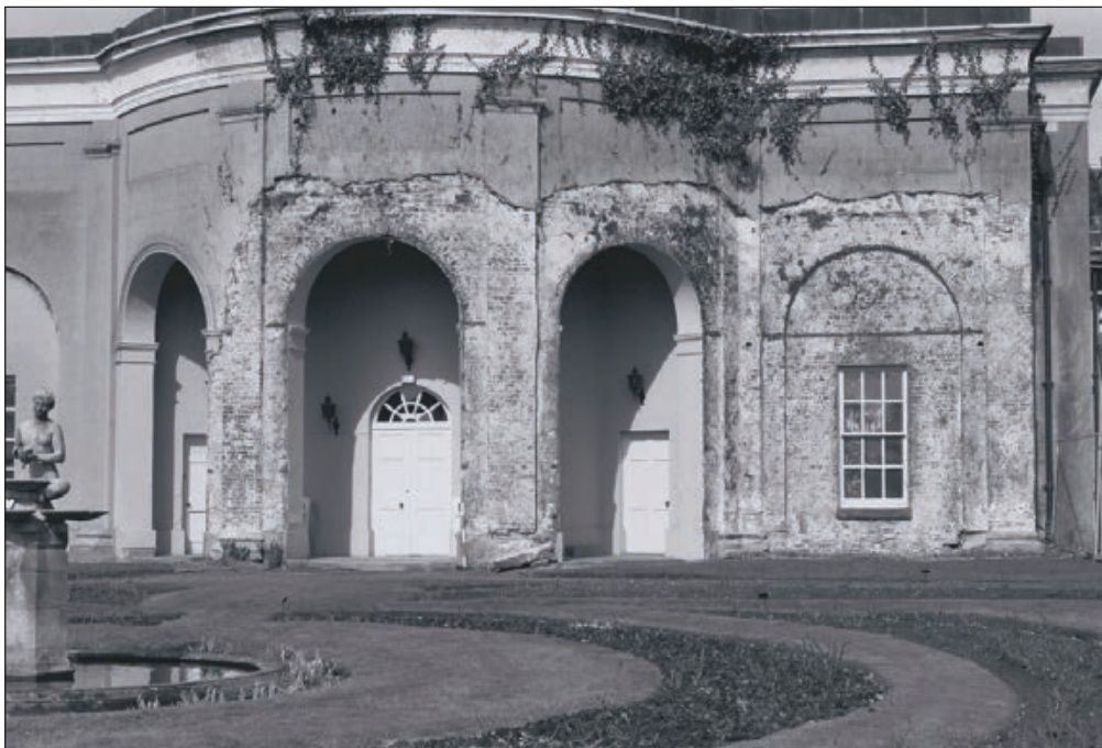
Plate 345: Detail of exposed brick fabric of the south elevation of the South Range - OB. 32 (Film 51.15)
