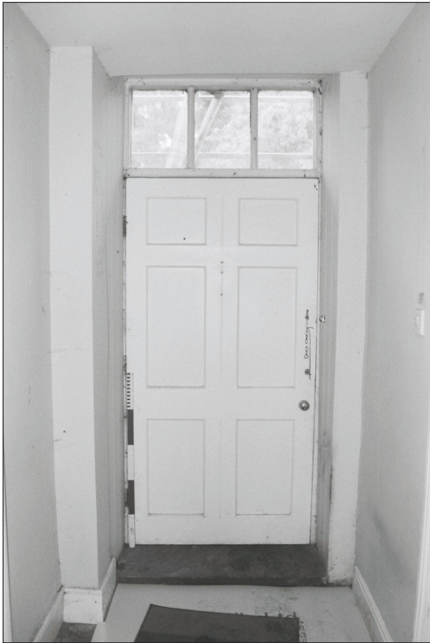
Plate 489: Detail of east entrance with timber panelled door and overlight, G48, South Range - Agent's House (Film 65.20)
