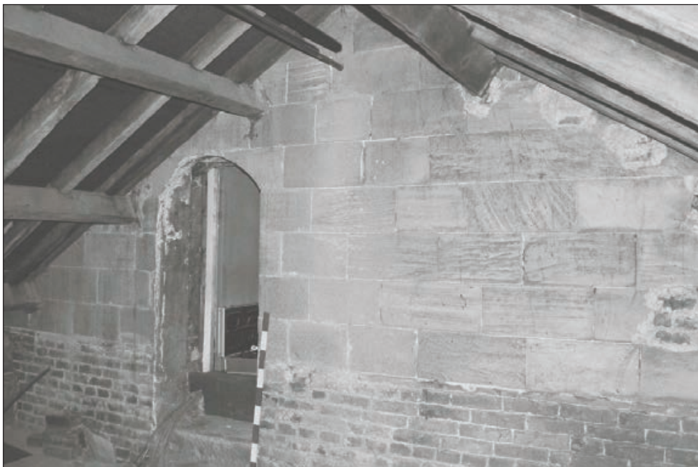
Plate 328: View of south gable wall of Roof Void 8, West Range - OB. 98 (Film 71.15)
