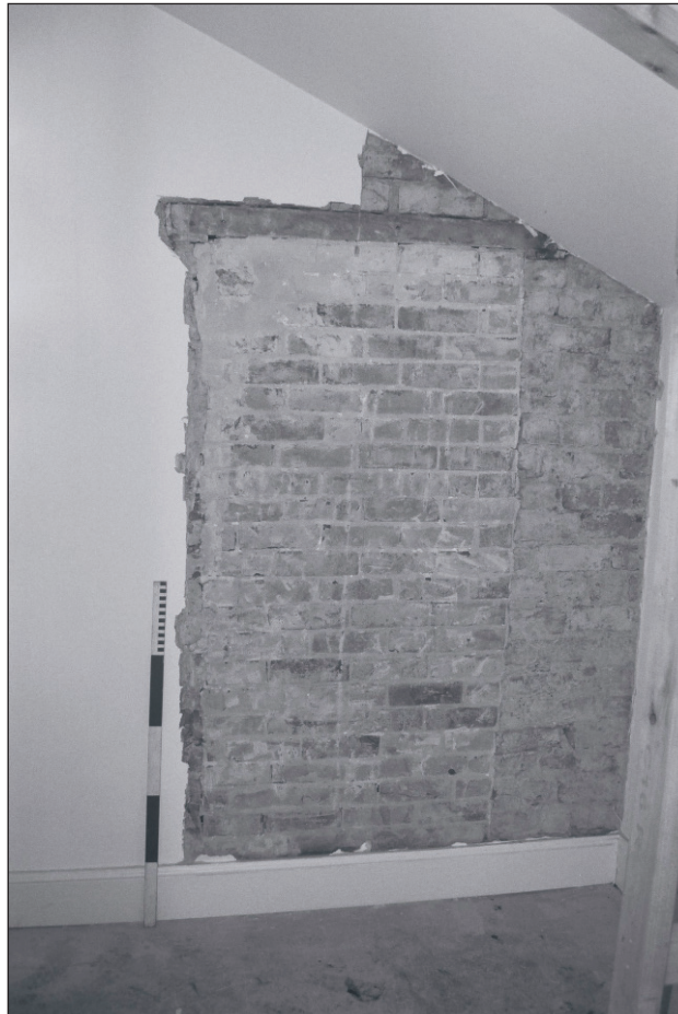
Plate 595: View of exposed blocked door within south wall of F43, East Range - OB. 06 (Film 46.02)
