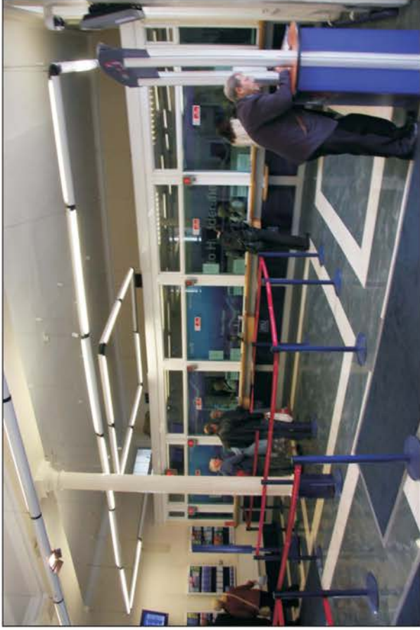
Plate 15: General view of booking hall in the Central Block, noting cast iron column and corniced ceiling.
