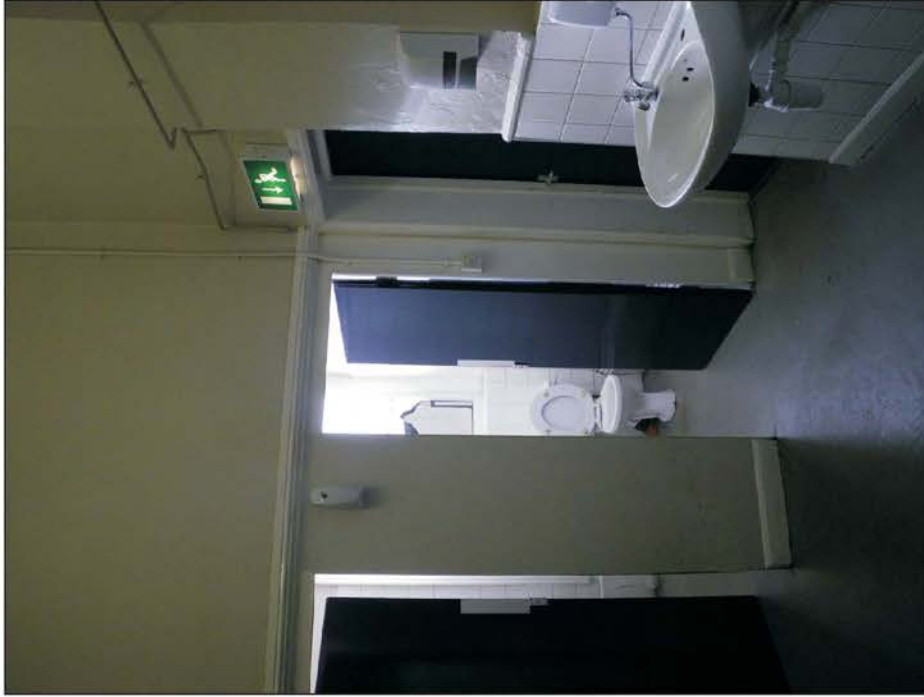
Plate 59: General view of toilets in South Wing, noting 1930s moulding, looking east.
