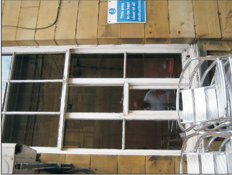
Plate 65: Detail of hatch in window to southwest corner of south pavilion, looking north.
