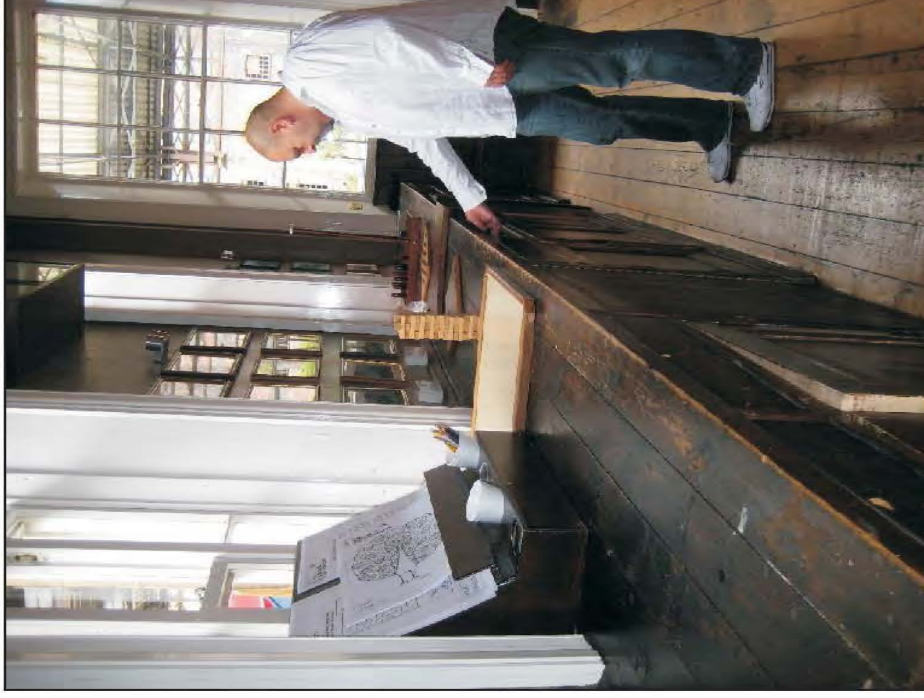
Plate 64: General view of counter in southwest corner of south pavilion, looking west.
