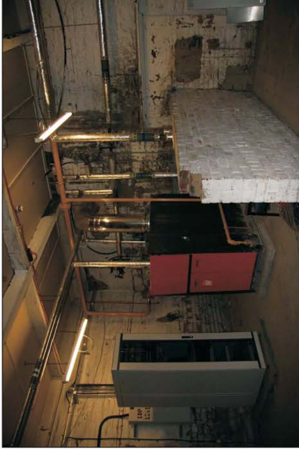
Plate 12: General view of boiler room in basement, noting blocked fireplace, looking north.
