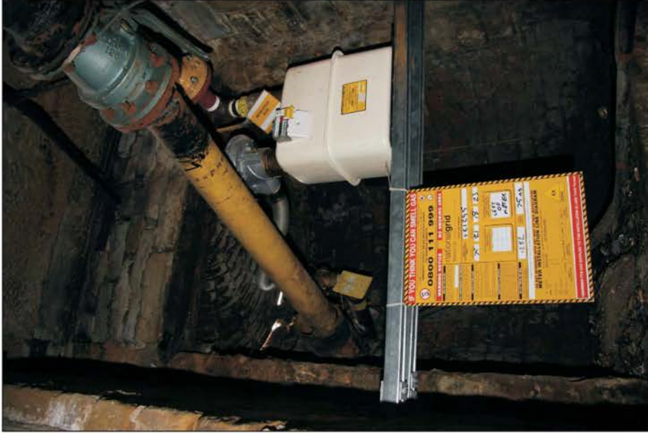
Plate 13: General view of former coal chute/light well in eastern wall of the basement.
