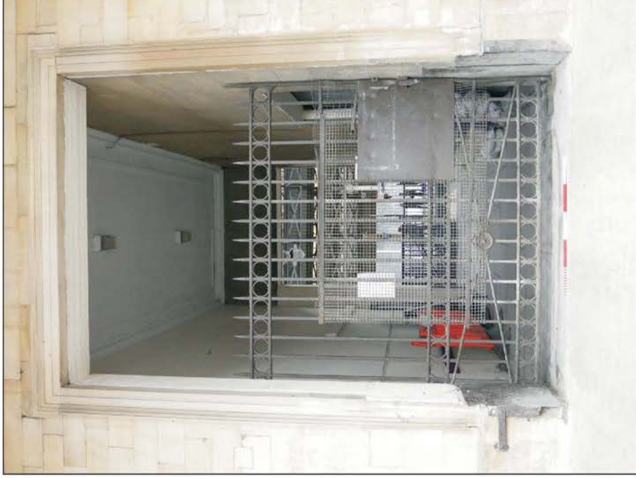
Plate 30: Detail of inserted through passage in the North Wing, noting iron gate and plaster ceiling within, looking west.
