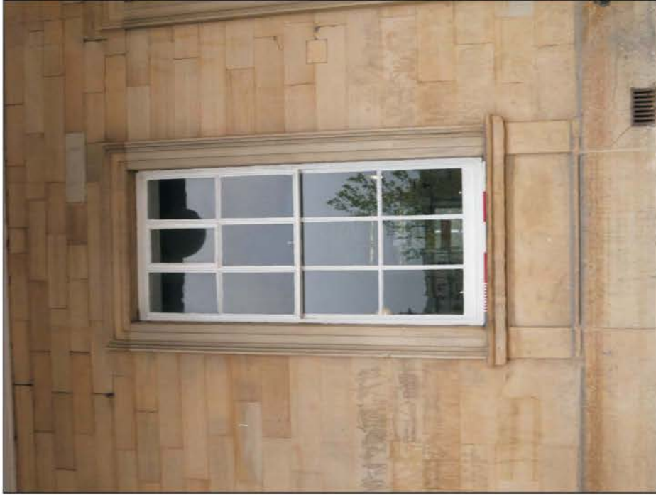
Plate 29: Detail of former doorway converted to a window in the east elevation of the northern pavilion.
