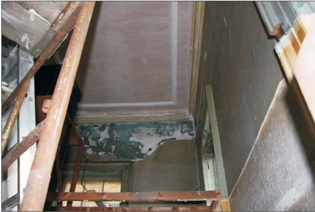
Plate 47: Detail of plastered ceiling in former managers office in the northern pavilion, looking north.
