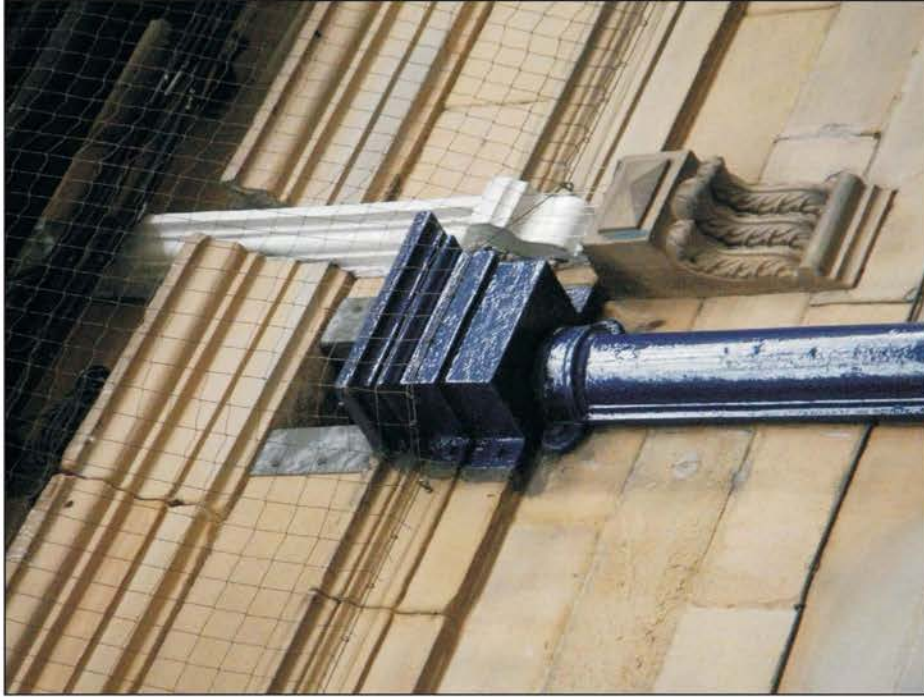
Plate 11: Detail of cornice , matching down pipe hopper and wall post on west elevation.
