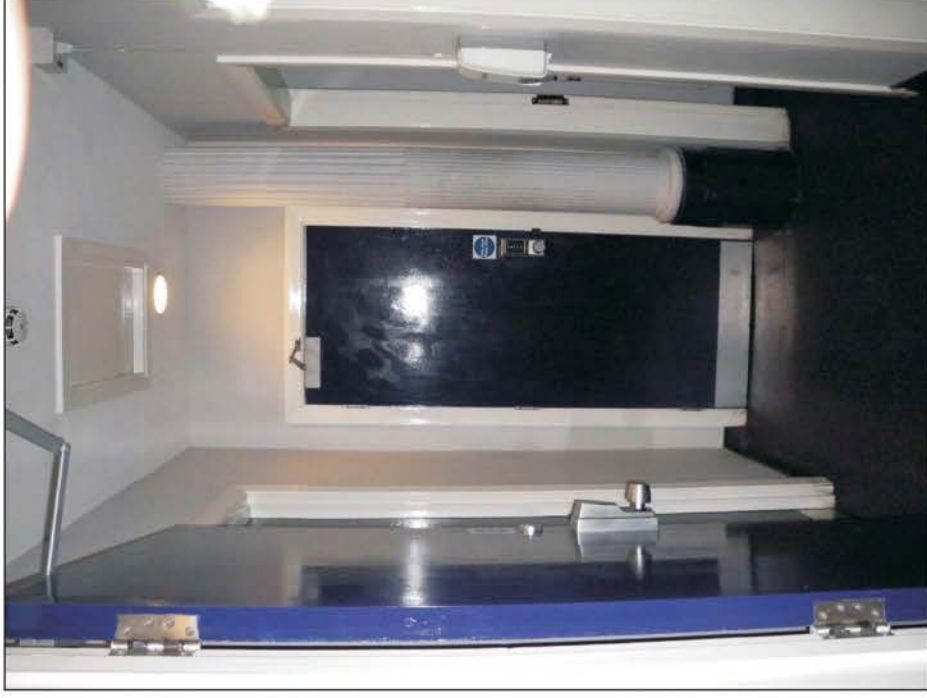
Plate 22: General view of admin area in south end of Central Block, noting cast iron column, looking north.
