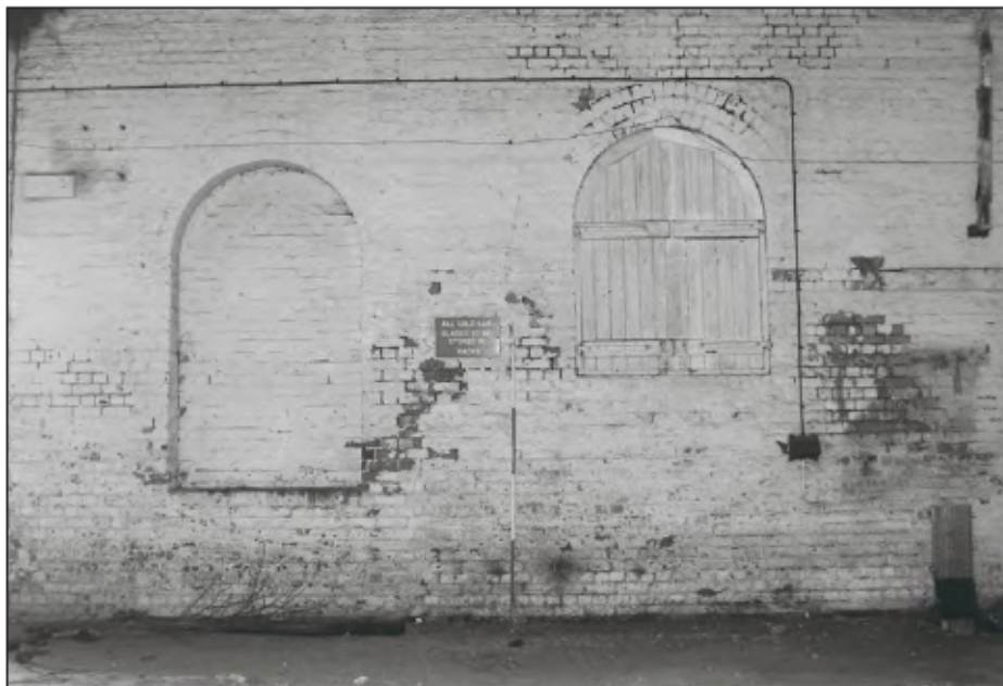
Plate 30: Detail of blocked arched windows in west elevation of Building 11, one retaining timber shutters. (film 12.28)
