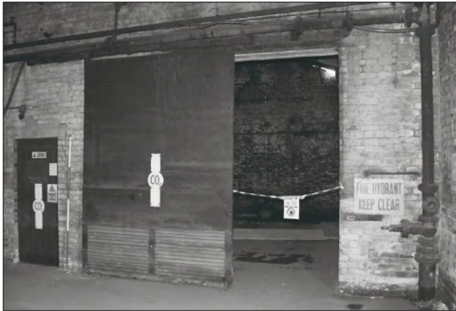
Plate 27: General view of Co2 storage room, Building 10. (film 27.14)
