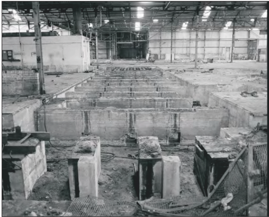
Plate 55: General view looking west over the foundations for the 18" Rolling Mill's cooling bed. (film 21.10)
