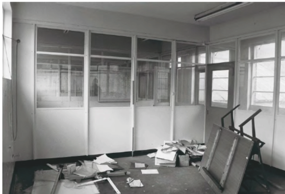
Plate 74: General view of the first floor interior of Building 14, looking south. (film 7.20)
