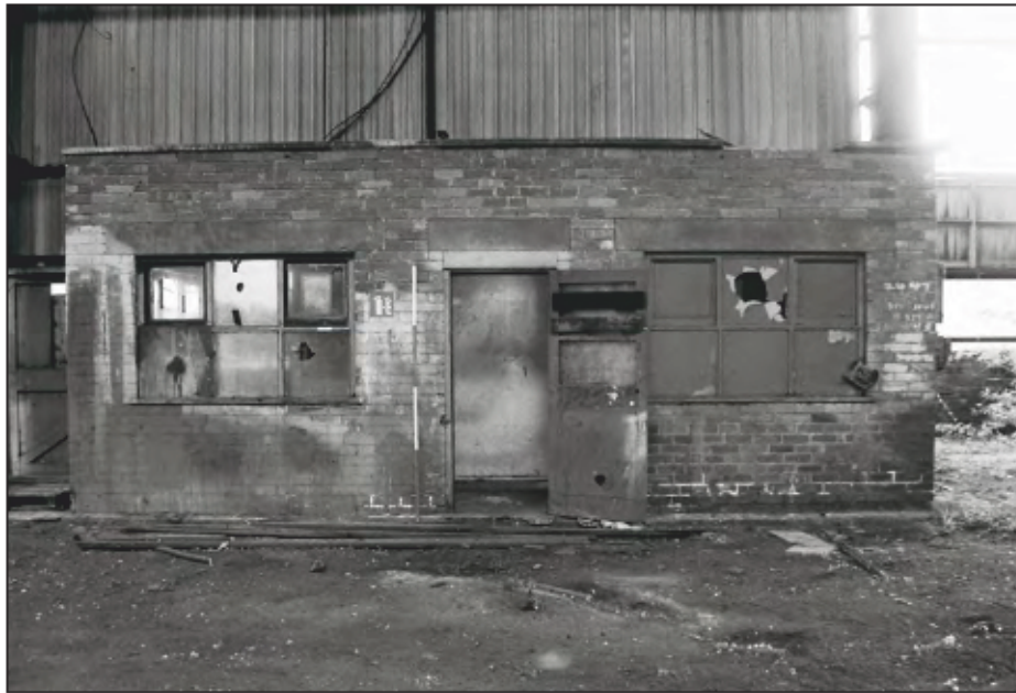
Plate 85: General view of office in centre of north wall of Building 18. (film 5.14)
