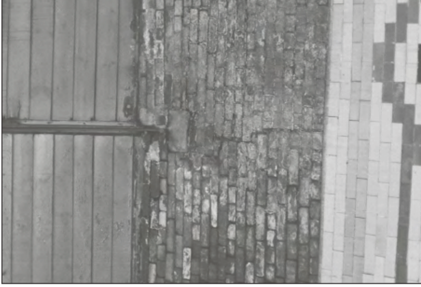
Plate 24: Detail of straight joint between original 1908 structure and 1915 extension. (film 26.29)
