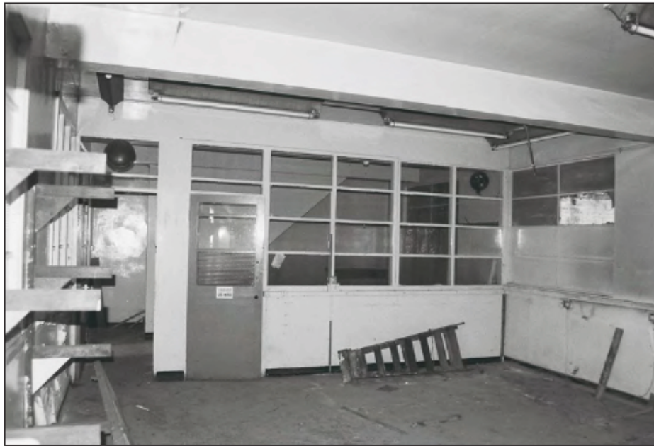
Plate 73: General view of the ground floor interior of Building 14, looking south. (film 7.22)
