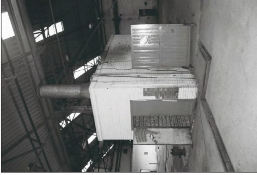
Plate 64: General view of the air filter house in the south of Building 11. (film 12.22)
