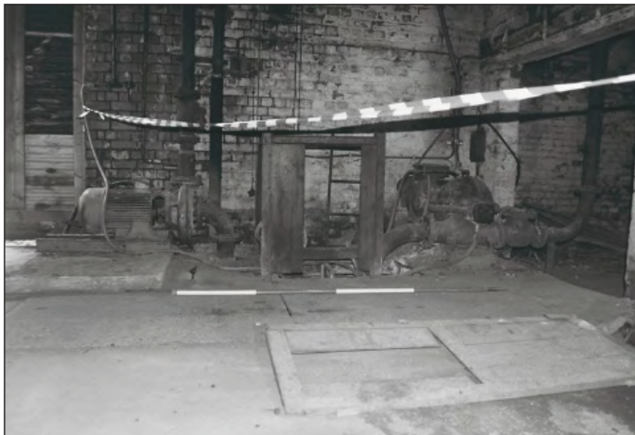
Plate 26: General view of pumps and well in lean-to extension to Building 10. (film 14)
