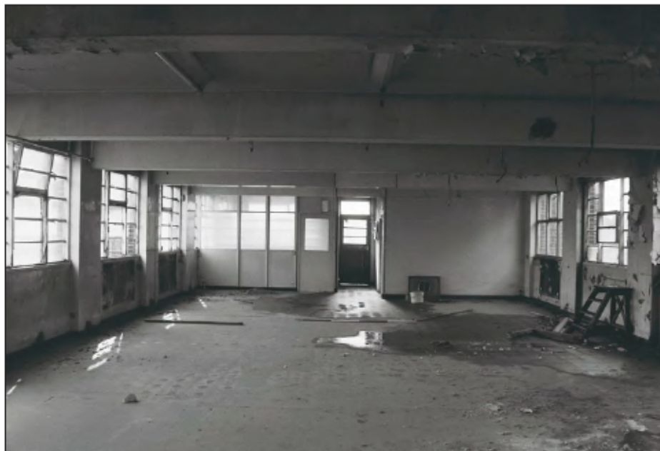
Plate 76: General view of the first floor interior of Building 15, looking east. (film 6.15)
