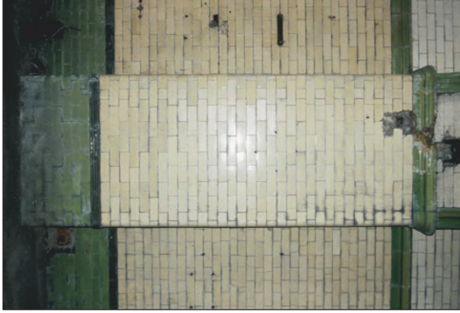
Plate 16: Detail of glazed tiles across original 1908 structure (right of pier) and 1915 extension (left of pier). (colour slide 4)
