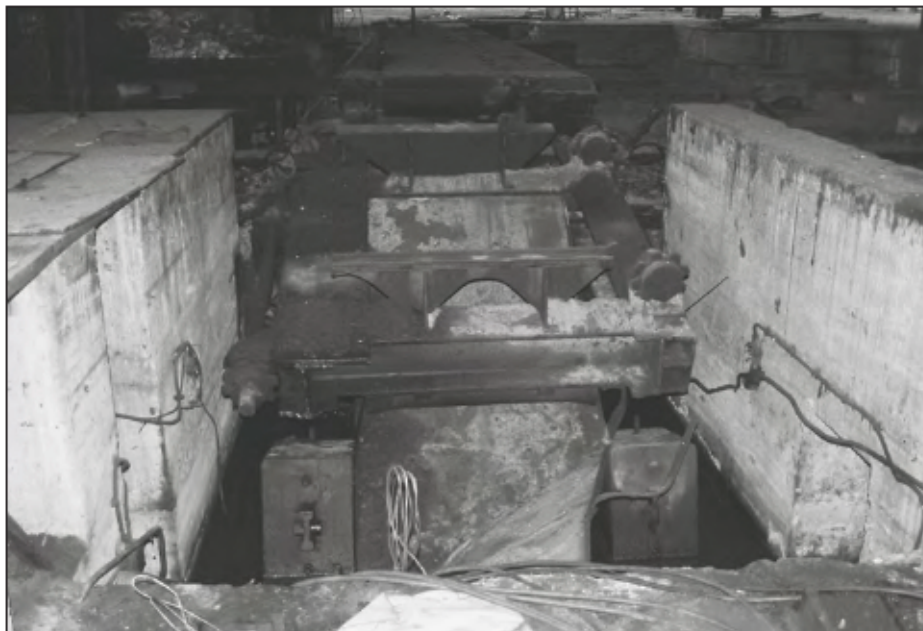
Plate 52: Detail of the remaining sub-structure of a tilt-table relating to the first intermediary stand of the 18" Rolling Mill. (film 11.11)
