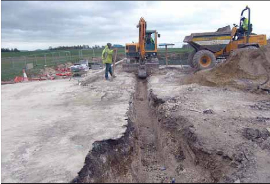
Plate 25: Monitoring of service trench in the old car park viewed from the south-west
