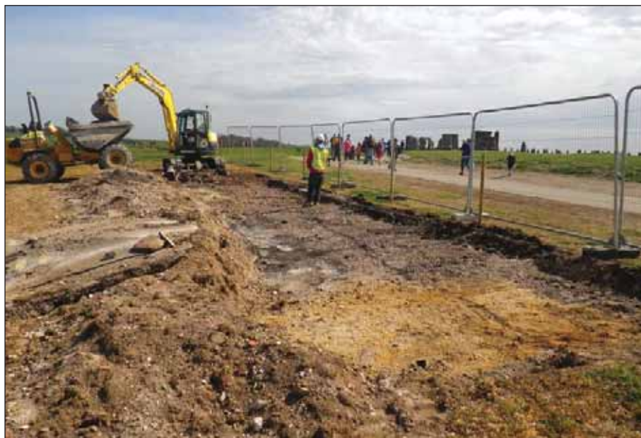
Plate 30: Removal of tarmac surface from north side of B344 during decommissioning works on former car park, viewed from northwest.
