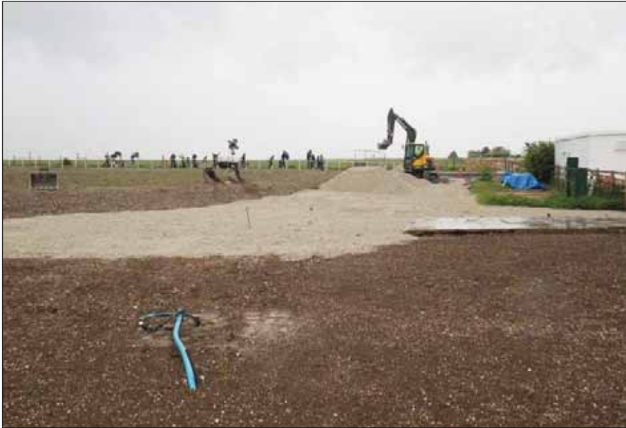
Plate 27: Re-instatement work in former visitors centre car park, viewed from the north.
