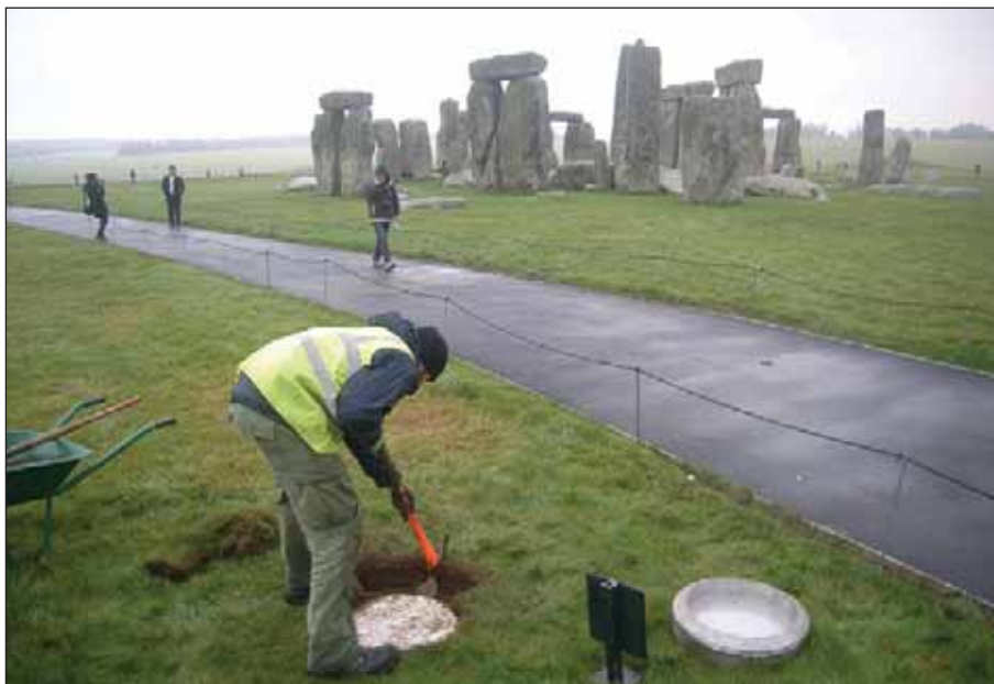
Plate 54: Removal of concrete marker for Aubrey Hole 32, and replacement setting for stone marker
