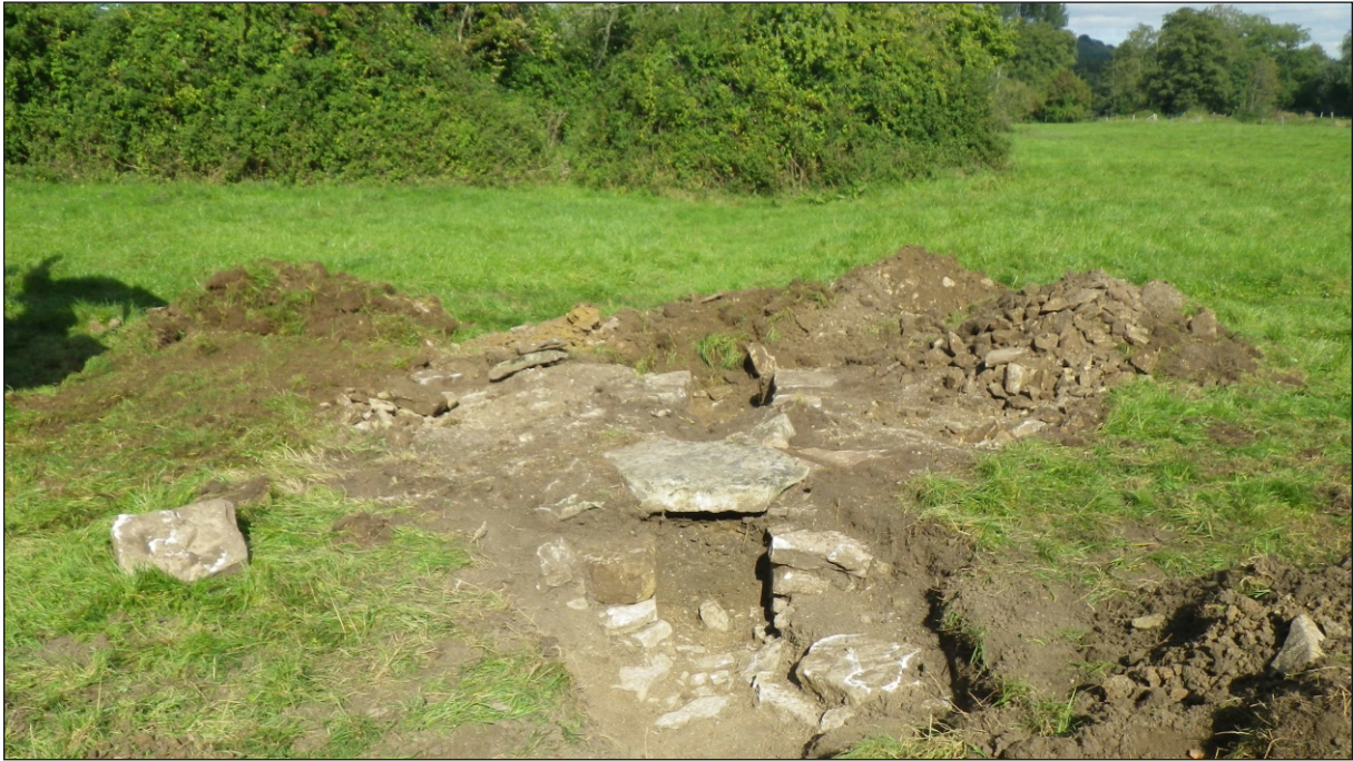
Plate 5: Wide angle view from south showing culvert in relation to silted up drainage ditch. Scale 1m
