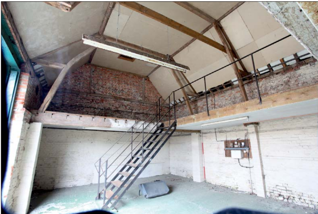
Plate 13: North end interior of Manor Barn showing sling braces and reset first floor
