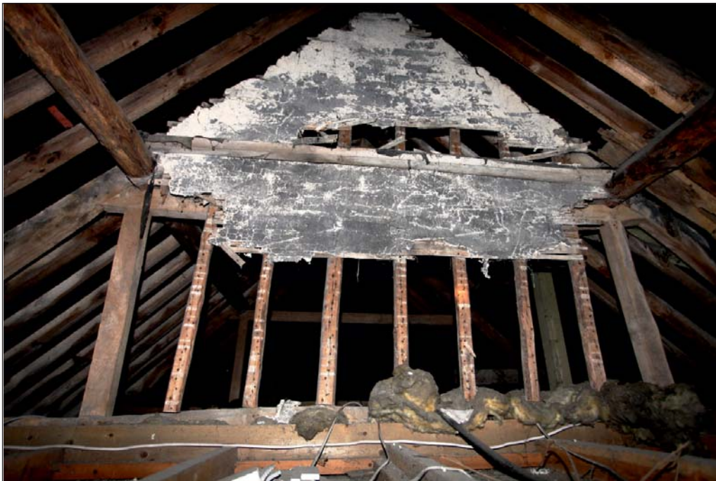
Plate 9: South end of Coach House roof space showing lath and plaster partition
