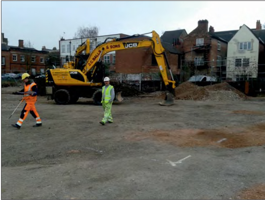
Plate 1: Site at start of works, looking south-east to rear of St. Mary's Gate
