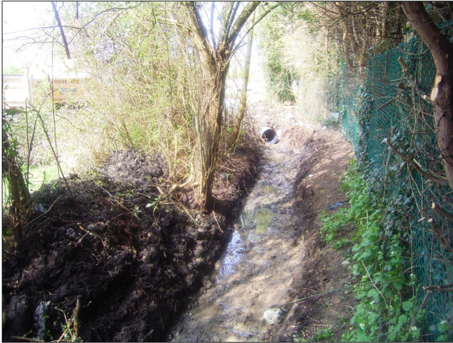
Plate 1: Section of drainage ditch south of Gas Lane taken from the east
