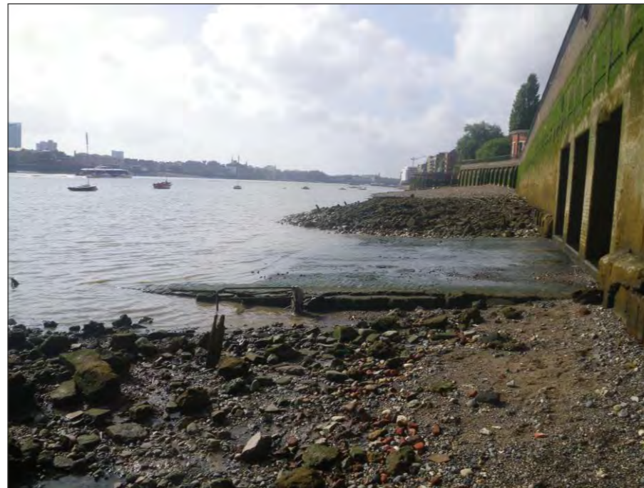
Plate 6: View from east of North Eastern Storm Relief sewer outlet and cobbled surface (HER ref 1P)
