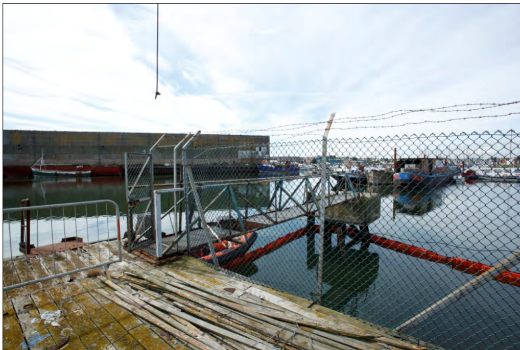
Plate 20: Deck of jetty, south-east end, showing south-west mooring dolphin and steel walkway, looking south-west
