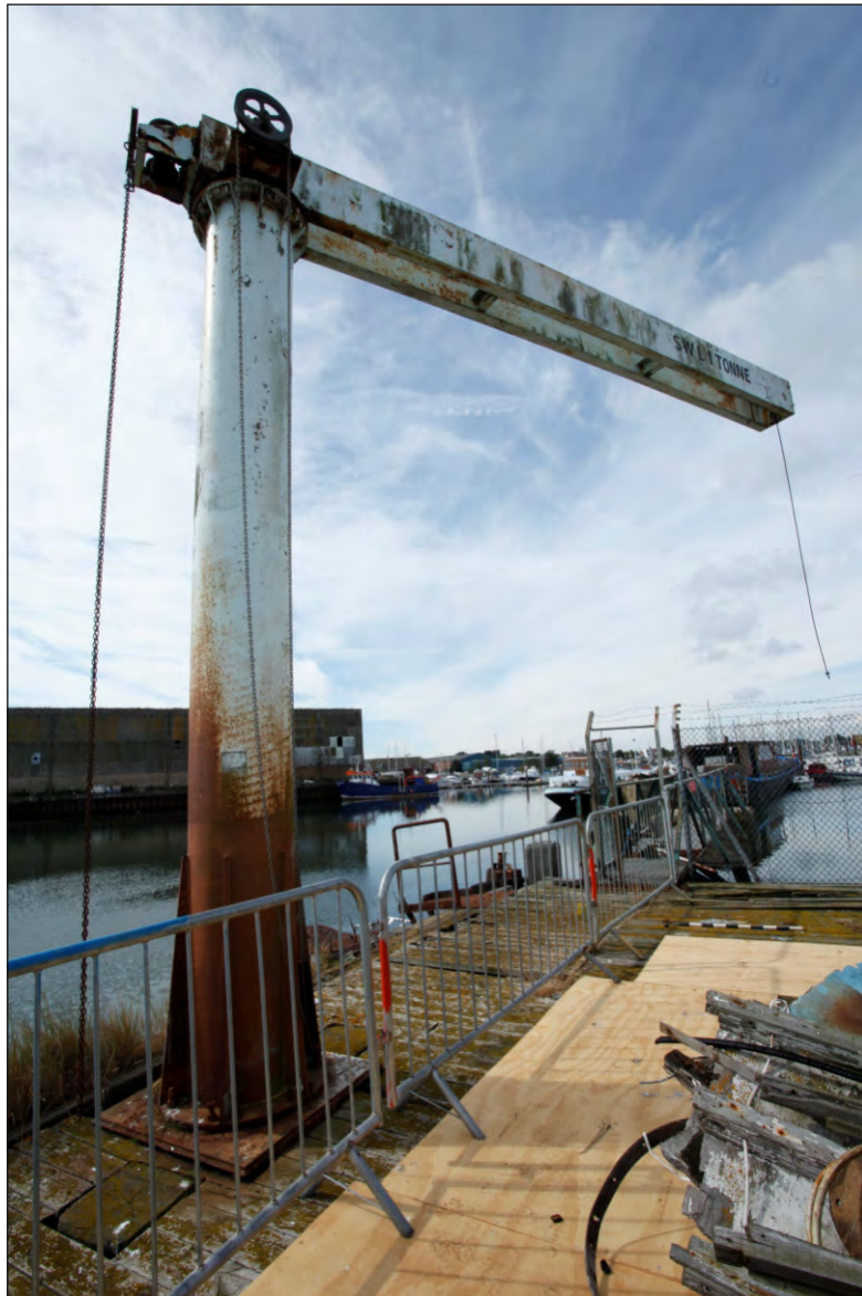
Plate 21: Detail of swing-jib crane on the south-east end of the jetty, looking south
