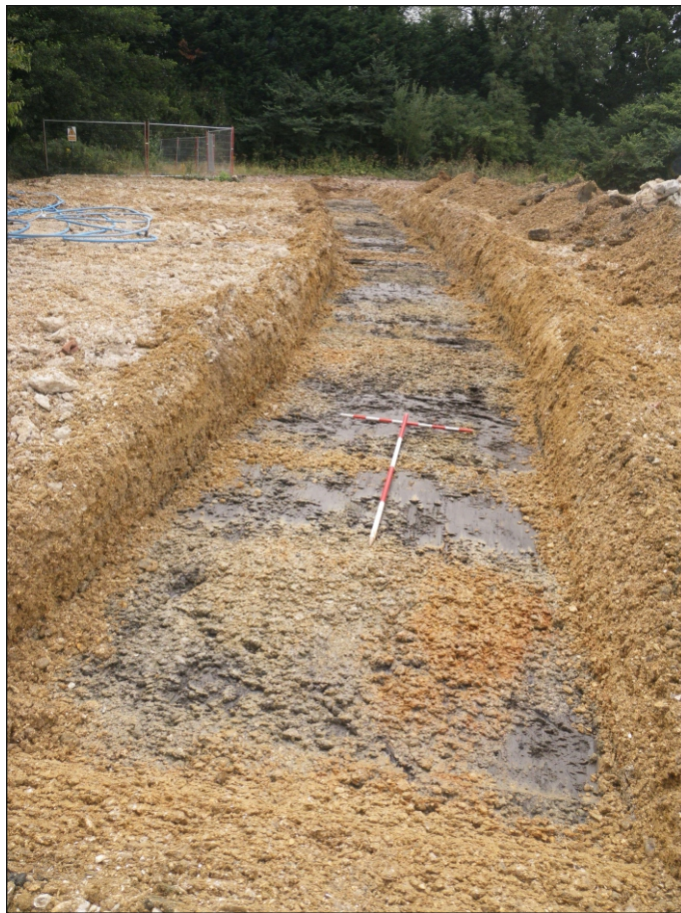
Plate 2: Trench 3 demonstrating the made ground and patches of contamination in the southern part of the Site
