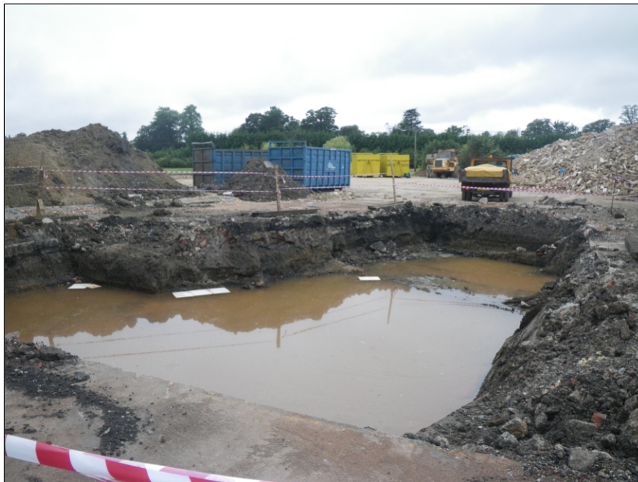
Plate 3: Area opened by the contractors to allow for the removal of deep contamination
