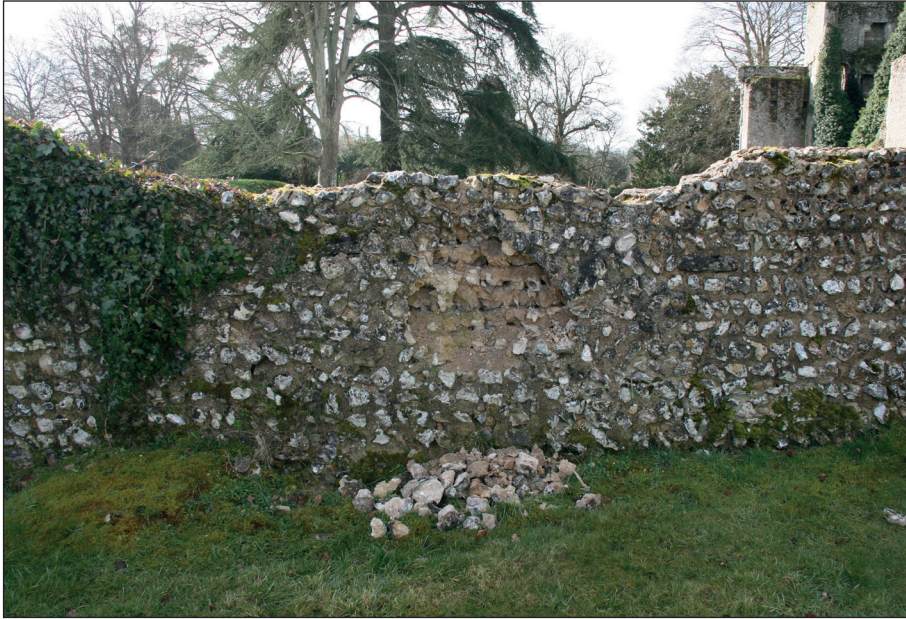
Plate 13: View from the north of the west end of the cross wall showing damage to stonework
