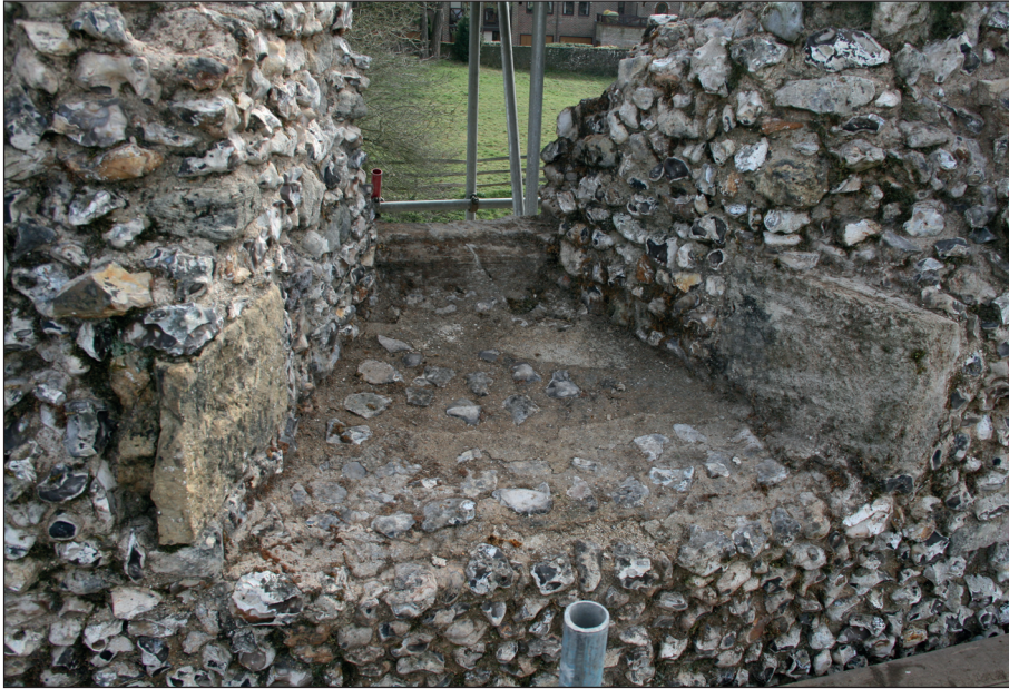
Plate 11: View from the west of a second floor window of the east wall, repointed across the base
