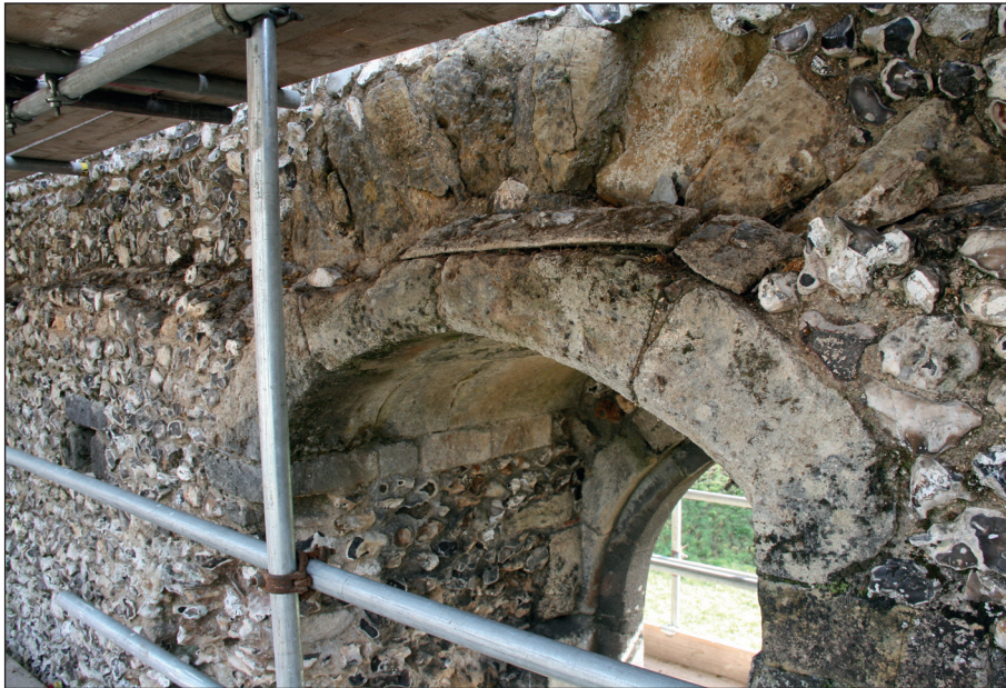
Plate 9: Northwest view of the east wall at the point above first floor where it narrows. The image shows the fragmented concrete that caps the ledge of the lower wall
