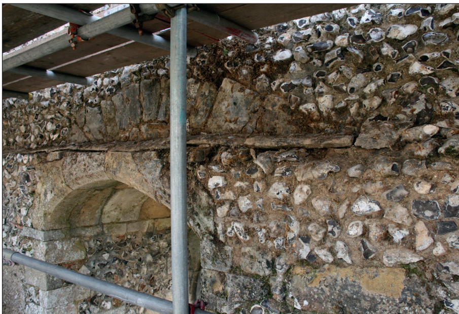
Plate 10: Northwest view of another part of the east wall at the point above first floor where it narrows. The image shows more fragments of the concrete capping prior to conservation.
