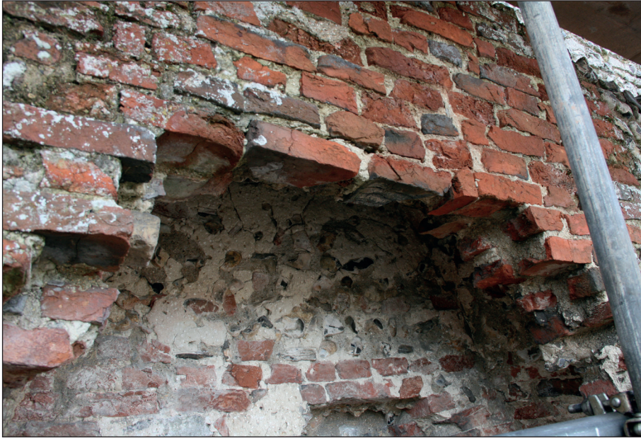
Plate 3: Amplified view of the brick fireplace including the chimney breast and flue
