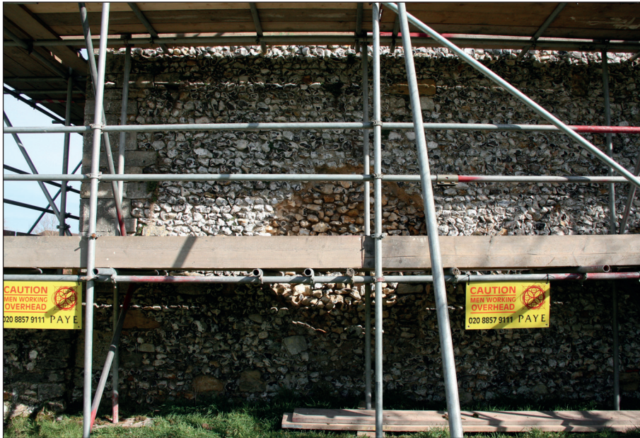
Plate 1: View of the southern elevation of the south wall prior to repair
