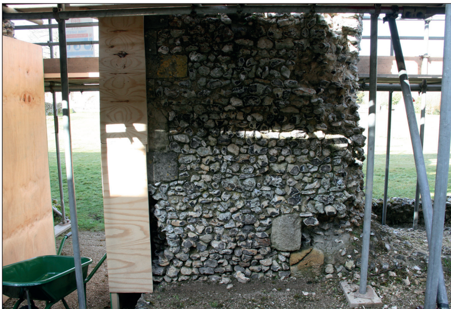
Plate 6: View from the north-east of the north side of a large breach in the centre of the west wall
