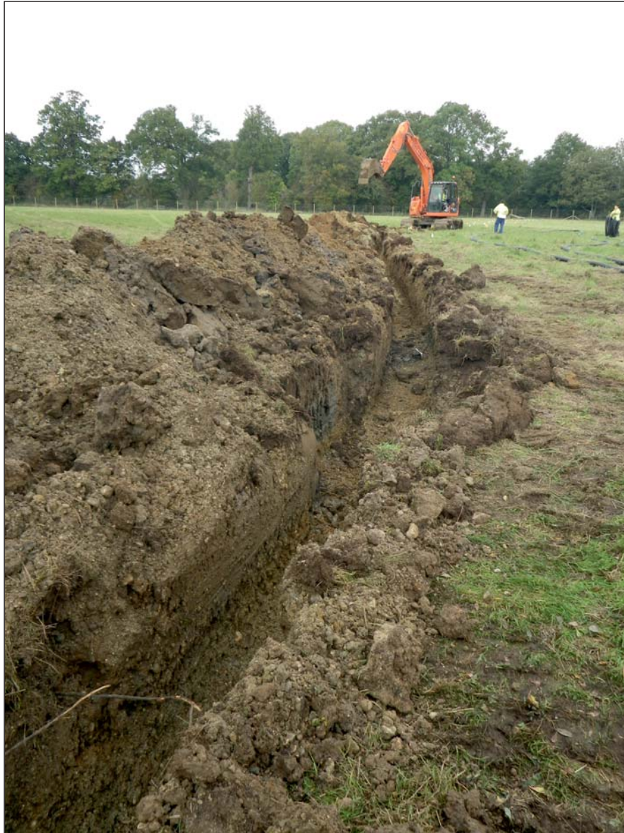
Plate 7: Main electrical cable trench from across northern field, viewed from the south
