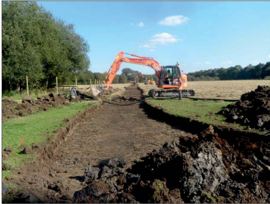
Plate 5: Main electrical cable trench within priority zone, viewed from the east
