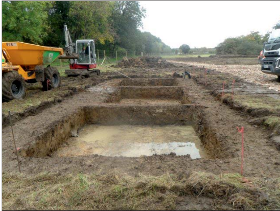
Plate 8: Foundation trenches for communications building and inverter cabin, viewed from the east
