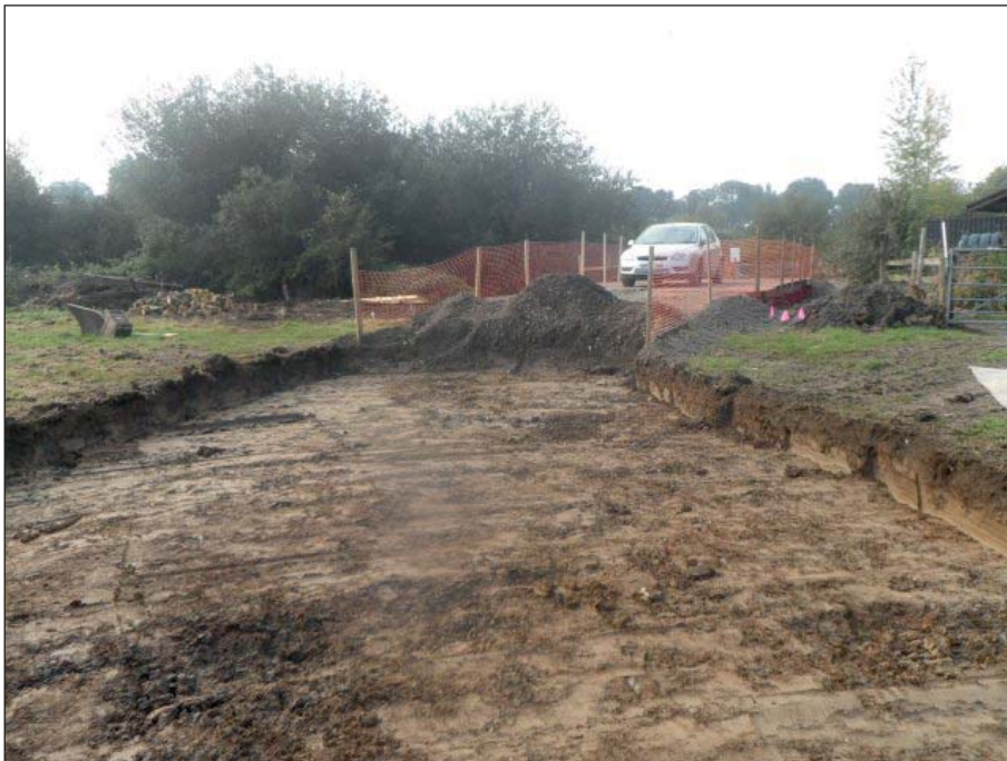
Plate 2: Strip for access road adjacent to new bridge, viewed from the north
