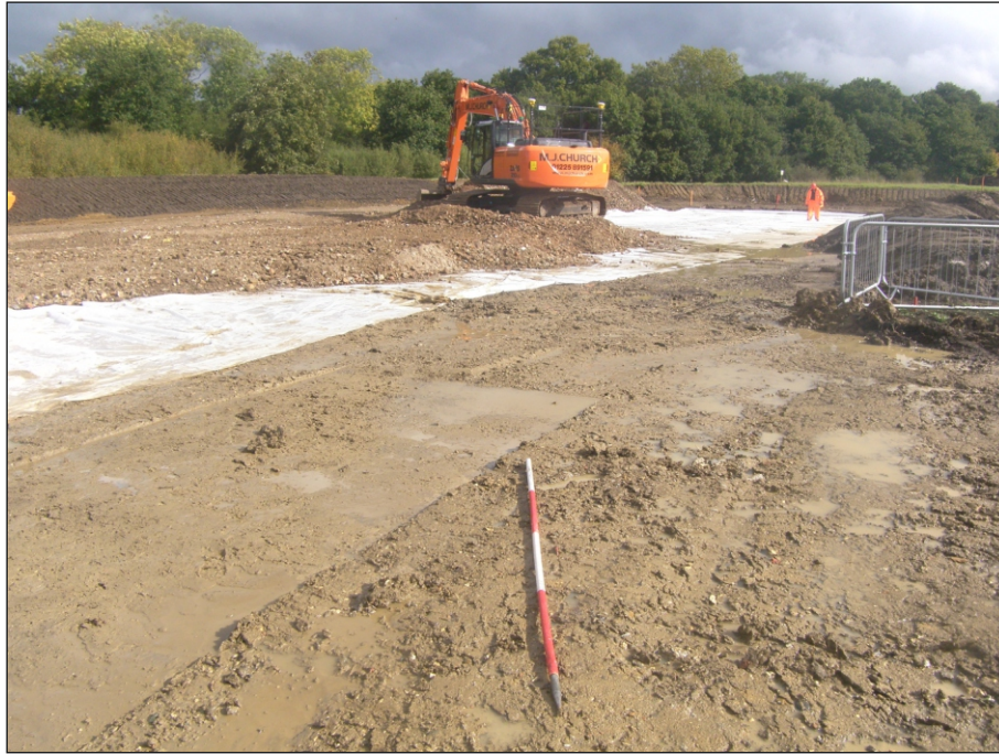
Plate 1: The north end of Site viewed from the southwest. The image shows the striped area being covered with terram and a layer of stone rubble. Context 1003 is visible in the foreground.
