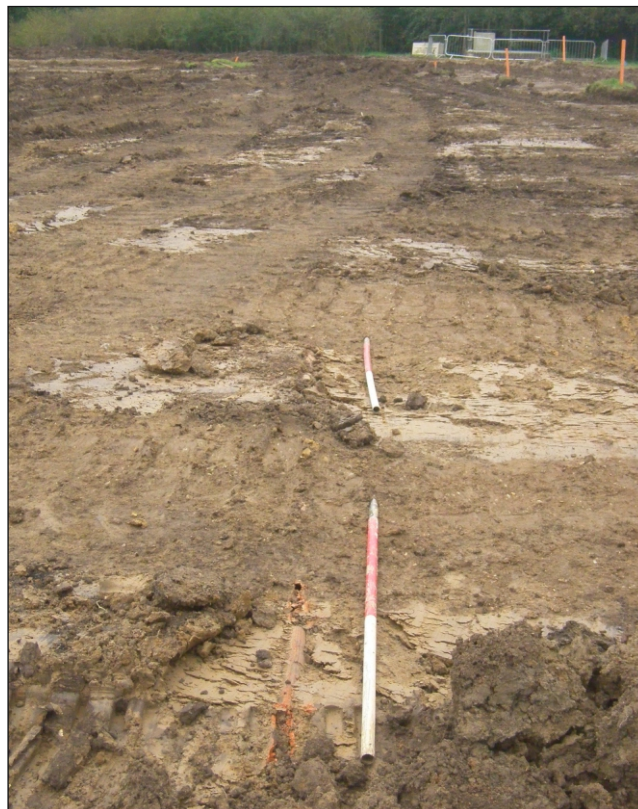
Plate 6: Ceramic drainpipe 1015 that forms part of a field drain network across the Site. View from the northwest.
