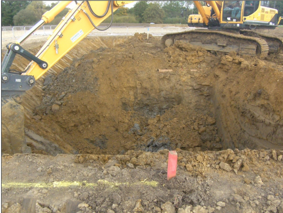
Plate 7: Ceramic drainpipe 1017 in-situ during excavation of the Cake Import Hopper area. View from the south.
