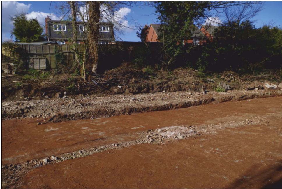
Plate 3: General view of Trench 1 from the south-east to illustrate the truncation of the Site
