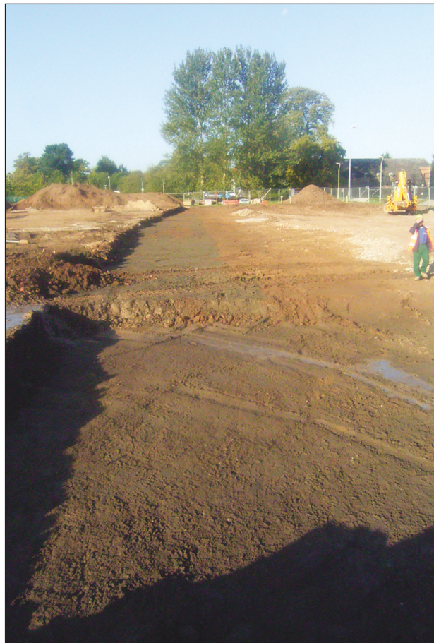
Plate 2: Dark silty clay within palaeochannel, found in last machine stripped area of the Site
