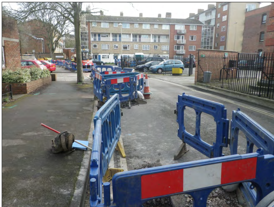
Plate 16: General view of Clare Street (Heritage Zone 5), camera facing south-east
