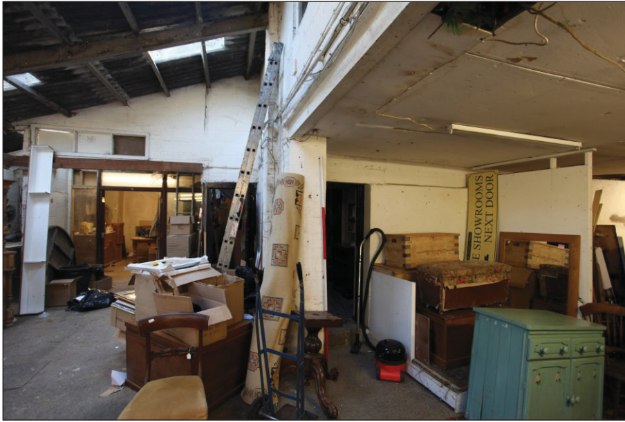
Plate 9: East-facing view showing the lean-to extension and the outer wall of the flat-roofed structure
