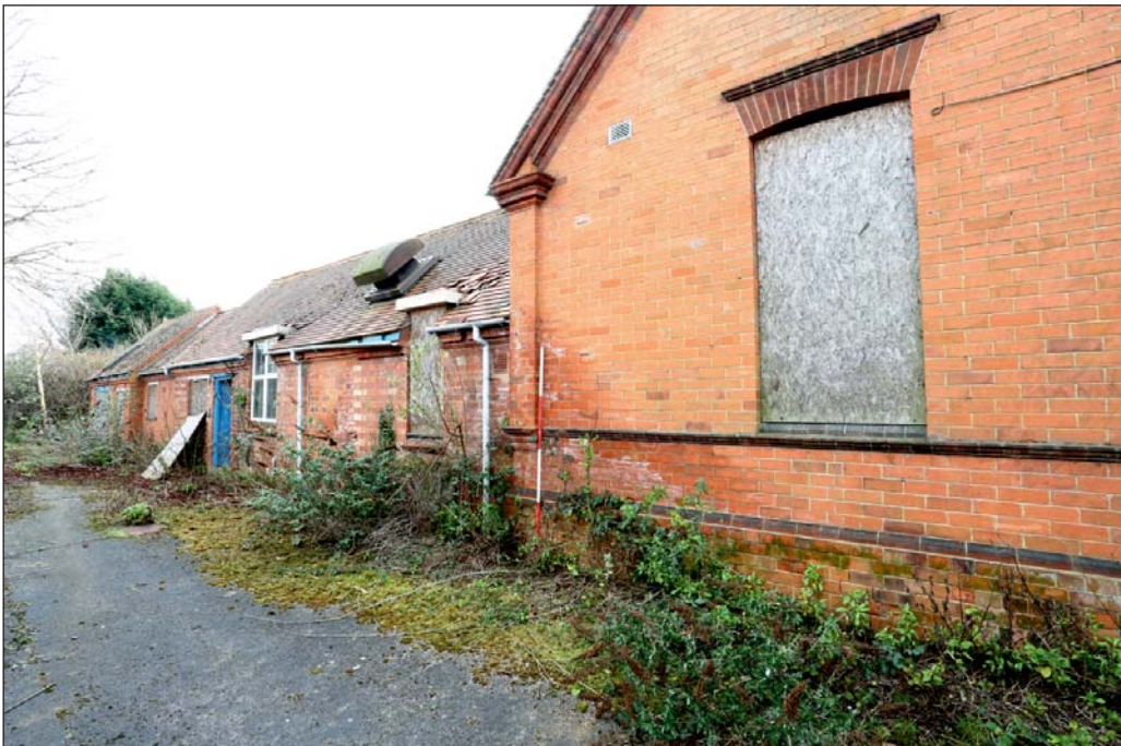
Plate 4: North side single storey wing also showing air vent in north projection wall
