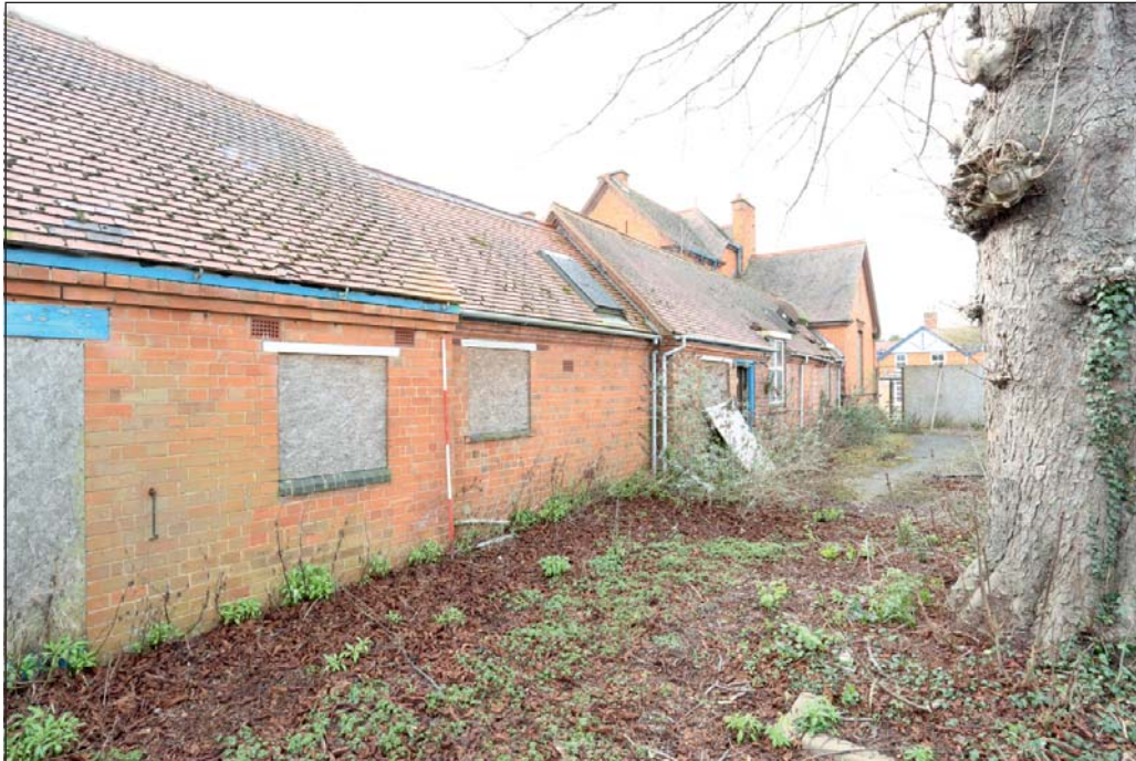
Plate 5: Showing original single storey kitchen to right of image and lower pre WW1 extension. Mortuary to left
