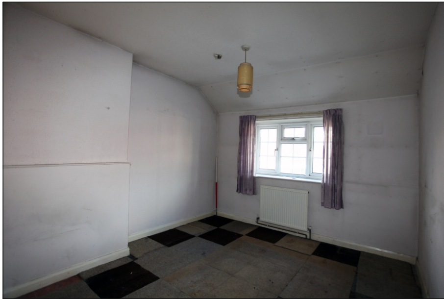
Plate 11: View from the east of bedroom 1 on the first floor of No. 13
