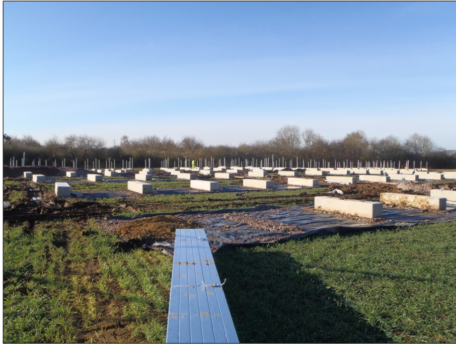
Plate 1: View of area of preservation in situ, with above-ground structure for solar array
