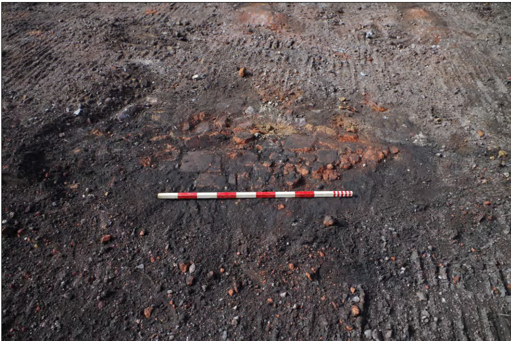
Plate 2: Damaged yard surface 107 from north
