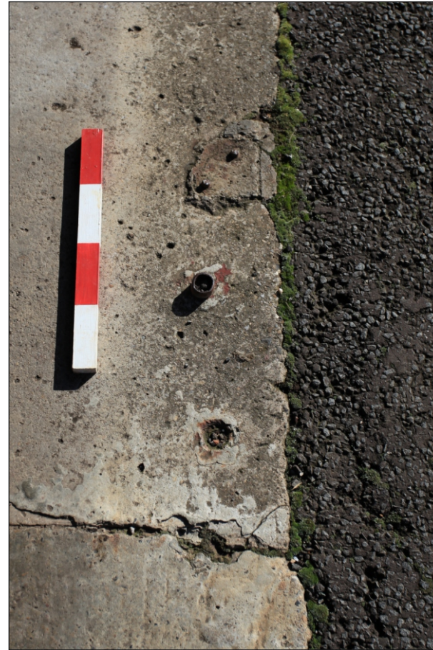
Plate 23: Detail of typical bolt keeps embedded within the threshold to the vehicular entrances of the tank garages (Romney sheds)
