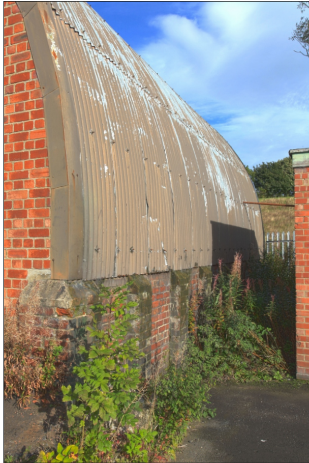
Plate 10: Oblique view of the east elevation of the tank garages (Romney sheds)
