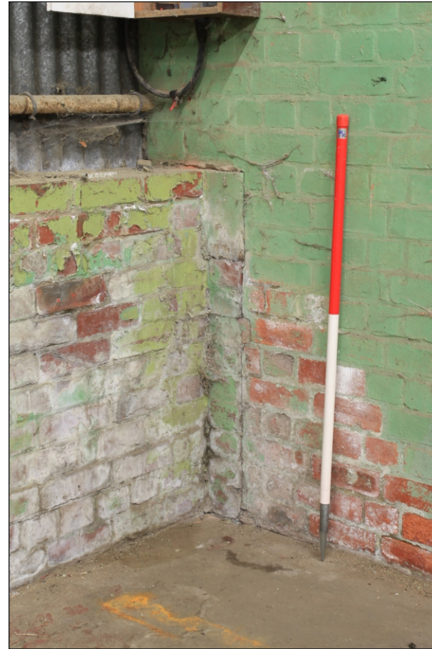
Plate 19: Detail of an embedded pier with the south-east corner of the tank garages (Romney sheds)
