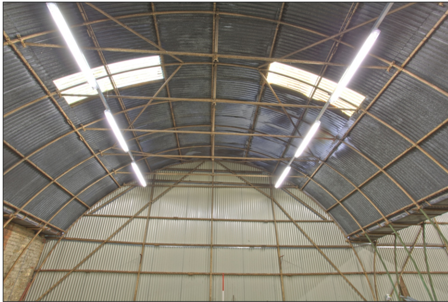
Plate 14: View within G2 showing a typical roof structure of the tank garages (Romney sheds)
