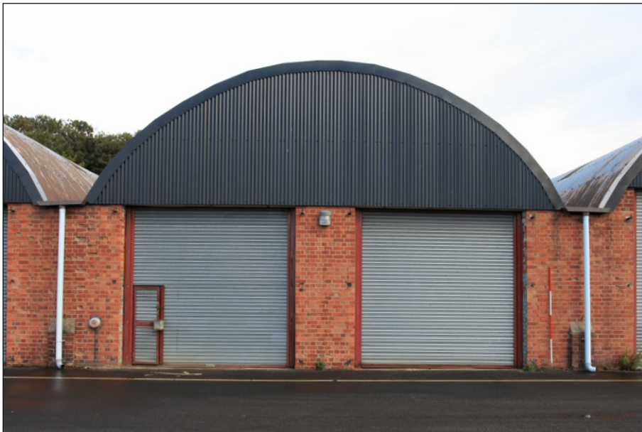
Plate 9: View of a typical bay of the south elevation of the tank garages (Romney sheds)
