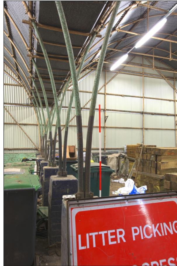
Plate 17: Detail of a typical row of piers and arch springs within the tank garages (Romney sheds)
