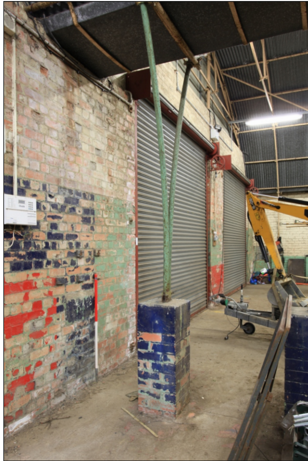
Plate 16: Detail of a typical pier showing the steel arches within the tank garages (Romney sheds)
