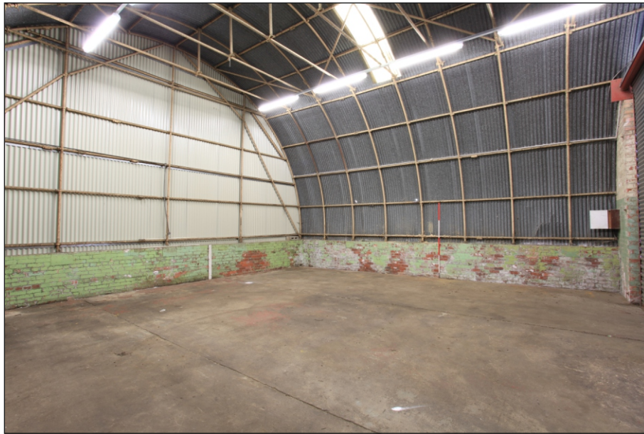
Plate 20: General view of G6 showing the joint of roof structure with the outer walls, looking north-east
