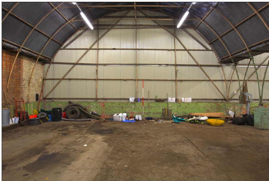
Plate 15: View within G2 showing a typical north wall and gable structure within the tank garages (Romney sheds)
