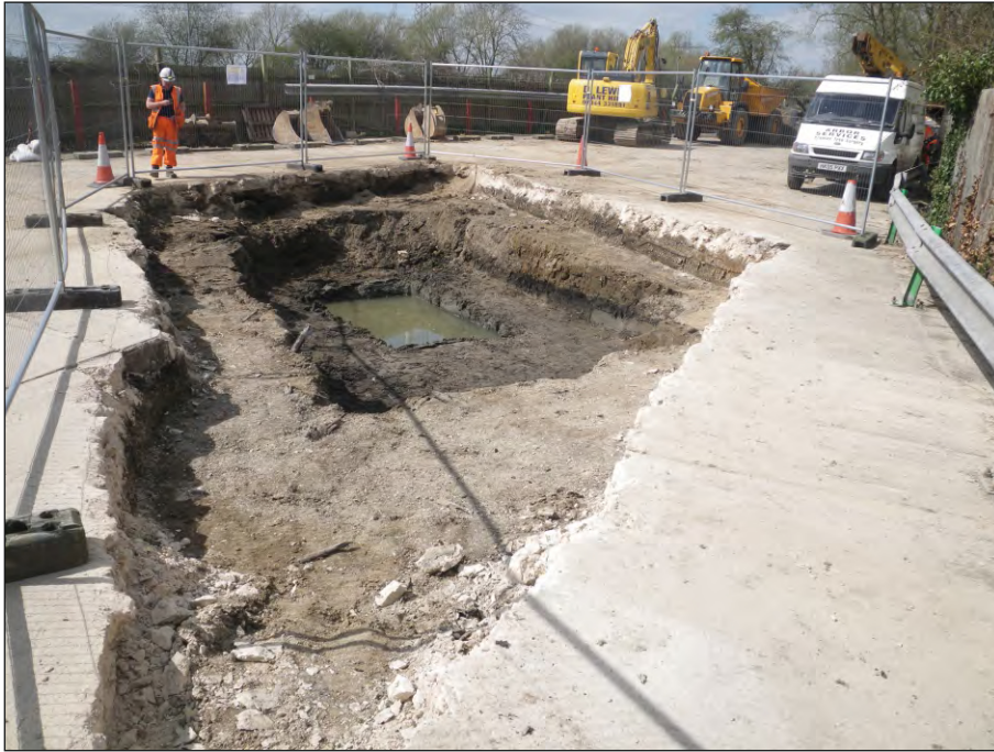
Plate 3: View from the south-east of completed excavated area with groundwater infilling central sondage
