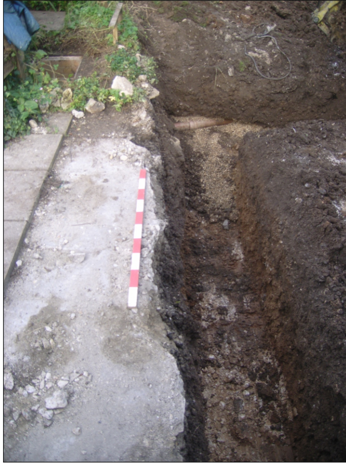
Plate 1: View to west along southernmost excavated foundation trench showing disturbed soils above a yellowish/reddish brown natural clay layer with underlying degraded chalk. A drainage pipe trench is also visible in far corner.
