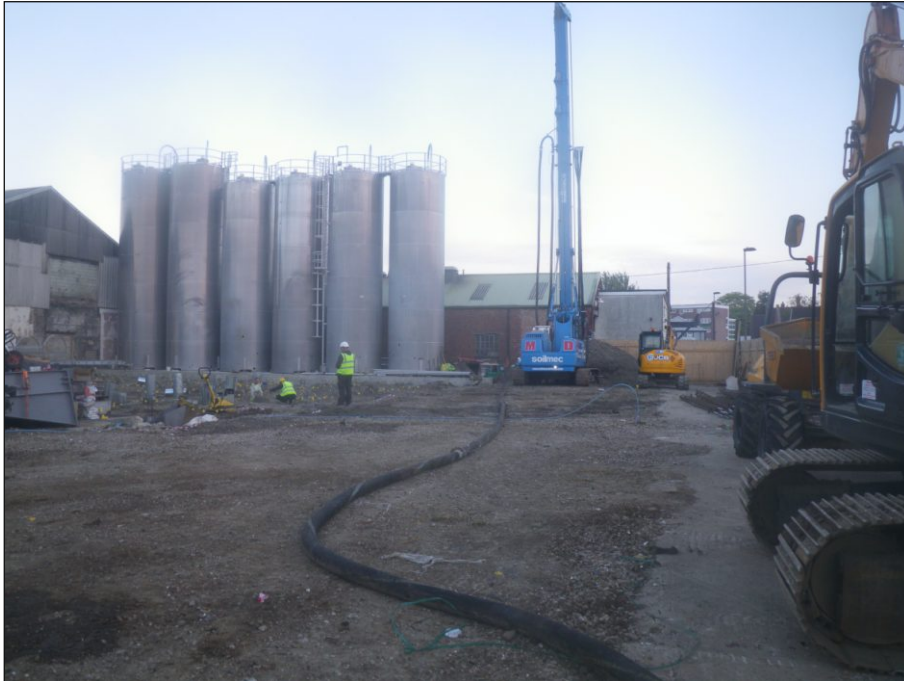
Plate 1: Site of proposed office building with silos to the left, looking north
