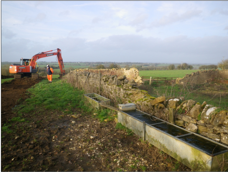
Plate 3: Site TC6, access road adjacent to ruined farm building, view from the north
