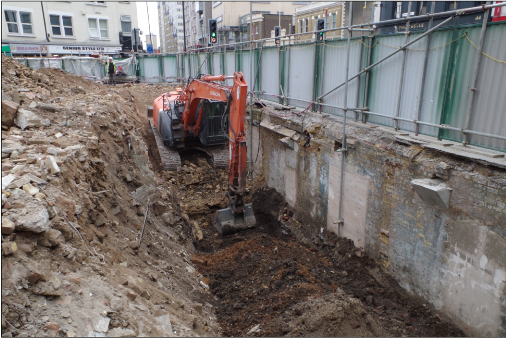
Plate 1: Working shot along the edge of Whitechurch Lane from the north east
