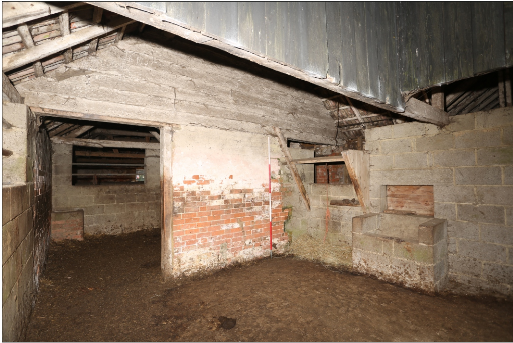
Plate 21: Building 6 south pen viewed from the north-east. The interconnected north pen of Building 7 is partially visible to the left
