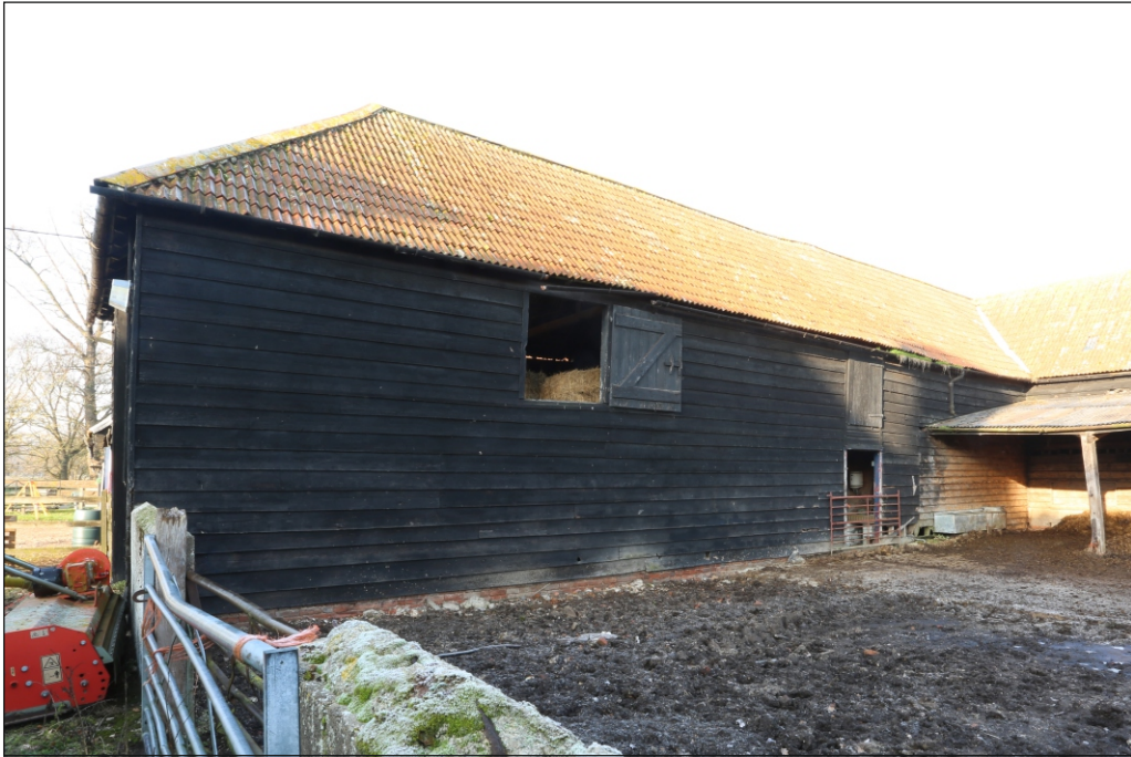
Plate 9: Redundant agricultural buildings viewed from the south-east, specifically the east side of Buildings 1 and 2 (left to right)
