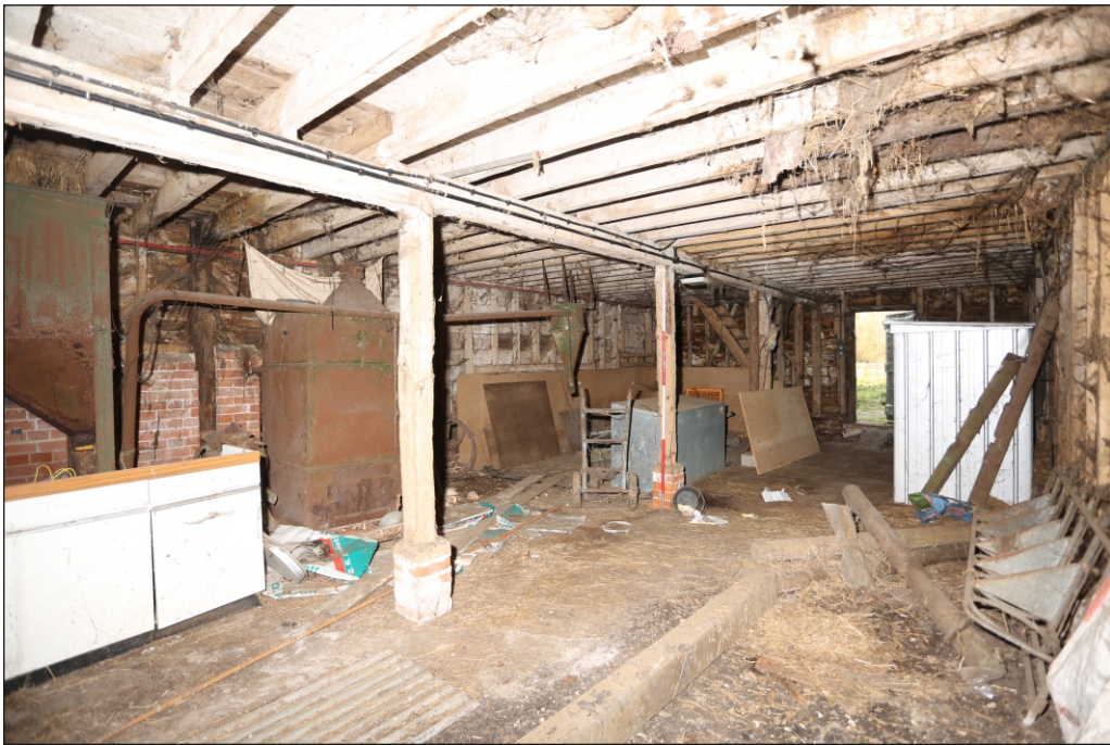
Plate 14: Building 3 ground floor viewed from the south-east. Note the staircase in the far corner and machinery to the left
