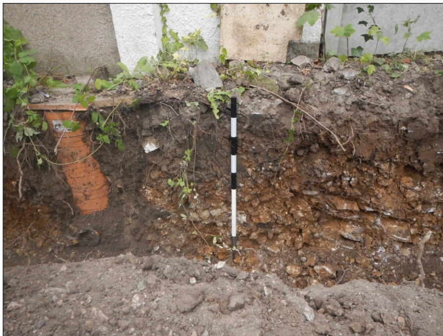
Plate 2: Limestone bedrock below subsoils in the northeast corner of the site, looking north-east, 1 m scale
