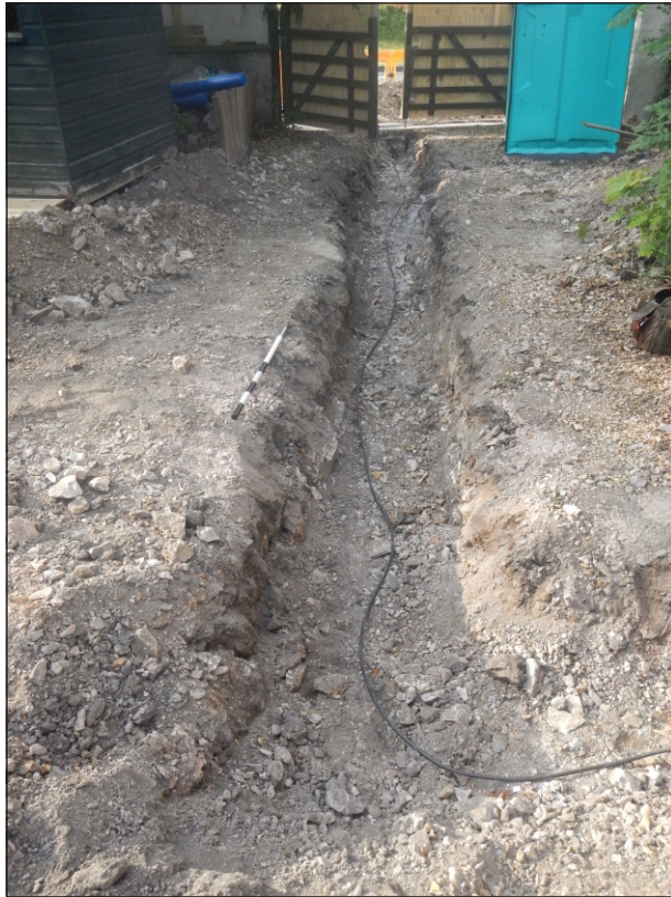
Plate 1: The service trench at the western side of site, looking south-west, 1 m scale
